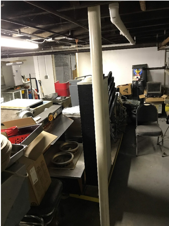
Photo 5: Looking west at northern pickup point and lateral piping to southern pickup point.
