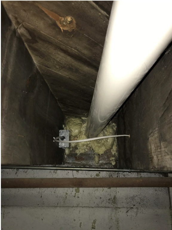
Photo 3: Looking north at ceiling from inside 5619 22 nd Avenue at electrical connection and pipe to fan.
