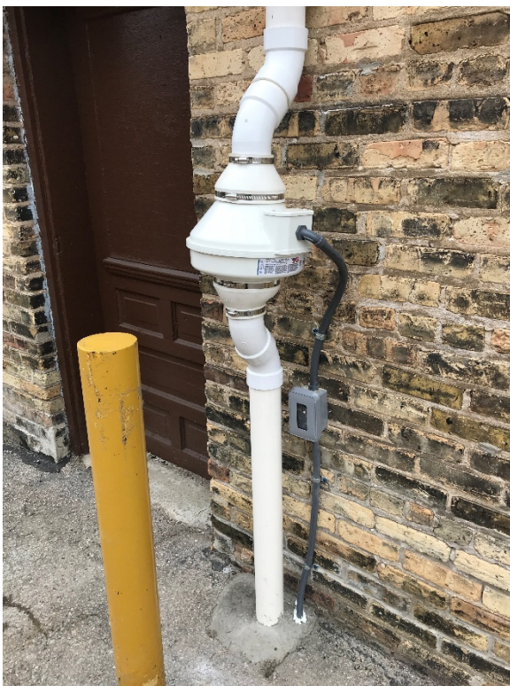
Photo 2: Looking at VMS fan and electrical connection.
