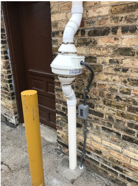
Photo 2: Looking at VMS fan and electrical connection. 11/21/18
