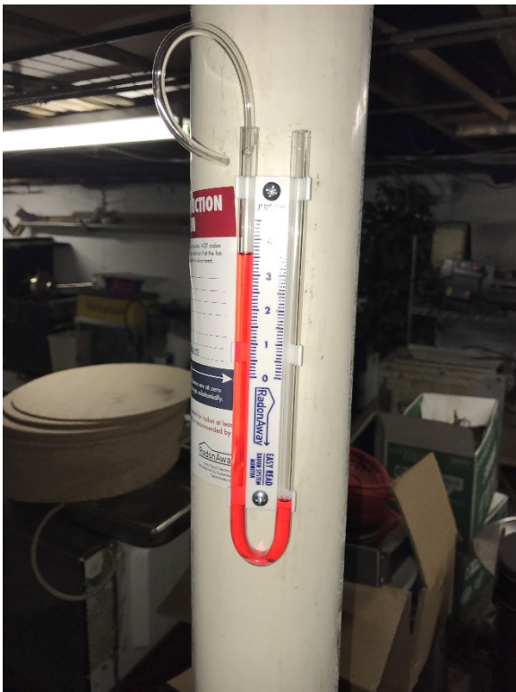
Photo 6: Manometer on northern pickup point. 11/21/18
