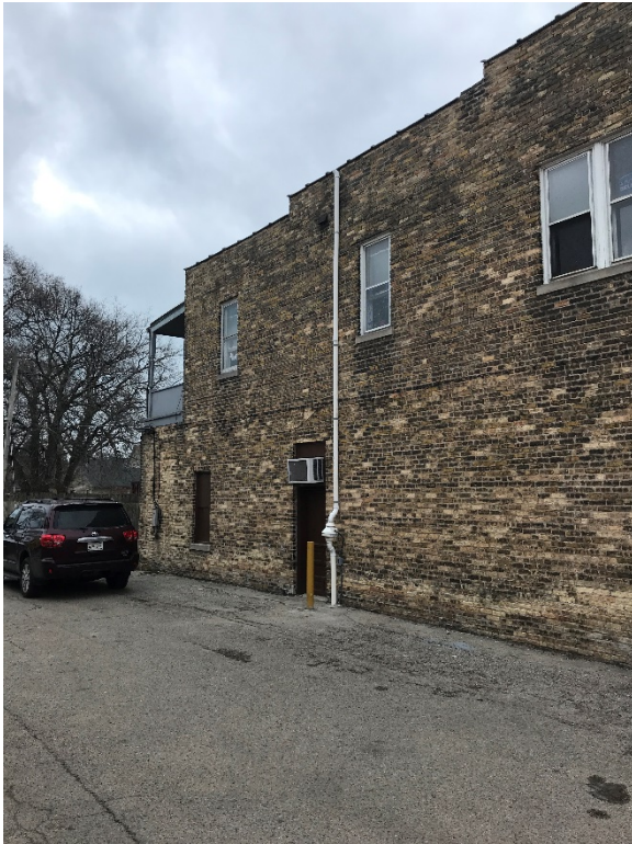
Photo 1: Looking southeast at vapor mitigation system (VMS) fan and exhaust line on north side of 5619 22 nd Avenue building (former Arctic Laundry & Cleaners). 11/21/18
