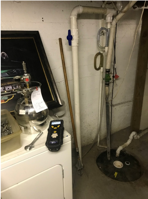
Photo 9: Looking northeast at southern pickup point (left side of photo) and sealed sump. 4/22/21
