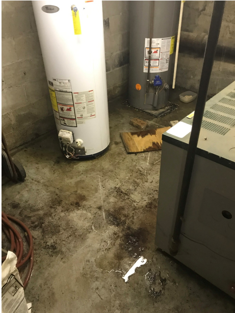
Photo 9: Looking at utility room near southeast corner of basement.
