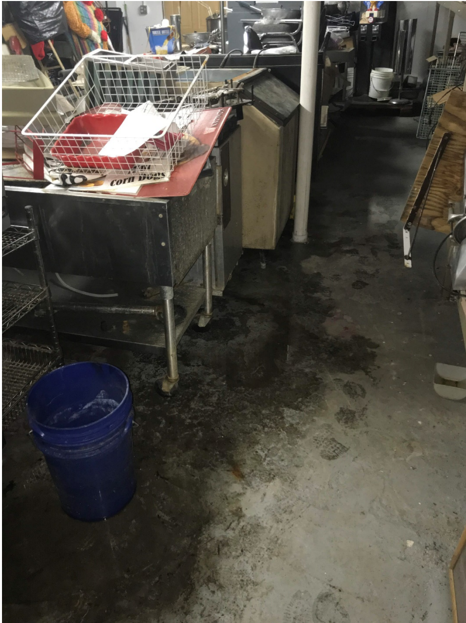
Photo 2: Looking west in basement at northern vapor mitigation system pickup point.
