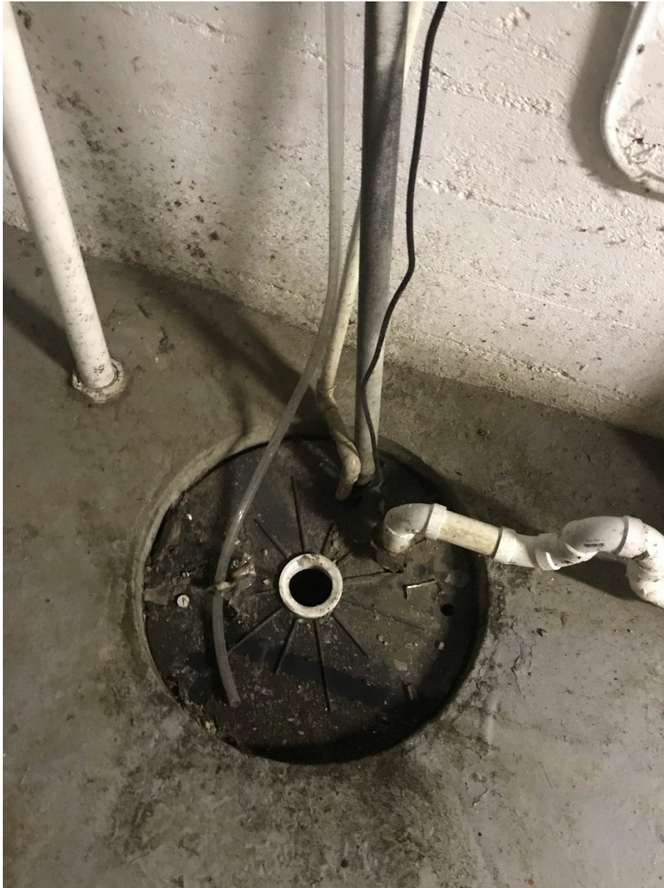
Photo 7: Looking at basement sump lid and southern vapor mitigation system pickup point. Owner had unsealed and removed sump lid. Floor is dry near sump.
