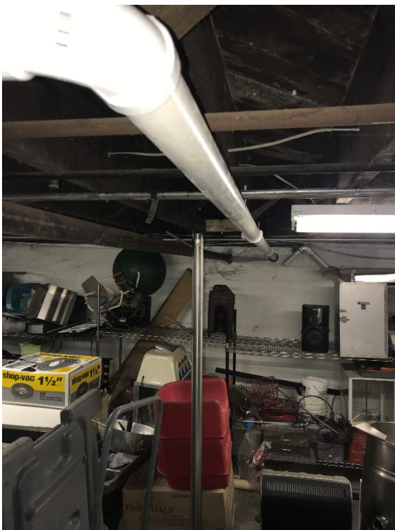
Photo 8: Looking south at lateral piping to southern pickup point. 11/21/18
