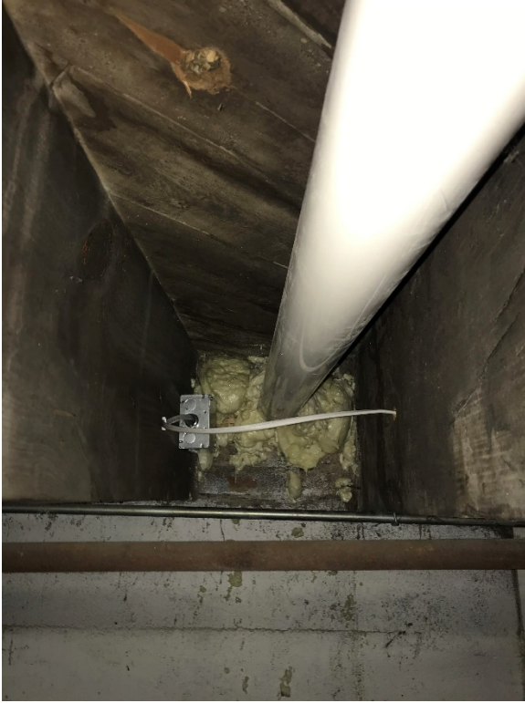
Photo 3: Looking north at ceiling from inside 5619 22 nd Avenue at electrical connection and pipe to fan. 11/21/18
