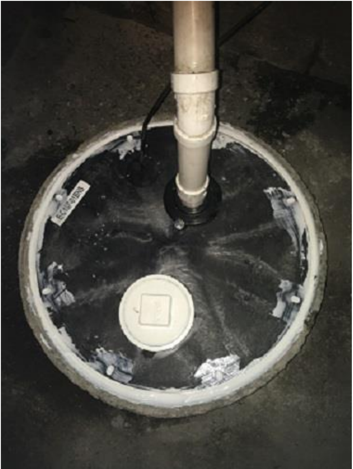
Photo #1: New vapor-tight basement sump lid with threaded plug to allow access for collecting samples.
