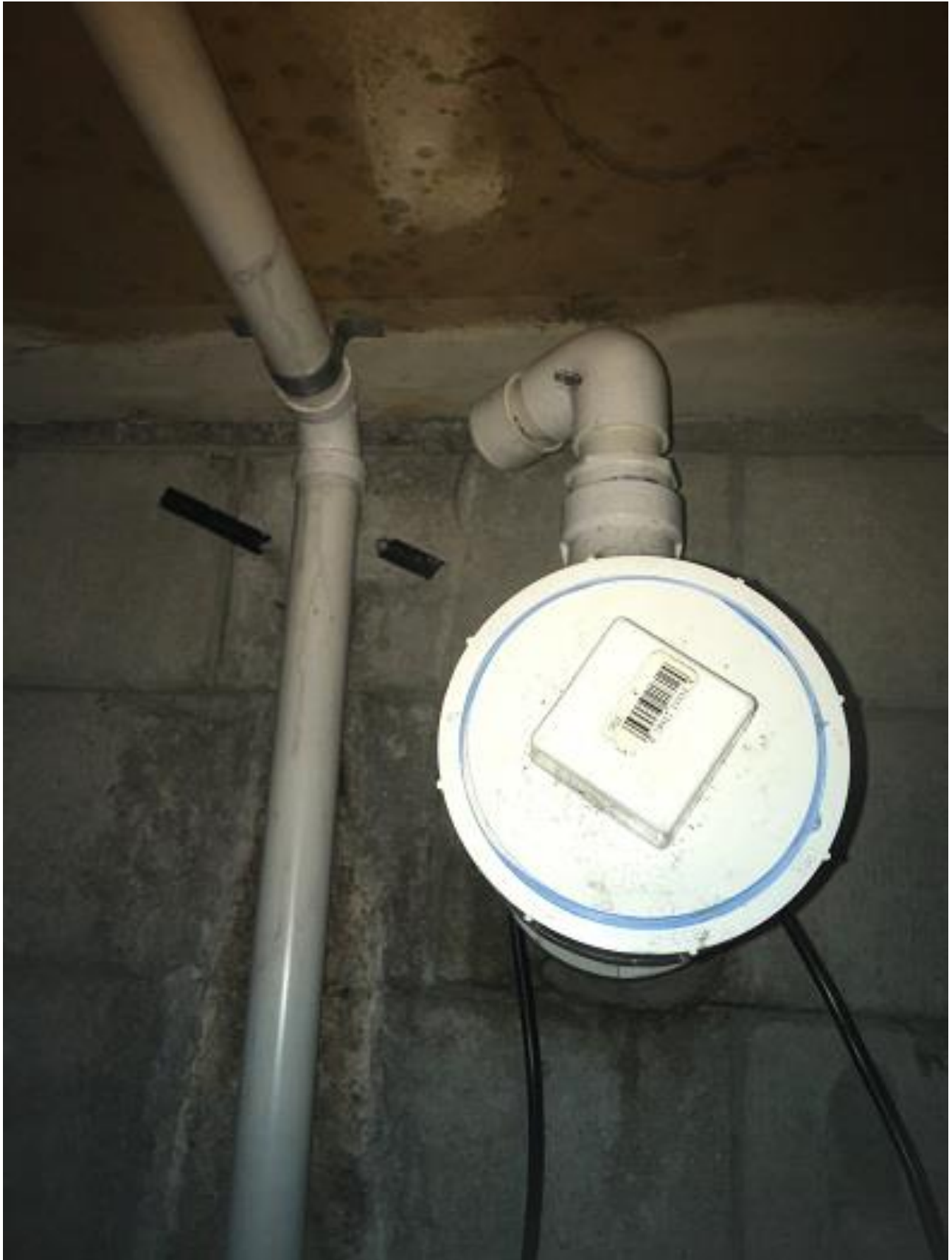
Photo #3: Close up showing that the sump discharge piping has been disconnected from the storm sewer lateral. The PVC elbow that formerly conveyed the sump discharge into the storm sewer lateral has been capped.
