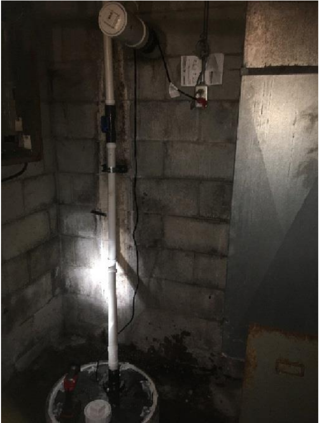
Photo #6: Flow volume totalizer installed on sump riser pipe approximately at same height as electrical outlet.
