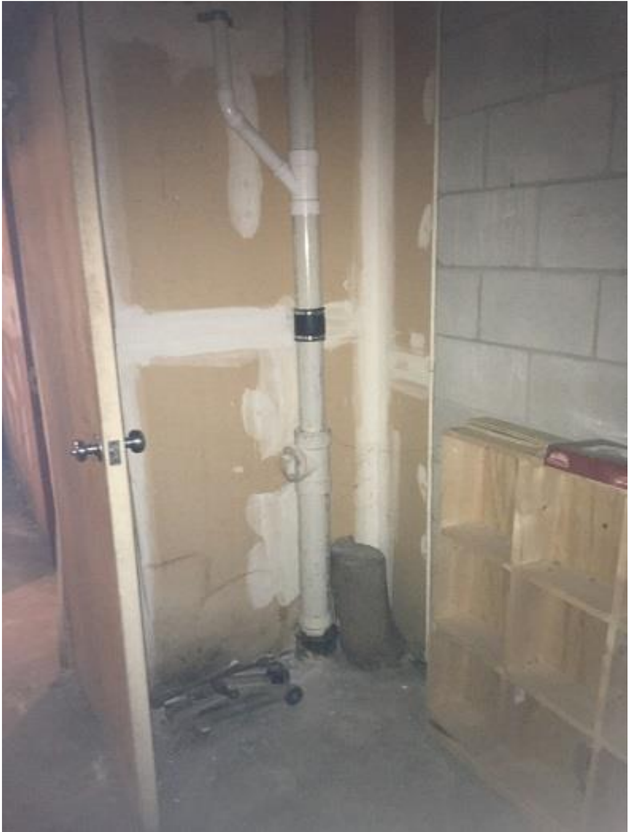
Photo #4: New sump discharge piping has been connected to a sanitary sewer lateral located just outside of the basement utility room.
