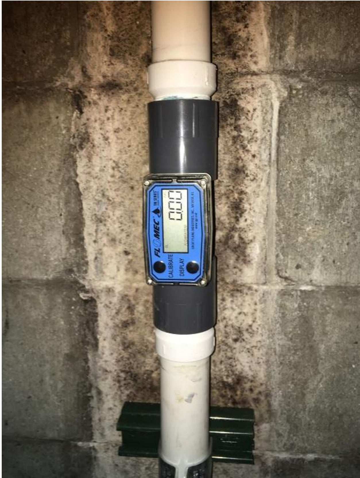
Photo #5: Flow volume totalizer installed on sump riser pipe.
