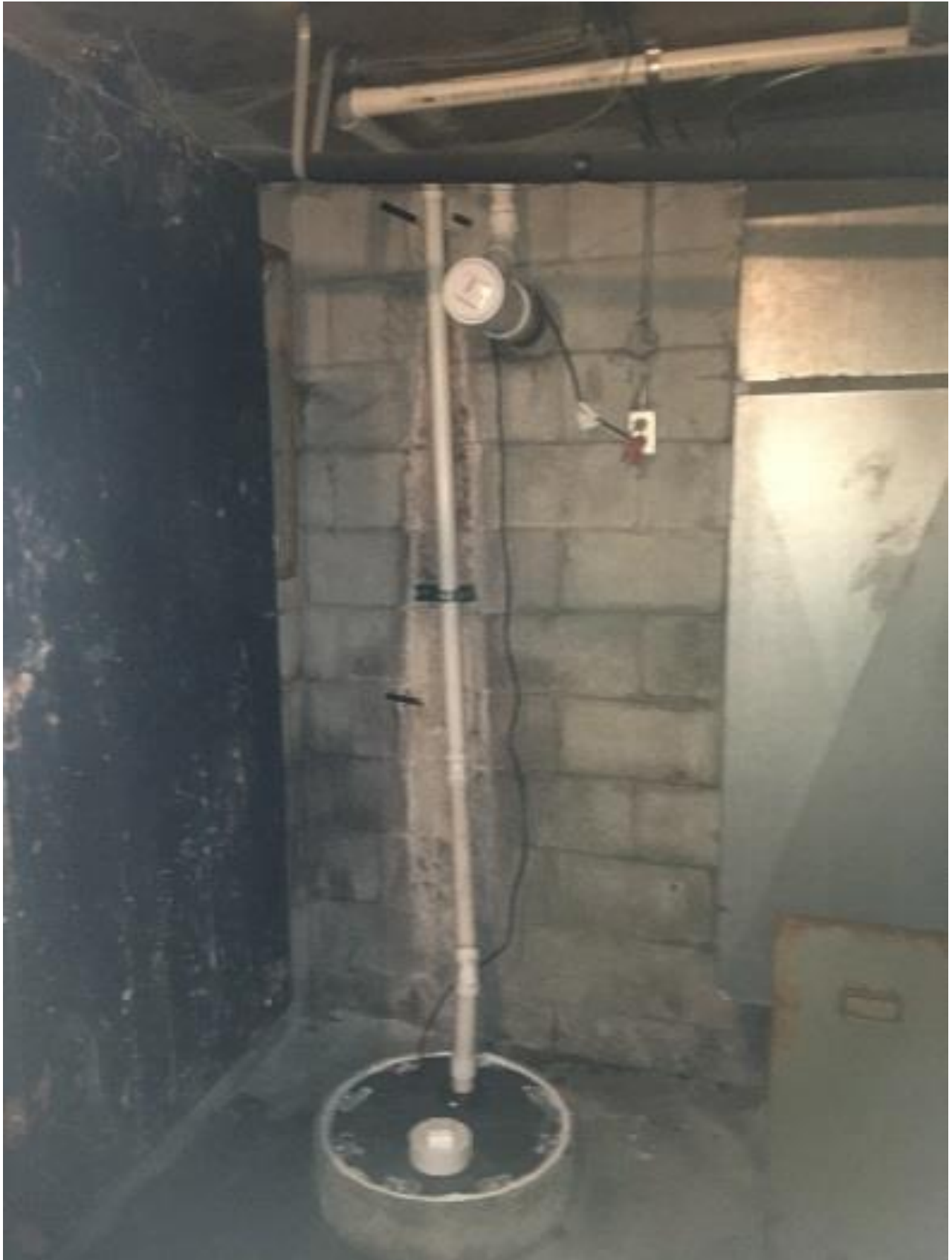
Photo #2: Basement sump and piping. Sump discharge has been disconnected from the storm sewer lateral seen adjacent right of the sump riser.
