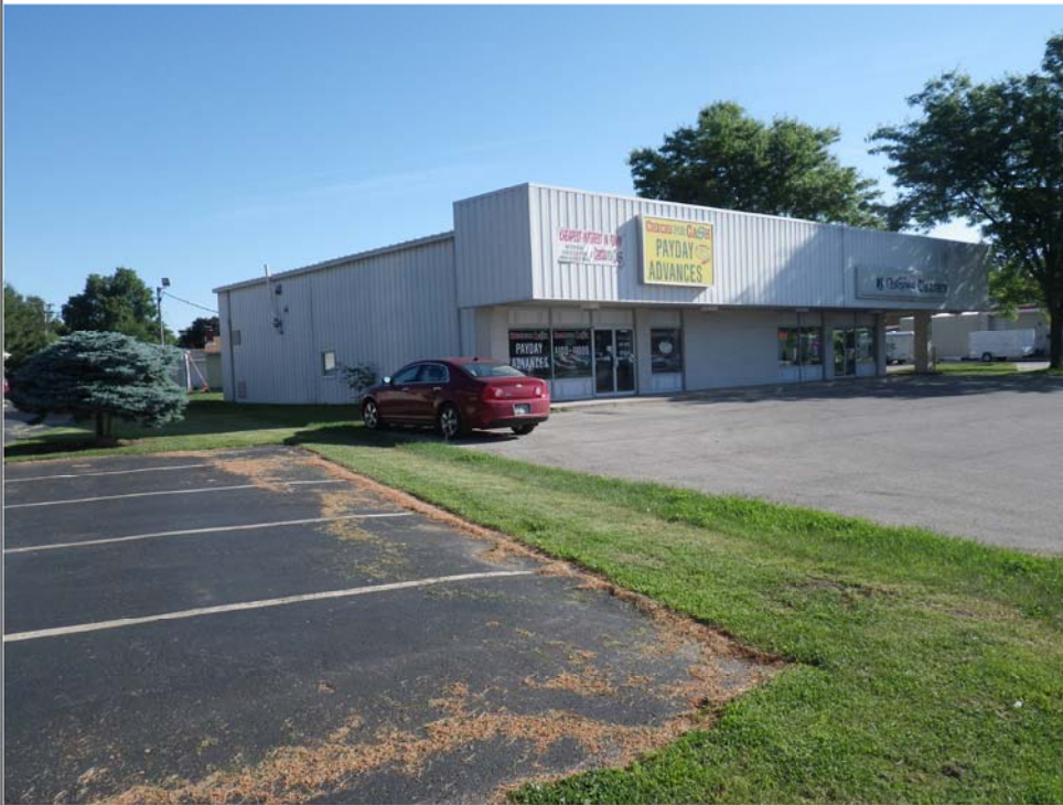
Title: Looking northeast from Milwaukee Street. Depressurization fan and stack visible on shady side of building.
