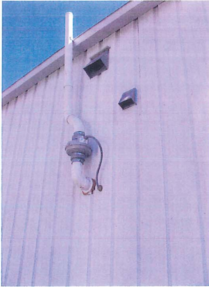
Photo 5 - In-line centrifugal fan and vent pipe
