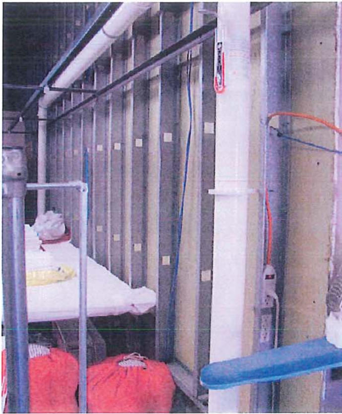
Photo 2 – front and middle extraction points with manometer gauge
