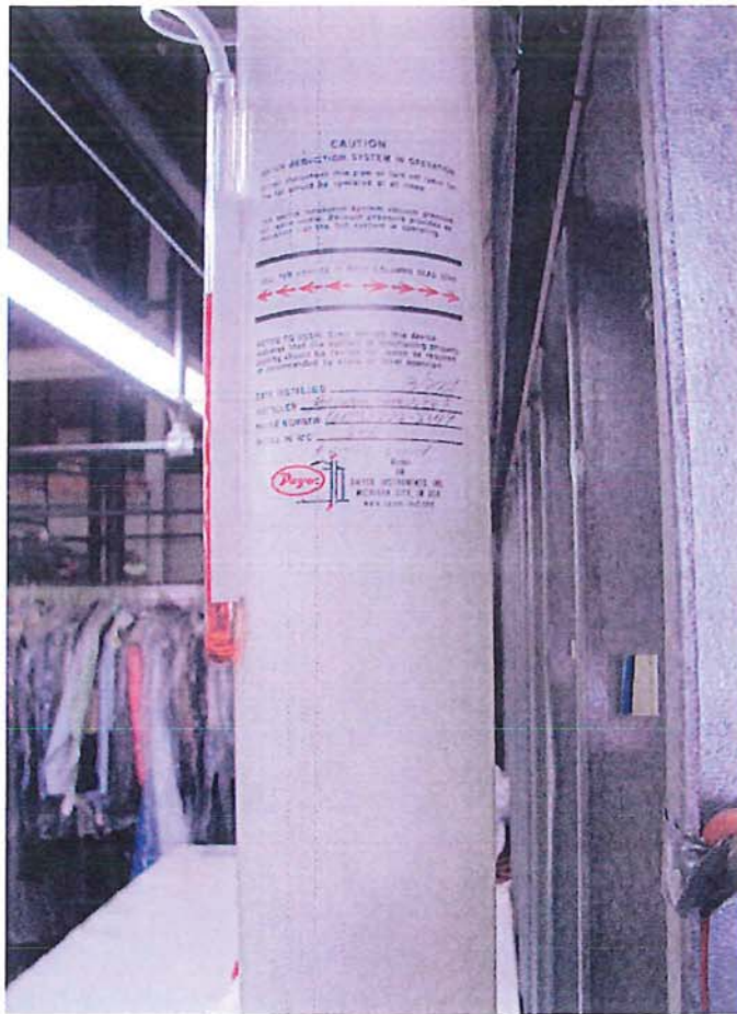
Photo 3 - Mitigation System description on middle extraction point
