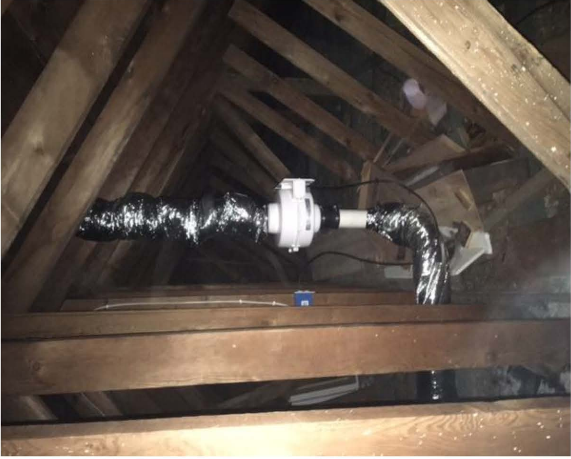
Depressurization Fan in Attic
