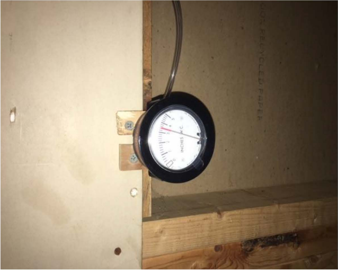
Vacuum on Depressurization Point 1
