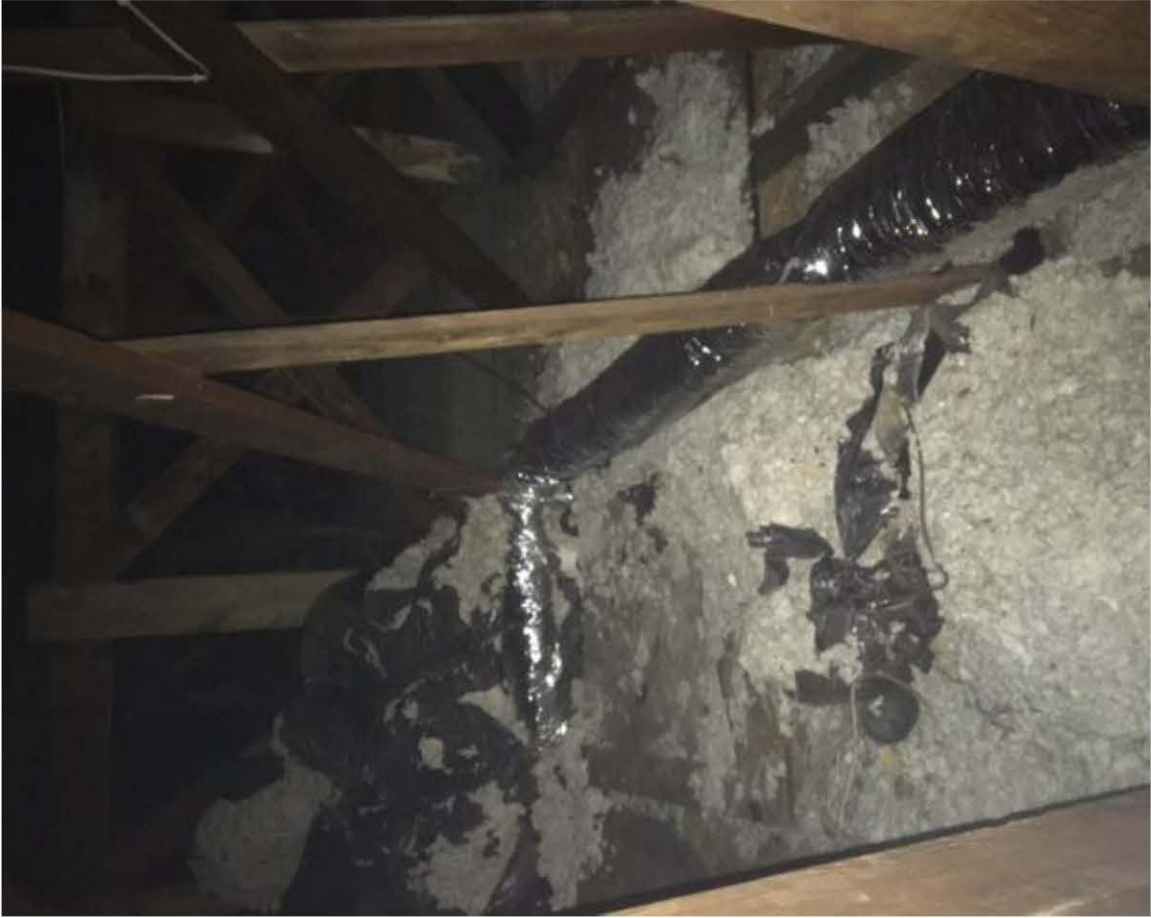
Insulated Depressurization Piping in Attic
