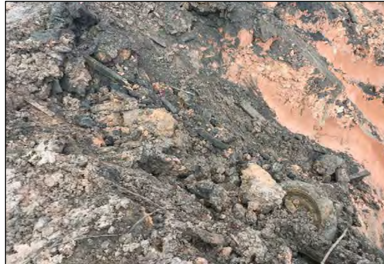
Buried debris and organics in new UST basin
