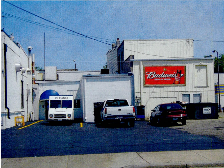
Greater detail of existing cap in area of MW-2, MW-4, PZ-5, MW-3 – west side of building looking east from Division Street
