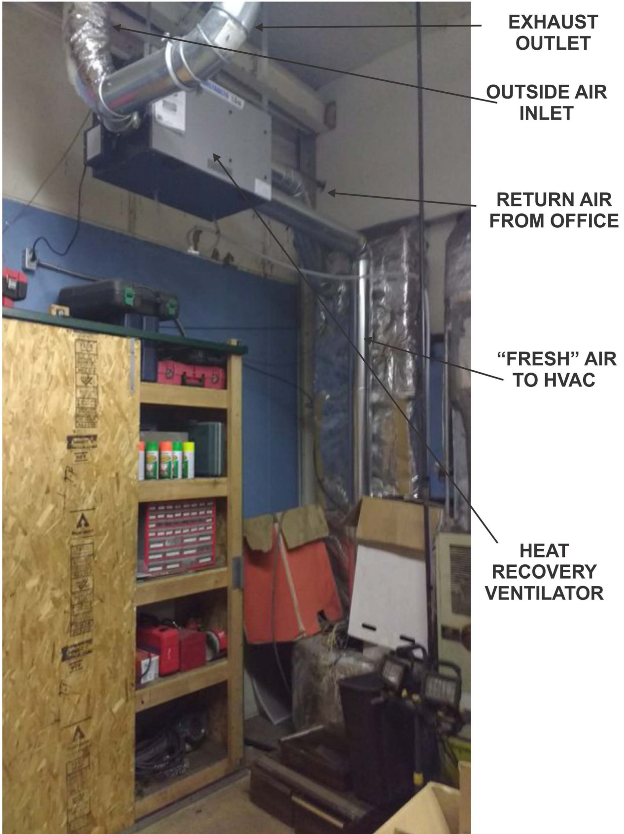
PHOTO 1 - Heat Exchange Ventilator and ducting components. In northwest corner of shop.
