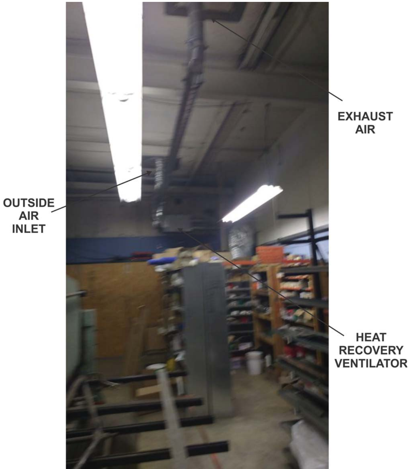
PHOTO 2 - Ductwork showing the roof penetrations for ventilator the intake and exhaust air.
