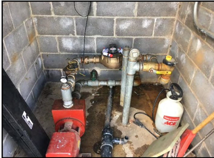
Sprinkler well pump house
