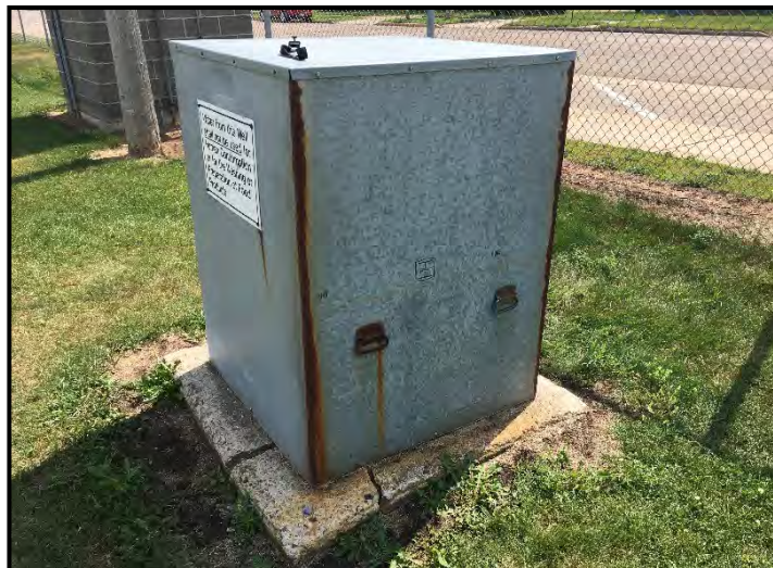
Witter Field sprinkler wells
