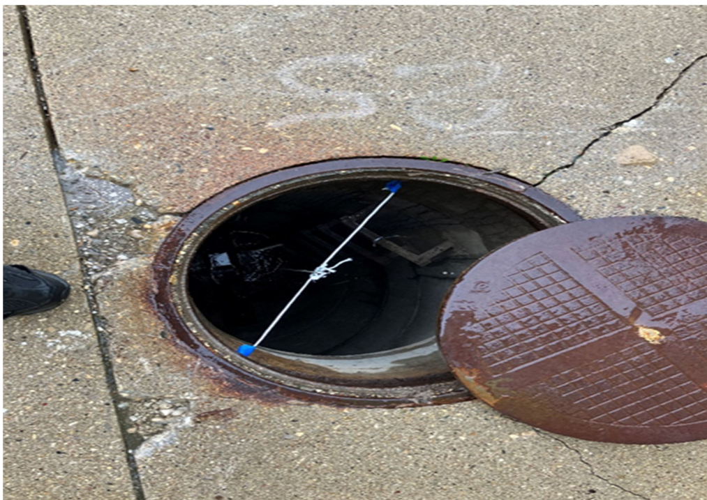
Photo 4: Sanitary Sewer Manhole 25 (IA-1) with magnets/nylon string for passive vapor sampler support.
