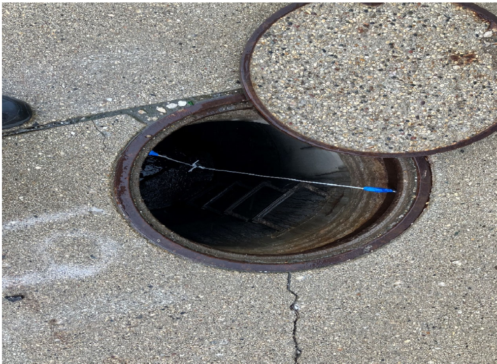
Photo 2: Sanitary Sewer Manhole 19 (IA-3) with magnets/nylon string for passive vapor sampler support.
