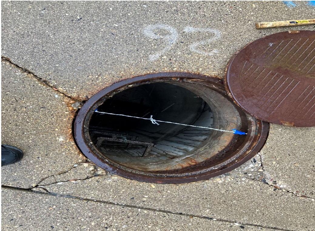
Photo 3: Sanitary Sewer Manhole 26 (IA-2) with magnets/nylon string for passive vapor sampler support.
