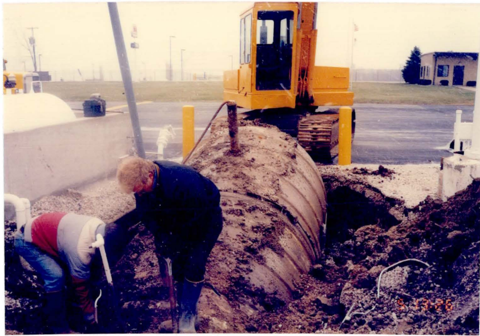
2. South end of UST rises above surface level after fiberglass straps are cut.
