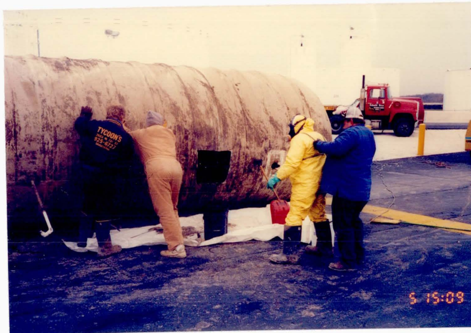
5. Disabled Additive UST; Schmidt Bros. employee outfitted in Level C preparing to extract sludge from UST.
