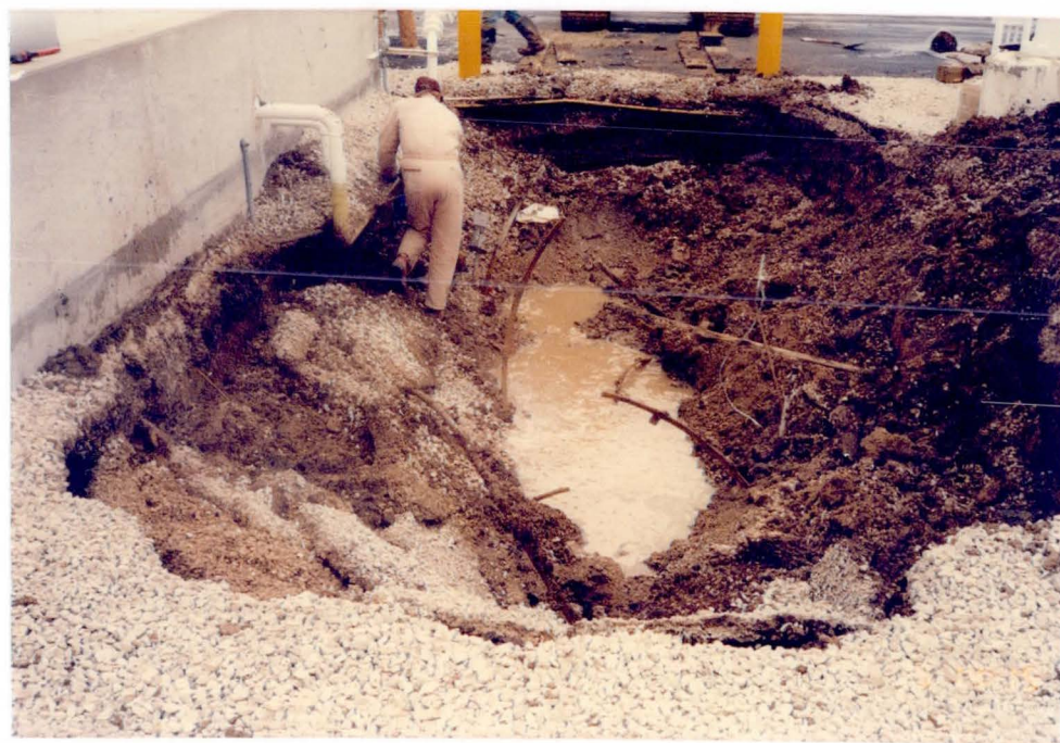
4. Collapsed backfill and standing water in excavation.
