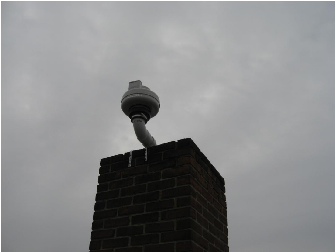
Photograph #: 5 Date: 9/28/2012 Direction: Jackson Plaza System #1 Subject: Fan mounted on chimney
