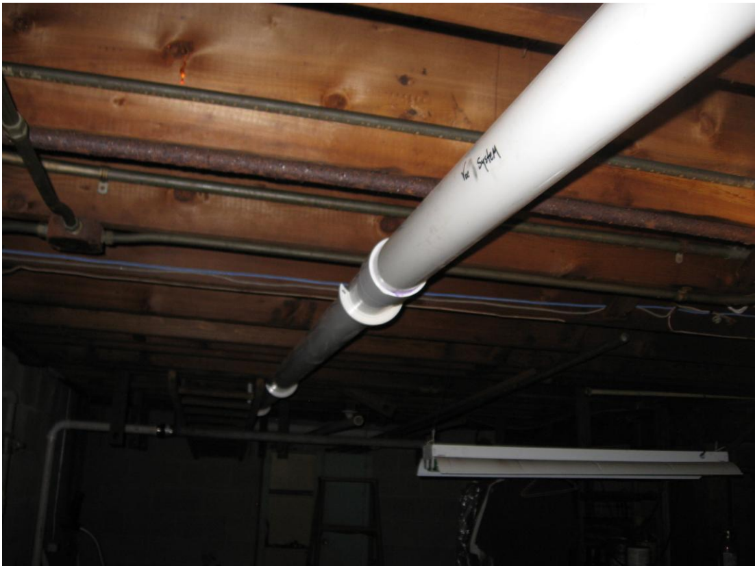
Photograph #: 2 Date: 10/26/2012 Direction: One Hour Cleaners (Site building) System Subject: Piping to block wall suction points
