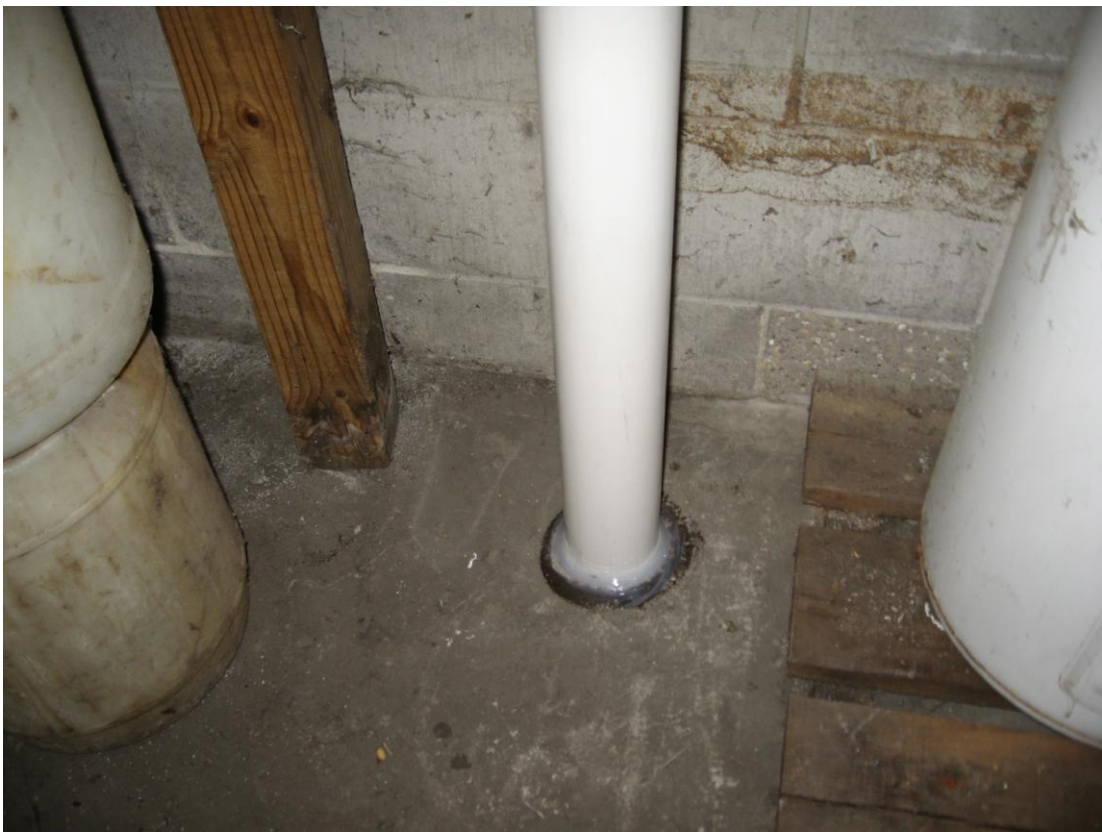
Photograph #: 1 Date: 10/26/2012 Direction: One Hour Cleaners (Site building) System Subject: Sub-slab suction point in basement
