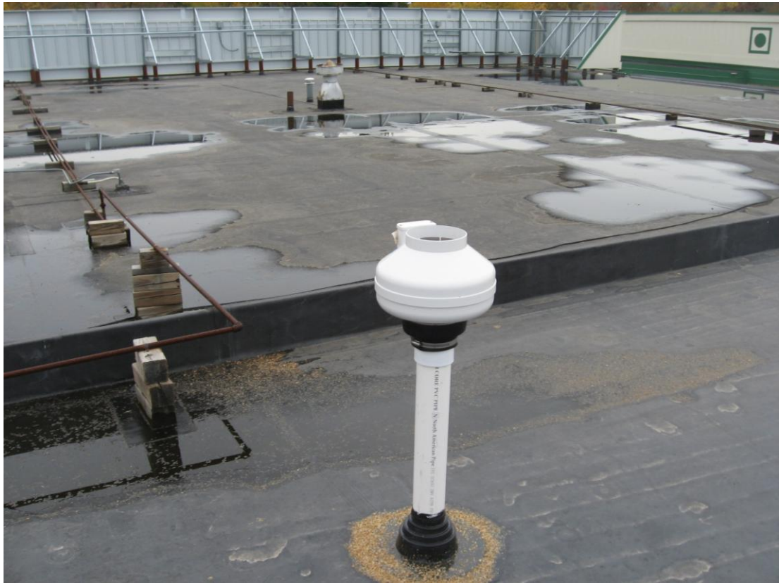
Photograph #: 9 Date: 10/11/2012 Direction: Jackson Plaza System #2 Subject: Fan mounted on roof
