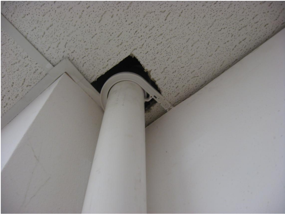
Photograph #: 7 Date: 9/28/2012 Direction: Jackson Plaza System #2 Subject: Exhaust piping exit through roof
