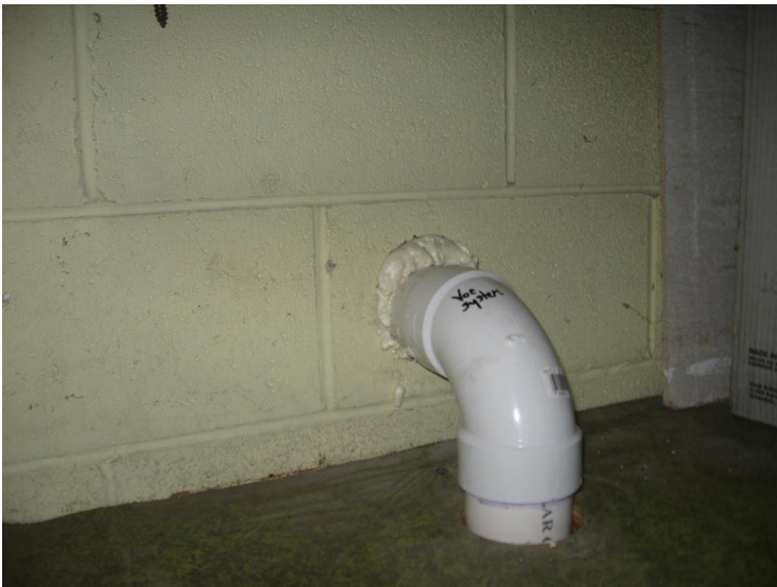
Photograph #: 5 Date: 10/26/2012 Direction: One Hour Cleaners (Site building) System Subject: Exhaust piping exit through wall on main floor
