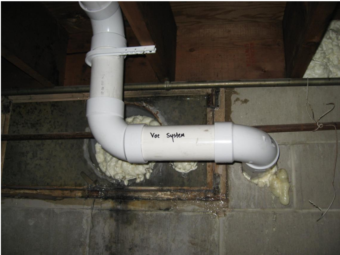
Photograph #: 4 Date: 10/26/2012 Direction: One Hour Cleaners (Site building) System Subject: Block wall suction point
