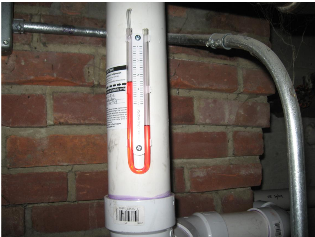
Photograph #: 4 Date: 9/28/2012 Direction: Jackson Plaza System #1 Subject: U-tube monometer
