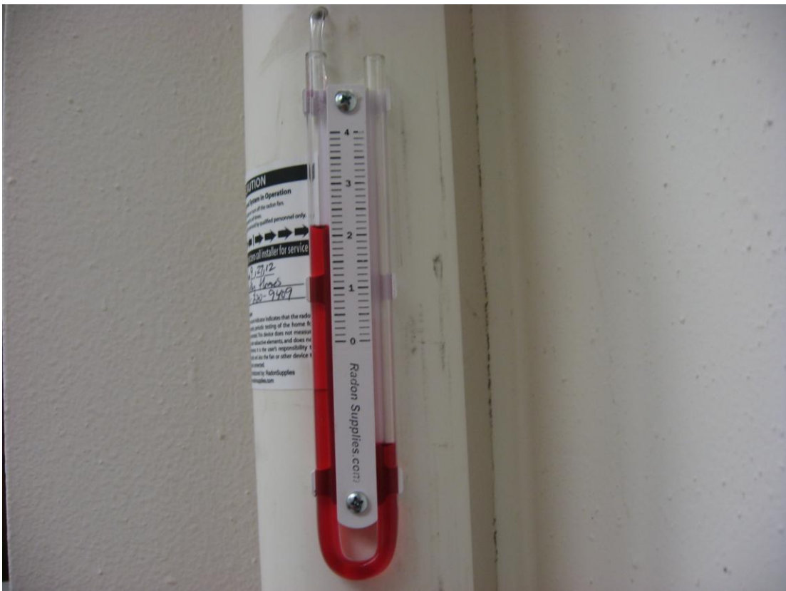
Photograph #: 8 Date: 9/28/2012 Direction: Jackson Plaza System #2 Subject: U-tube monometer
