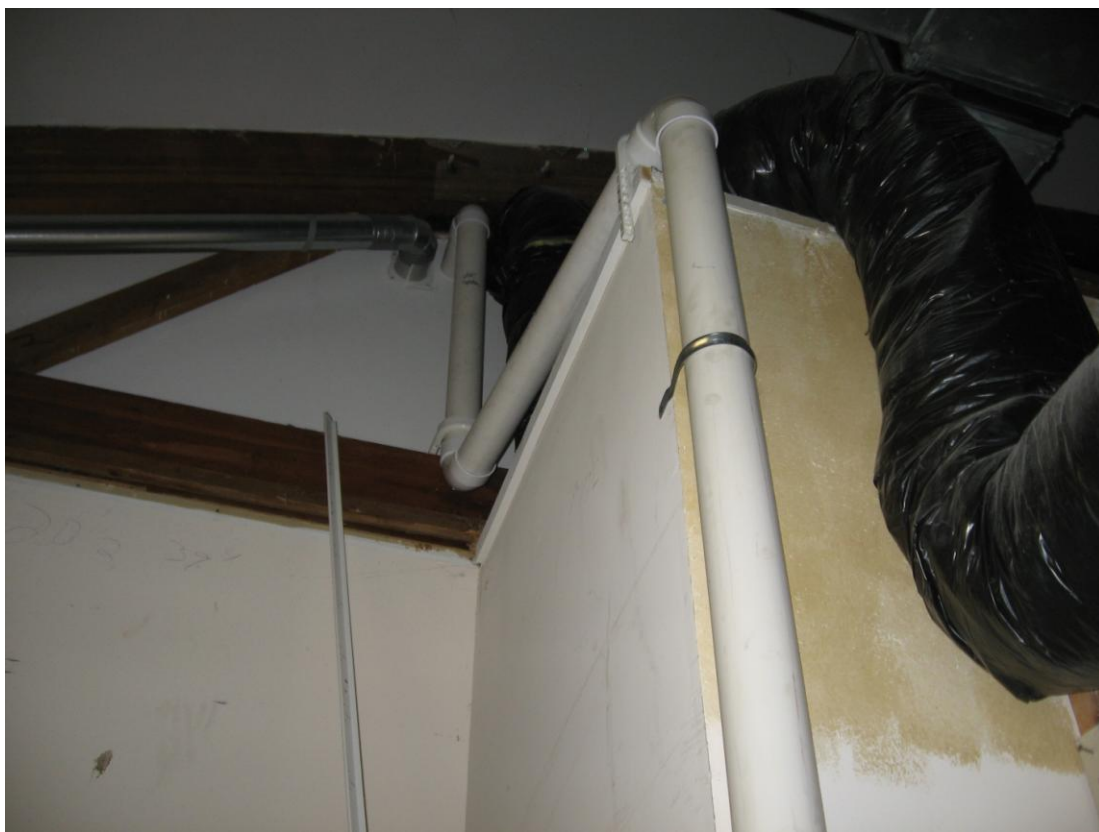
Photograph #: 11 Date: 10/11/2012 Direction: Jackson Plaza System #3 Subject: Exhaust piping exit through roof
