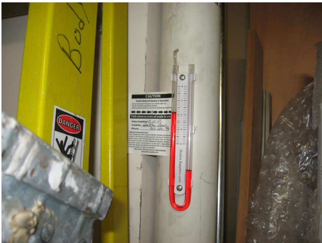
Photograph #: 12 Date: 10/11/2012 Direction: Jackson Plaza System #3 Subject: U-tube monometer
