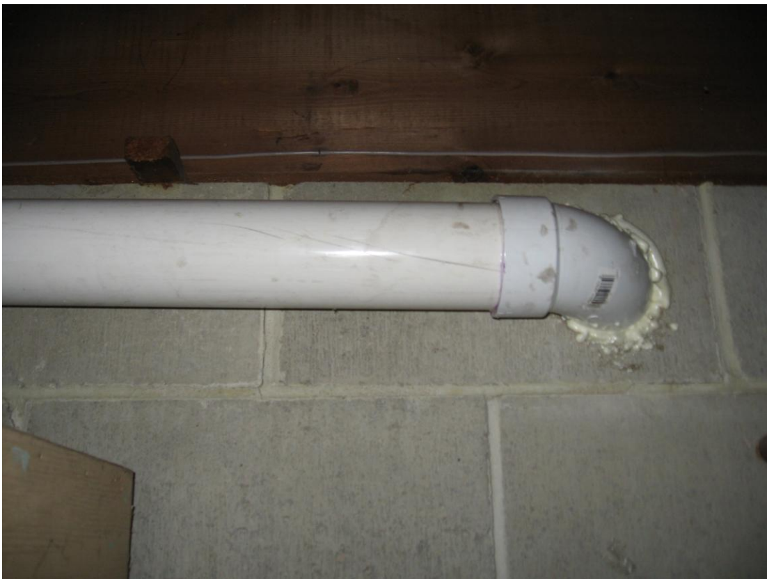
Photograph #: 3 Date: 10/26/2012 Direction: One Hour Cleaners (Site building) System Subject: Block wall suction point
