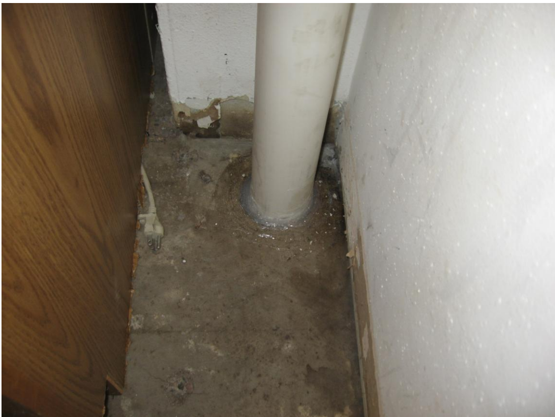
Photograph #: 6 Date: 9/28/2012 Direction: Jackson Plaza System #2 Subject: System suction point in A-1 Vacuum tenant space
