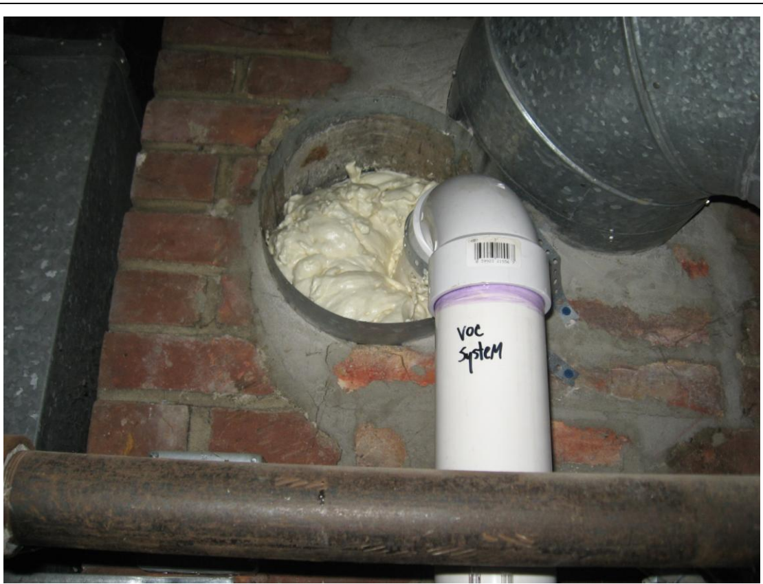
Photograph #: 3 Date: 9/28/2012 Direction: Jackson Plaza System #1 Subject: Exhaust piping exit through existing chimney
