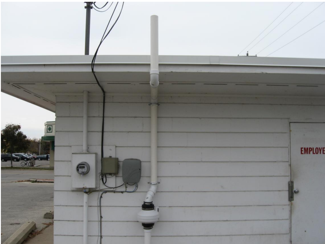
Photograph #: 6 Date: 10/26/2012 Direction: One Hour Cleaners (Site building) System Subject: Fan mounted on north side of building
