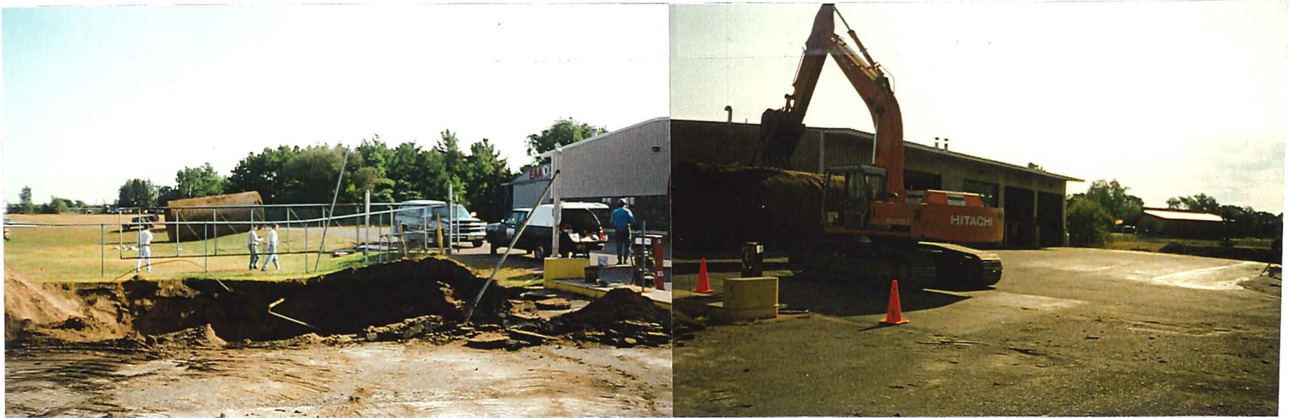
Photo 1 Gasoline and diesel tank excavation. Gasoline tank is in far left background. Diesel tank is in transportation.
