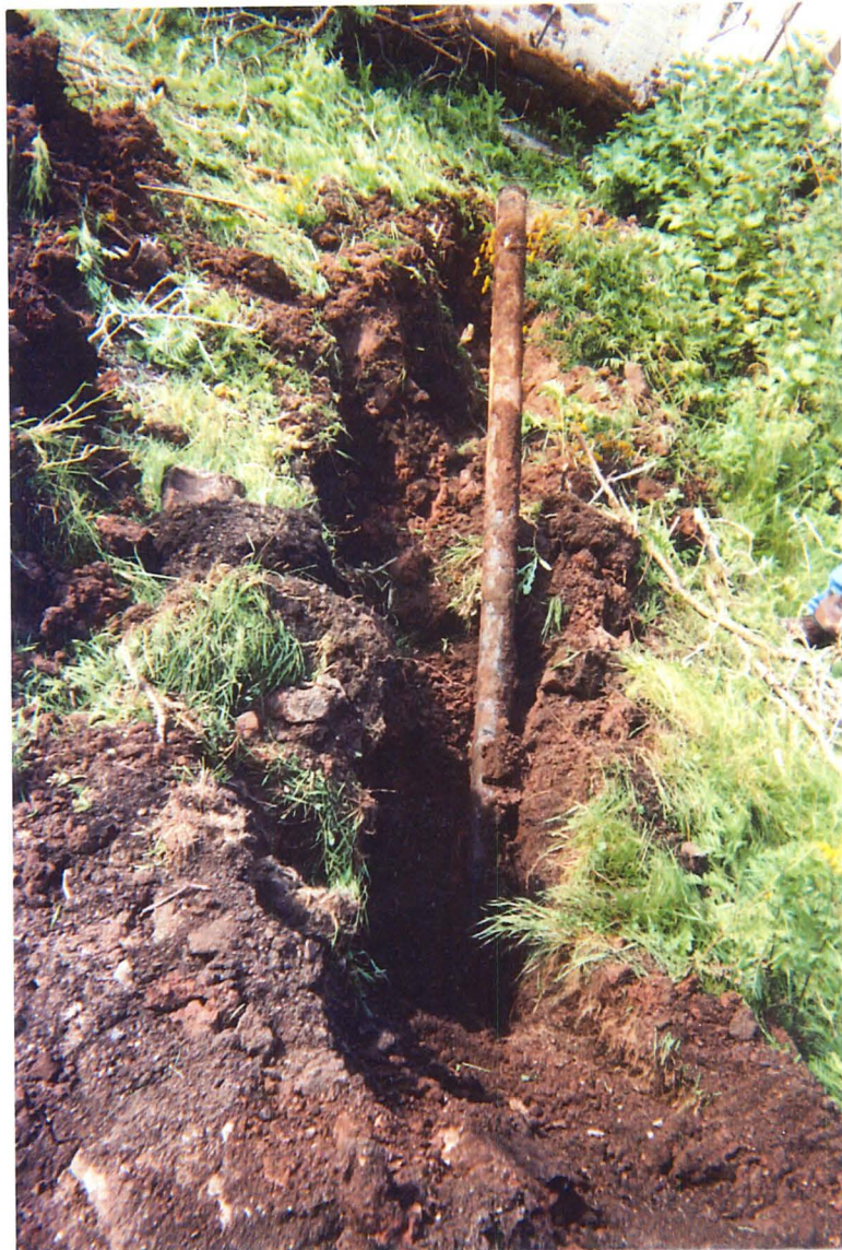
Photo 1: View of 5-inch steel pipe at south end of excavation with building in background.
