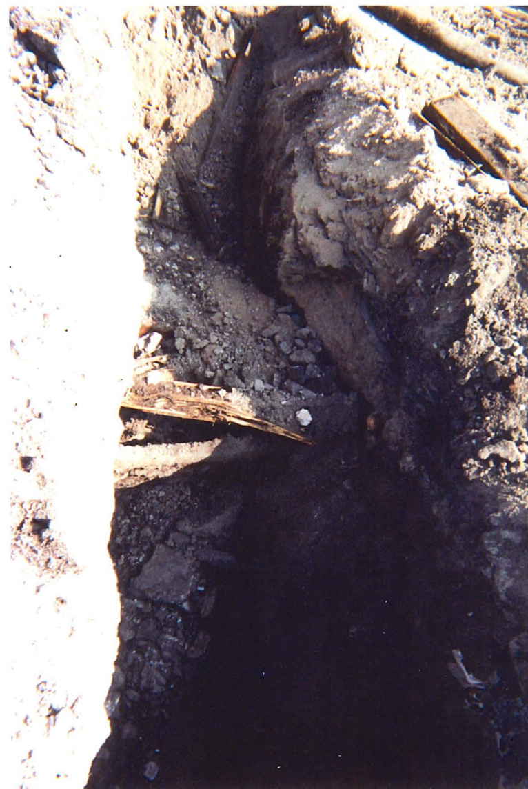
Photo 2: View of timber box discovered surrounding the steel pipe. The soil type is the gray lime-like fill material.
