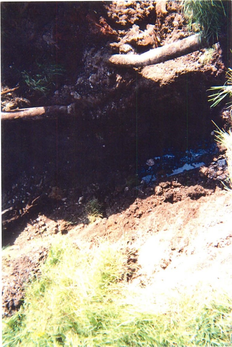
Photo 3: View of excavation looking down with water in bottom of excavation from 12-inch clay pipe.
