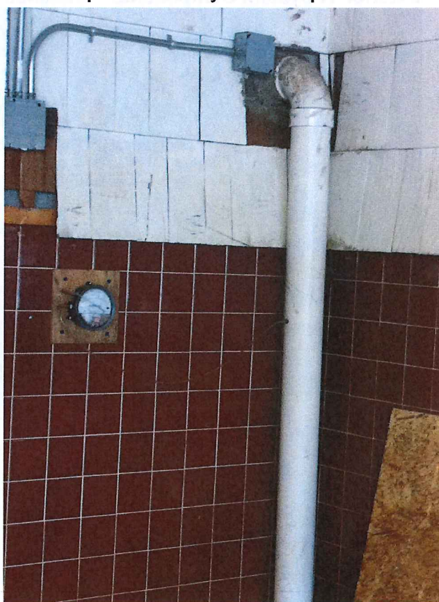
Close-up of Internal System Components
