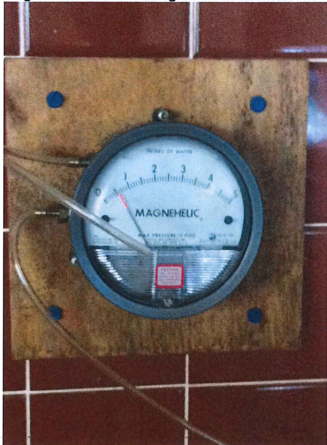
Magnehelic Meter Reading at ~6 inches of Water
