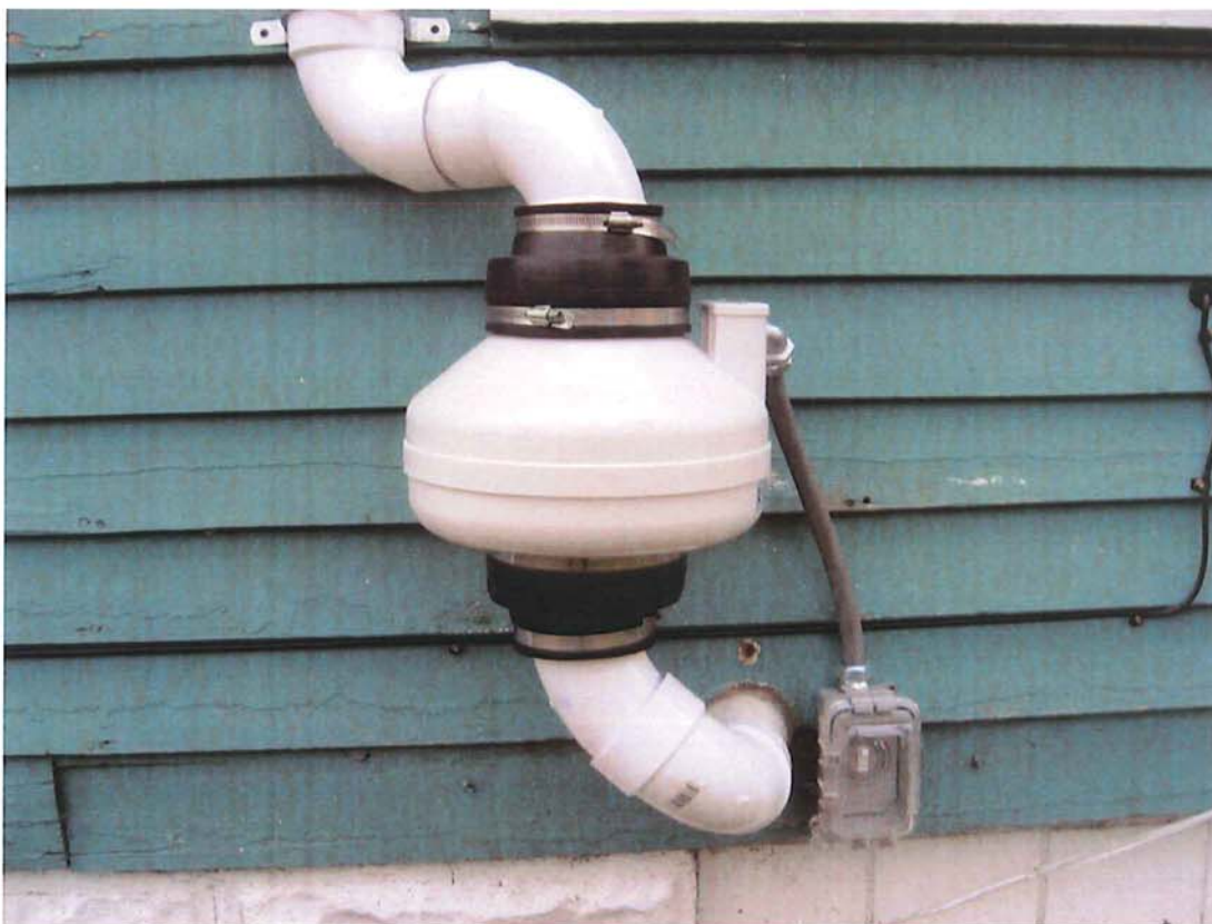
Photograph #: 2 Date: 11/9/2012 Direction: East side of building Subject: System fan and on/off switch
