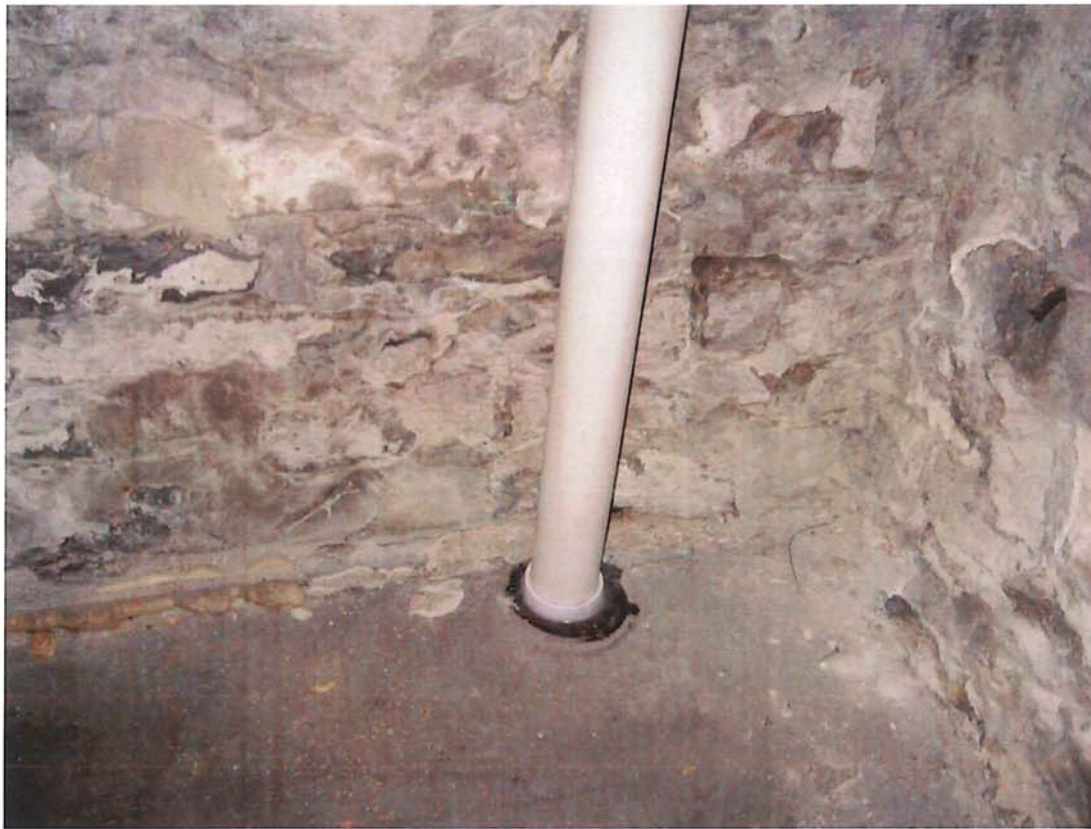
Photograph #: 3 Date: 11/9/2012 Direction: Basement Subject: System suction point
