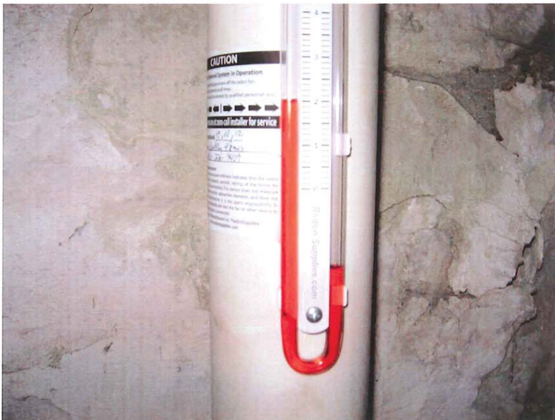
Photograph #: 4 Date: 11/9/2012 Direction: Basement Subject: U-tube monometer
