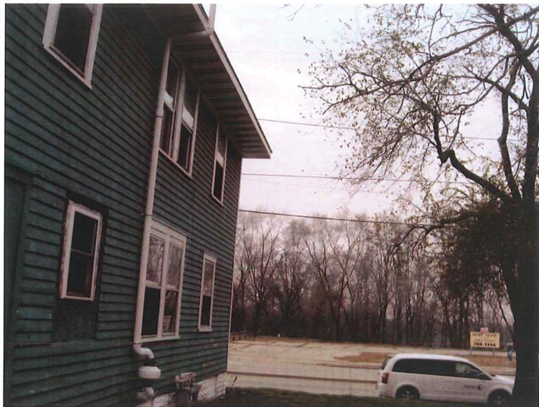
Photograph #: 1 Date: 11/9/2012 Direction: Facing North Subject: Sub-slab depressurization system fan and exhaust
