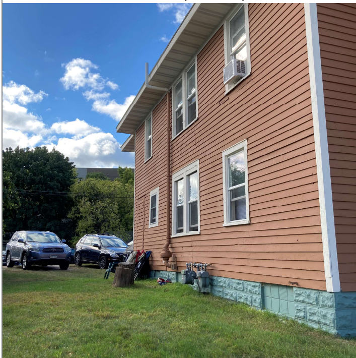
Title: One Hour Cleaners La Crosse Street/0232279690/20220926/ Affected property SSDS exhausting to roof
