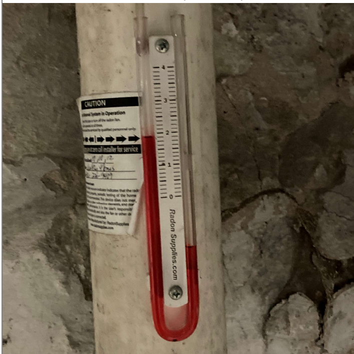
Title: One Hour Cleaners La Crosse Street/0232279690/20220926/ Affected property manometer with correct reading
