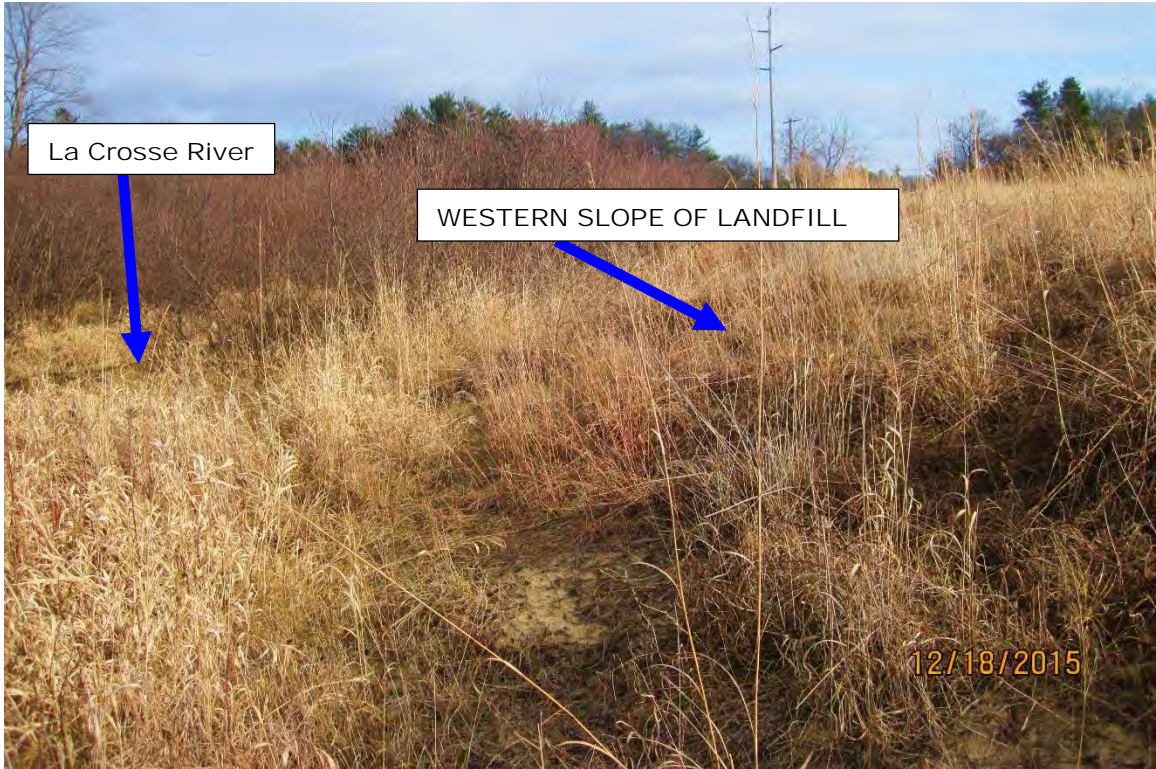
THE CAP OVER THE WESTERN SLOPE ALONG THE RIVER IS CONSTRUCTED OF 12 INCHES OF FILL OVERLAIN BY A GEOTEXTILE FABRIC, WHICH IS OVERLAIN BY 18-24 INCH RIPRAP ARMORING COVERED BY 2-4 INCHES OF SAND VEGETATED WITH NATIVE PRAIRE GRASS. (VIEW IS TO THE NORTH)
