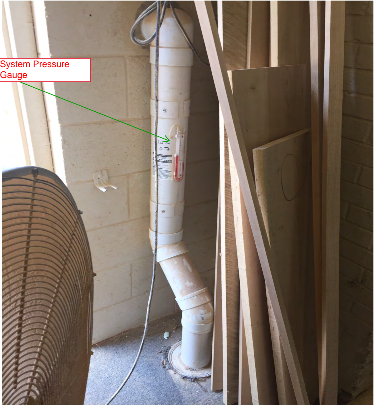
East vapor extraction system interior piping showing the piping going into the sub slab and venting outside of the building.
