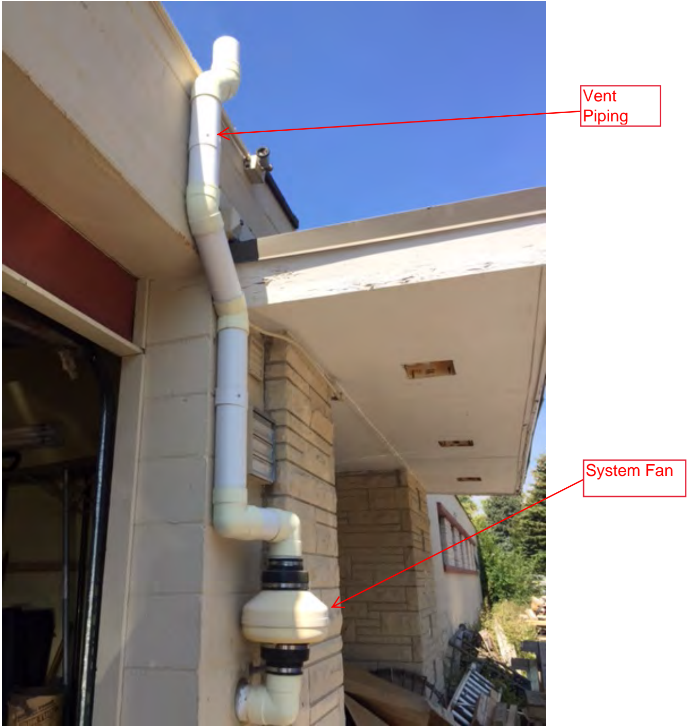
Vapor system located on the east side of the building showing the vent piping going up to the roof line of building.
