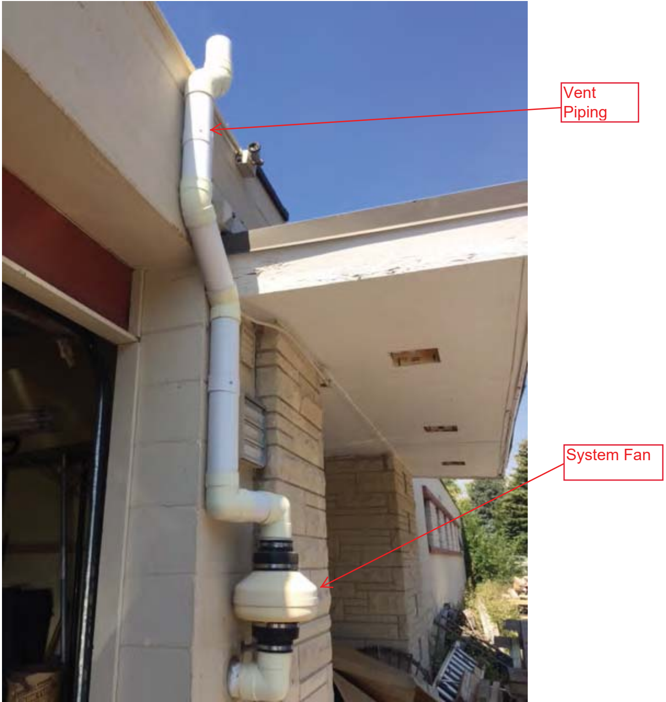
Vapor system located on the east side of the building showing the vent piping going up to the roof line of building.
