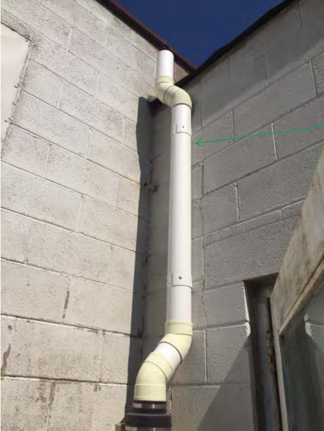
Vapor system located on the west side of the building showing the vent piping going up to the roof line of building.
