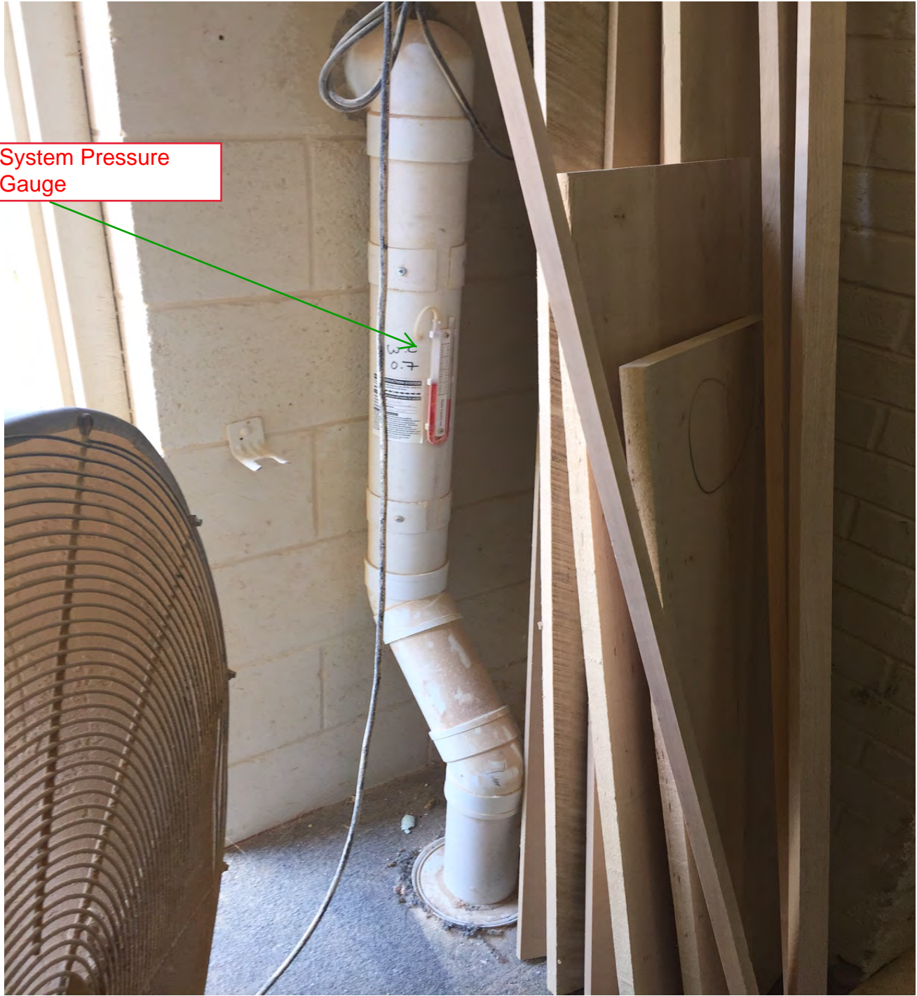
East vapor extraction system interior piping showing the piping going into the sub slab and venting outside of the building.
