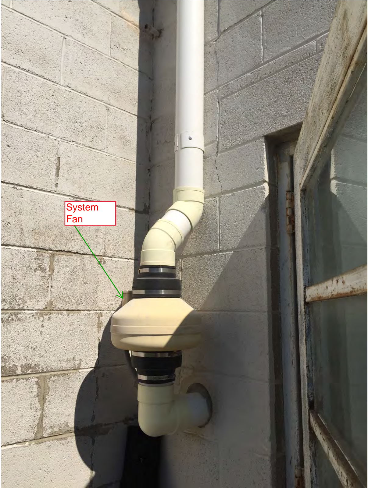
Vapor system located on the west side of the building showing the fan and vent piping going up to the roof line of building.
