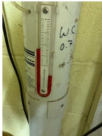
Description: Fan #1 pressure
