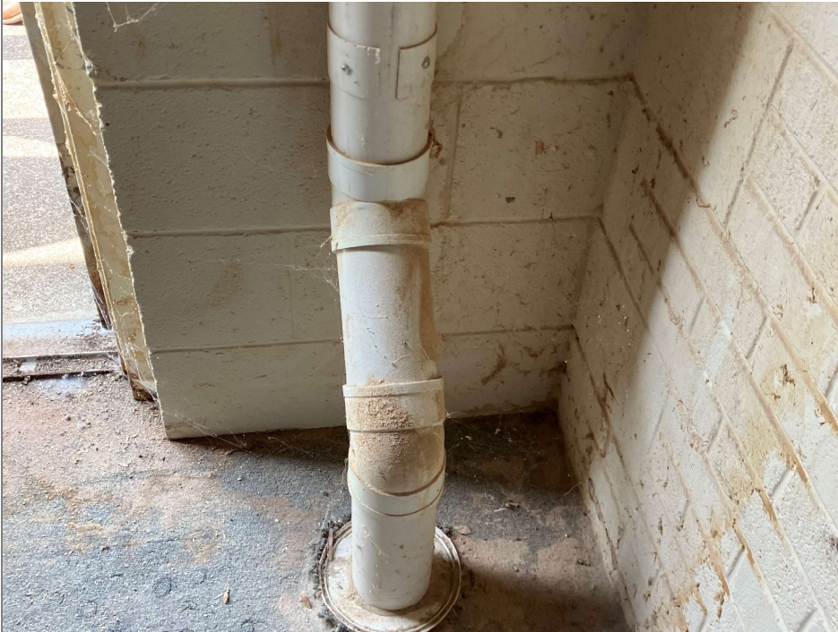
Title: West side piping
