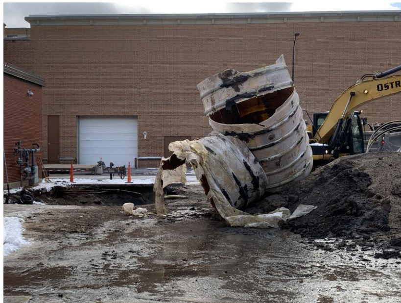
10,000-gallon gasoline after removal. Concrete ballast over tank caused it to split during removal.
