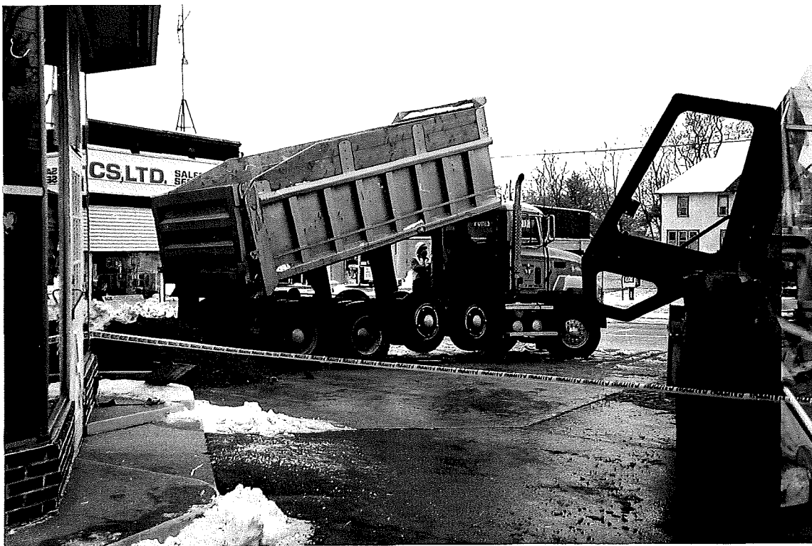
PHOTOGRAPH 4: Backfilling of the excavation with imported fill material following collection of confirmation samples.
