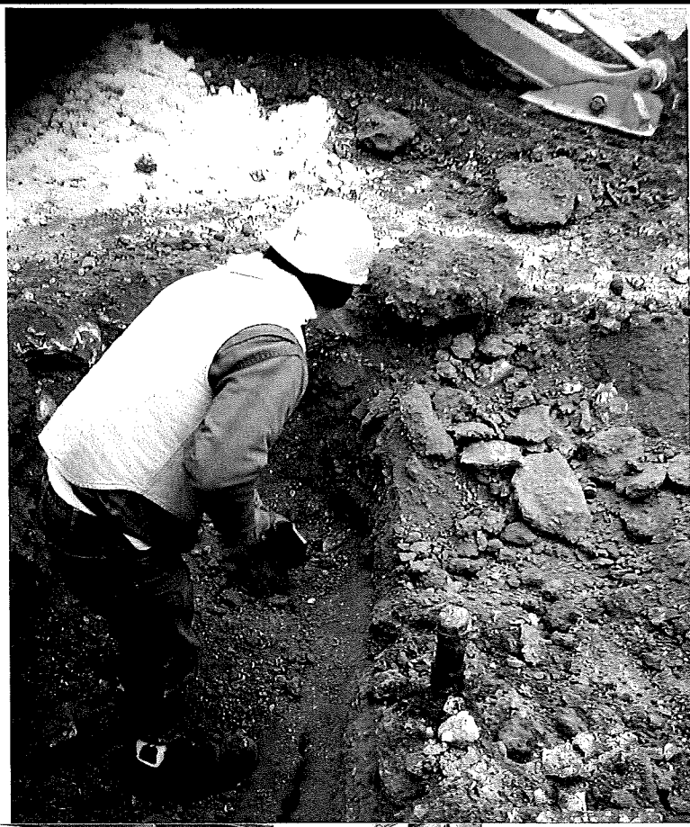
PHOTOGRAPH 1: A worker from North Shore Environmental Construction is exposing the top of the 550-gallon fuel oil UST.
