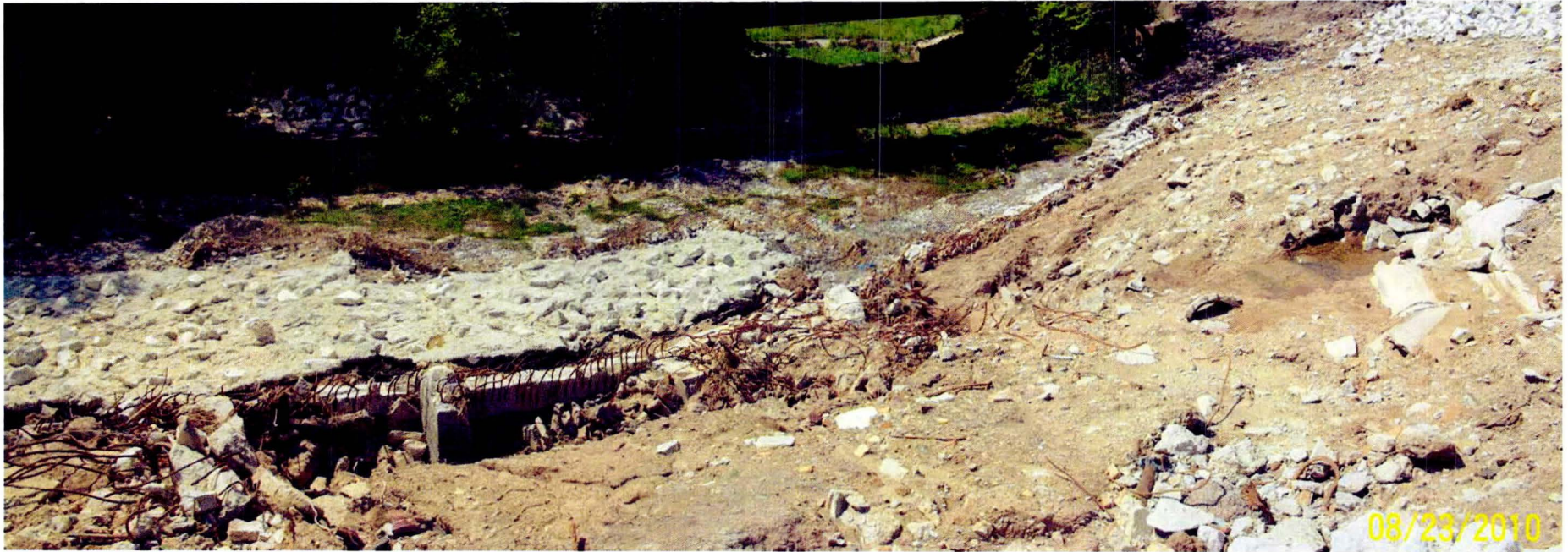
View of bank area looking west after flood damage and with former building footing walls cut down.
