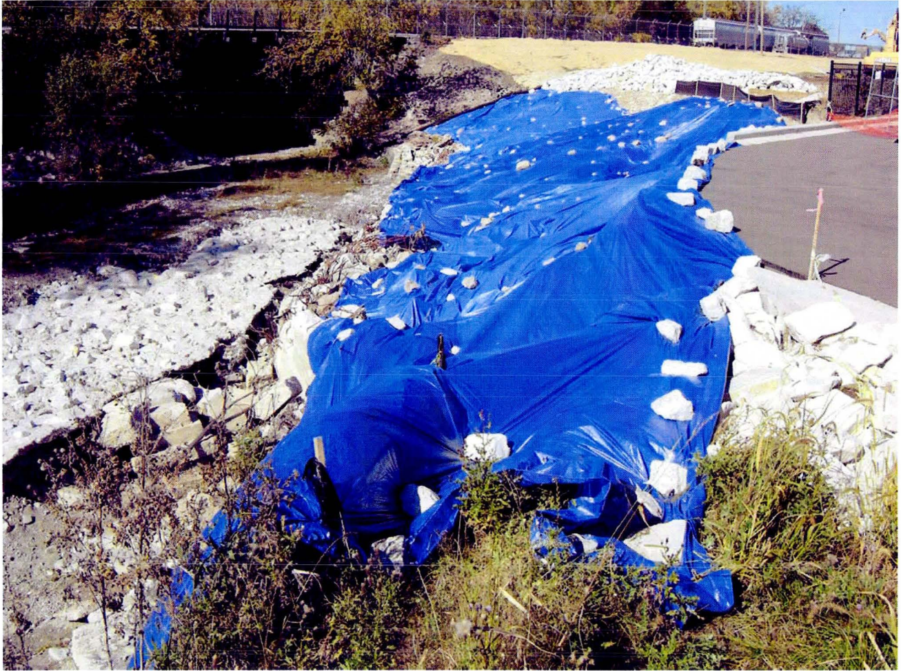
View of bank area looking west with temporary tarps placed to limit erosion and runoff.
