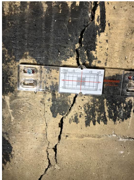
Photo 2: Building crack monitor and interior west wall on May 24, 2018.
