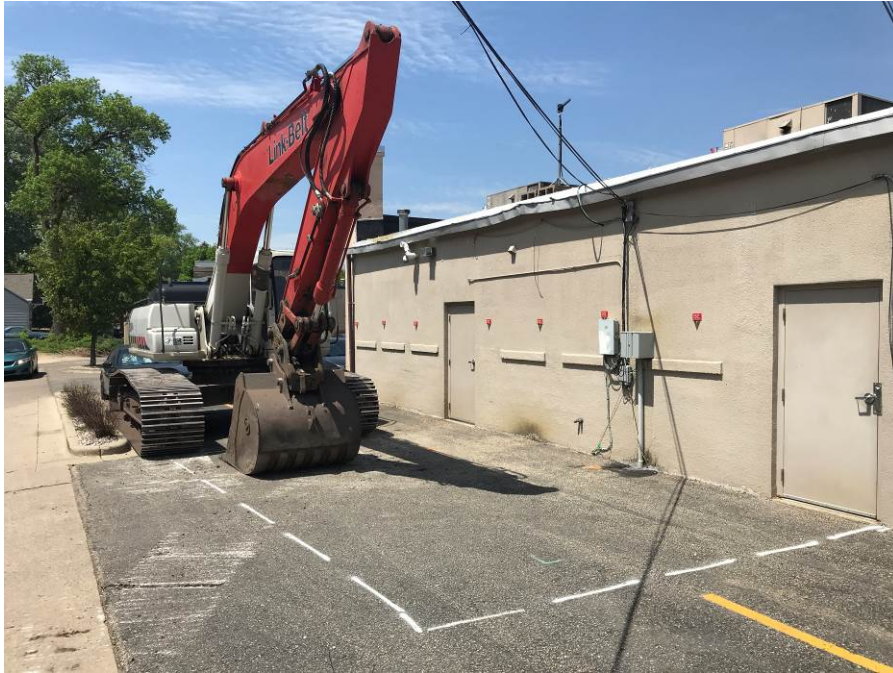
Photo 1: Looking northwest at south side of building on May 18, 2018, prior to excavation. Orange boxes on building wall are survey control points.
