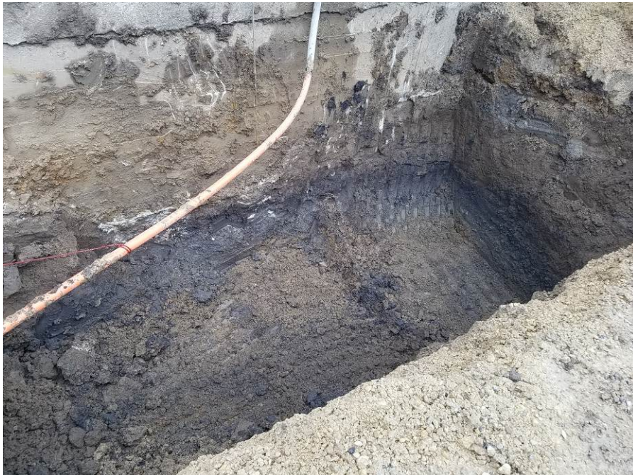
Photo 6: Looking northeast at east end of excavation along southern wall of the building on May 22, 2018. Conduit shown in photo is fiber optic line.
