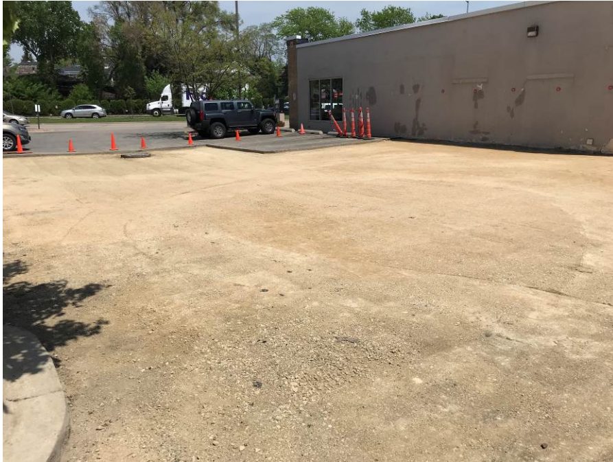
Photo 15: Looking northeast at base course along west side of building on May 24, 2018.
