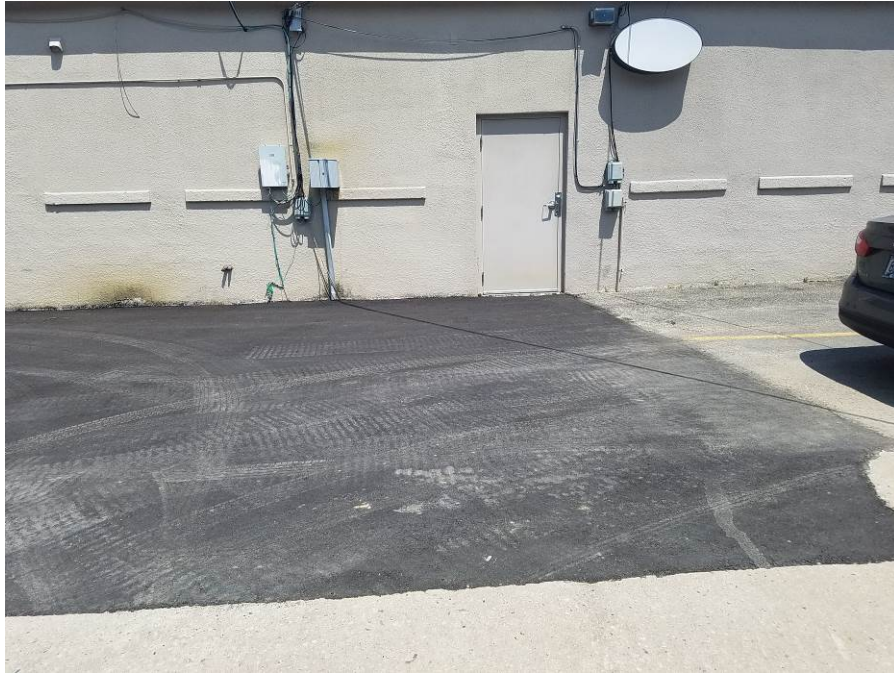
Photo 17: Looking north at new pavement at south end of building on June 7, 2018.
