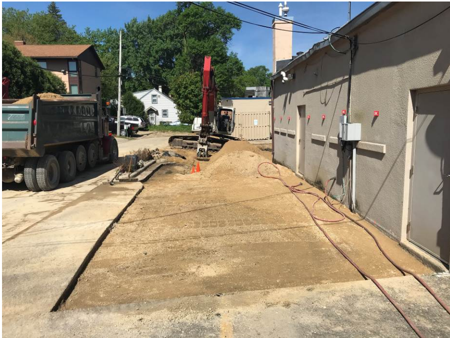
Photo 12: Looking west at excavation and compaction from west side of excavation area on May 23, 2018.
