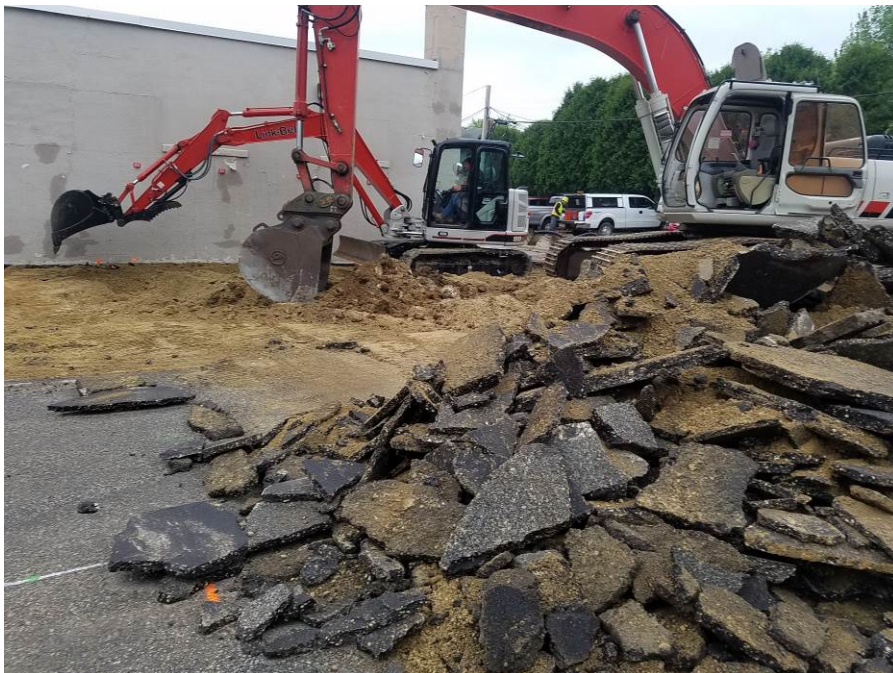
Photo 4: Looking southeast at west side of building during removal of asphalt on May 21, 2018. Orange boxes on wall behind excavator are survey control points.
