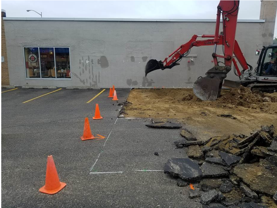
Photo 3: Looking east at west side of building during removal of asphalt on May 21, 2018.
