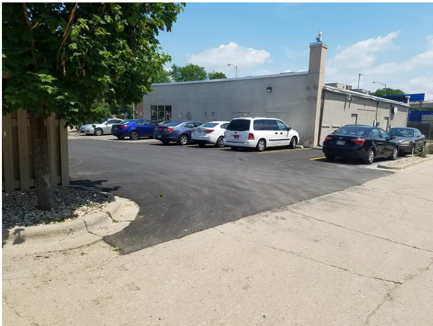
Photo 20: Looking northeast at new pavement from south side of the property on June 7, 2018. Note property owner paid for the additional base course and pavement beyond that replaced as part of the remedial action.
