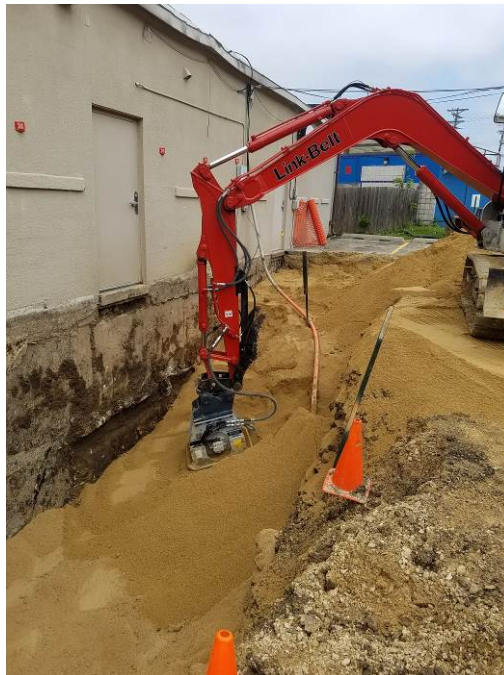
Photo 10: Looking east at backfill and compaction along south wall of building on May 22, 2018.
