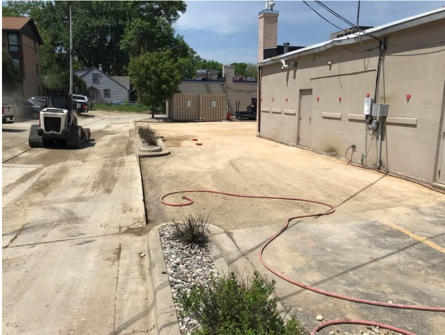
Photo 13: Looking west at base course material from west side of excavation area on May 24, 2018.
