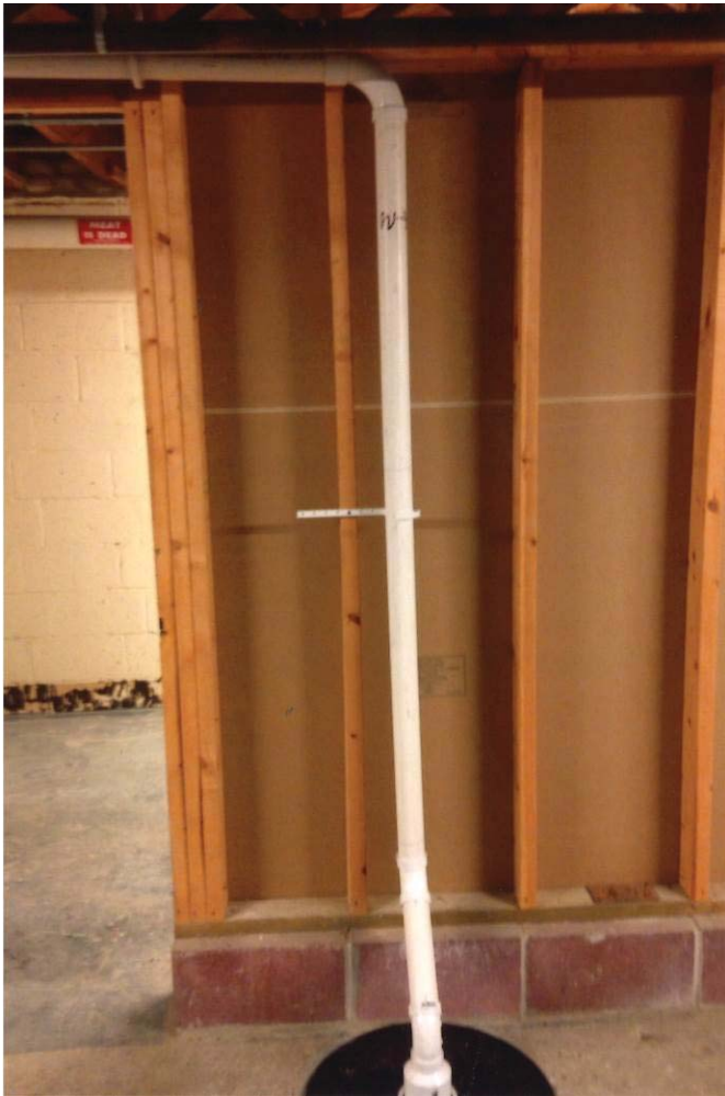
Photo 5: View looking west at mitigation system Pickup Point #4 (PU-4) in basement of 2803-2807 University Avenue.
