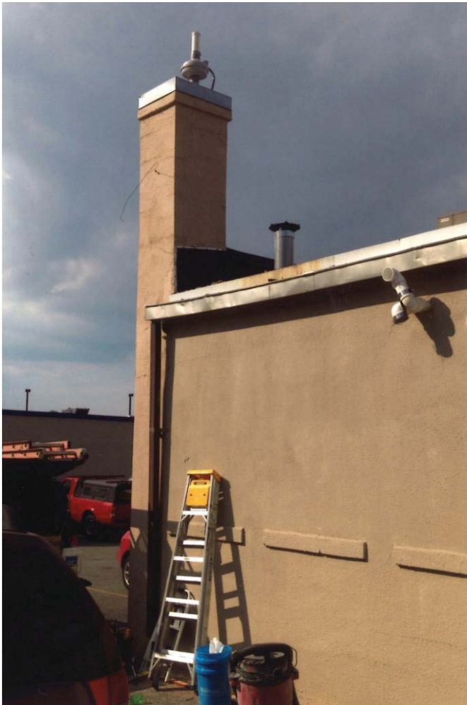
Photo 1: View looking northwest at southwest corner of 2803-2807 University Avenue building showing mitigation system fan and exhaust point.
