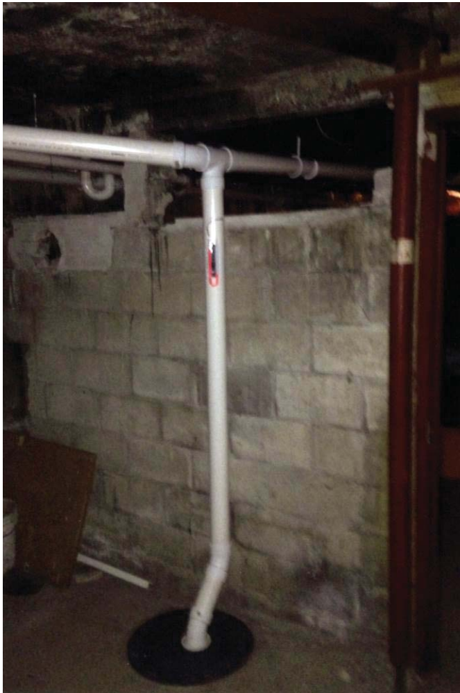
Photo 2: View looking northwest at mitigation system Pickup Point #1 (PU-1) in basement of 2803-2807 University Avenue.
