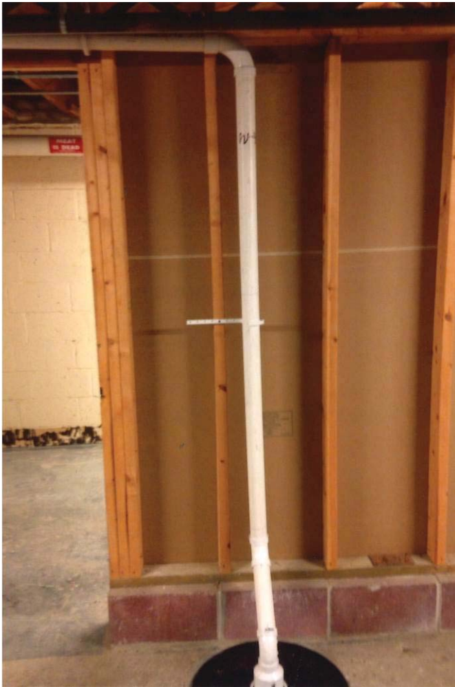
Photo 5: View looking west at mitigation system Pickup Point #4 (PU-4) in basement of 2803-2807 University Avenue.
