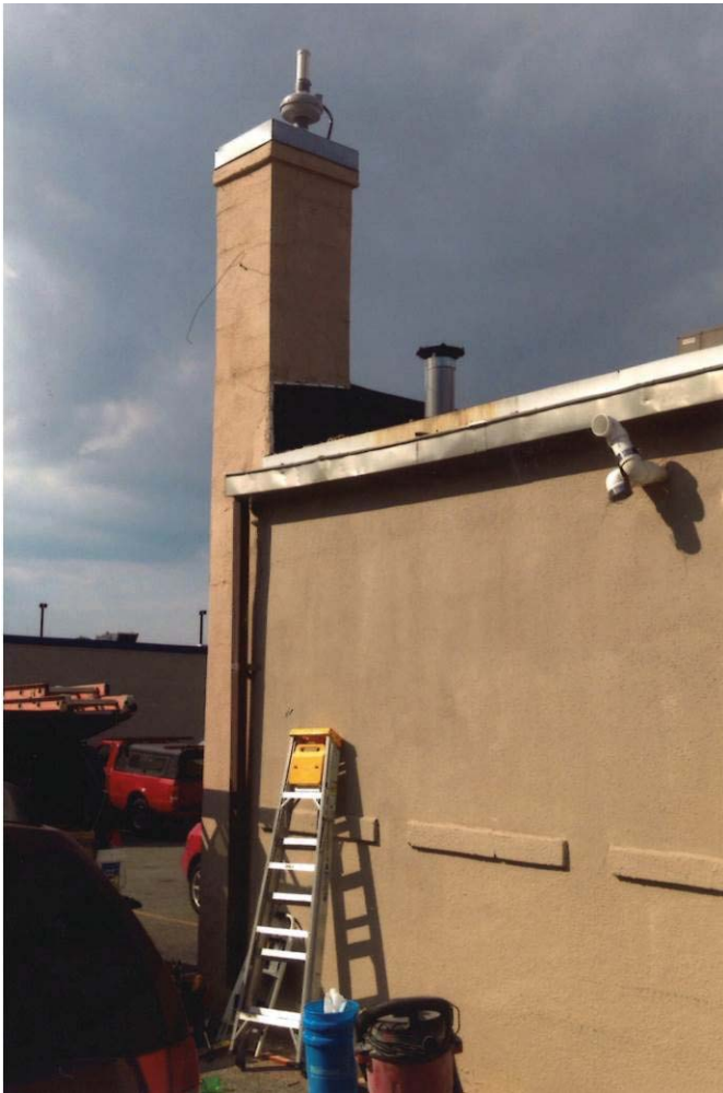
Photo 1: View looking northwest at southwest corner of 2803-2807 University Avenue building showing mitigation system fan and exhaust point.
