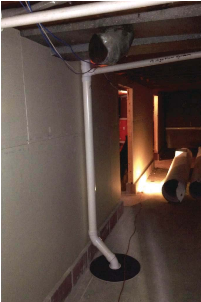
Photo 4: View looking northwest at mitigation system Pickup Point #3 (PU-3) in basement of 2803-2807 University Avenue.
