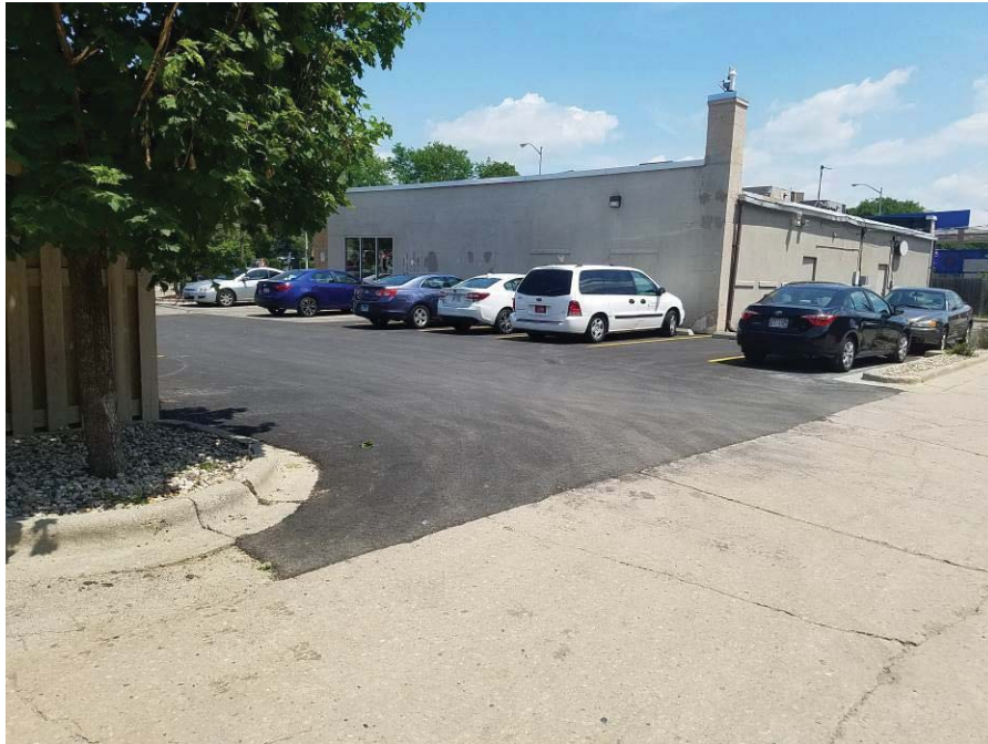
Photo 3: Looking northeast at pavement from south side of the property on June 7, 2018.
