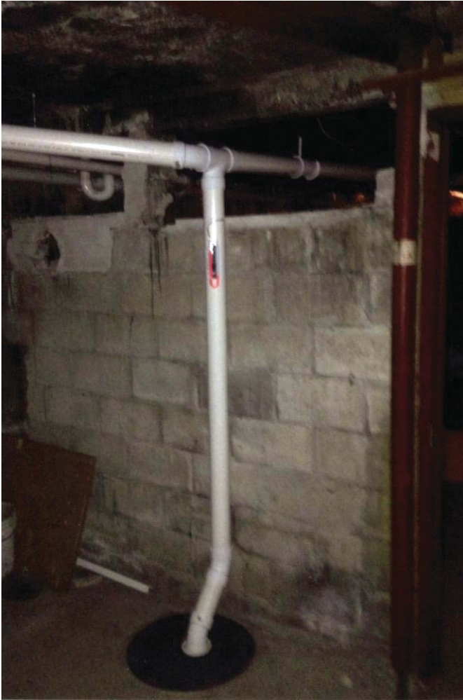
Photo 2: View looking northwest at mitigation system Pickup Point #1 (PU-1) in basement of 2803-2807 University Avenue.
