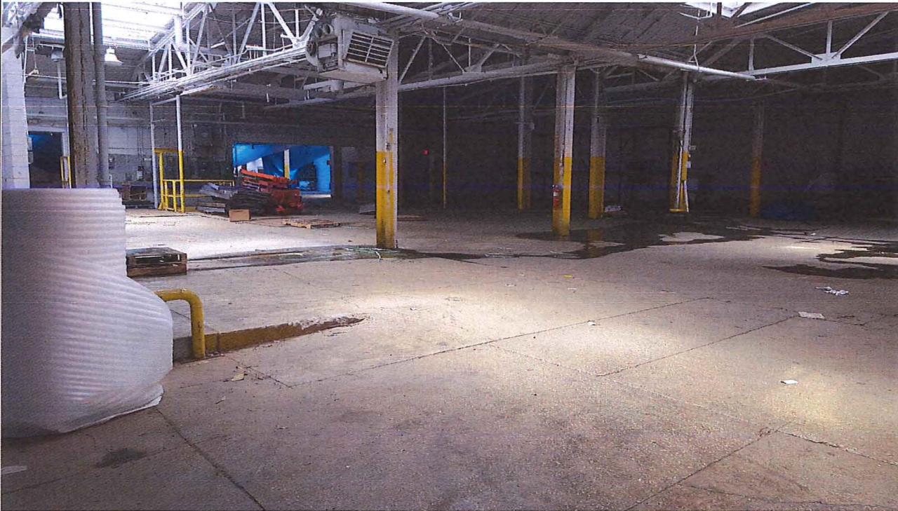
Title: Main Parcel (North Half, NE Corner), Facing SW (7/10/2017) - Findley Adhesives Property, BRRTS #: 03-41-005301
