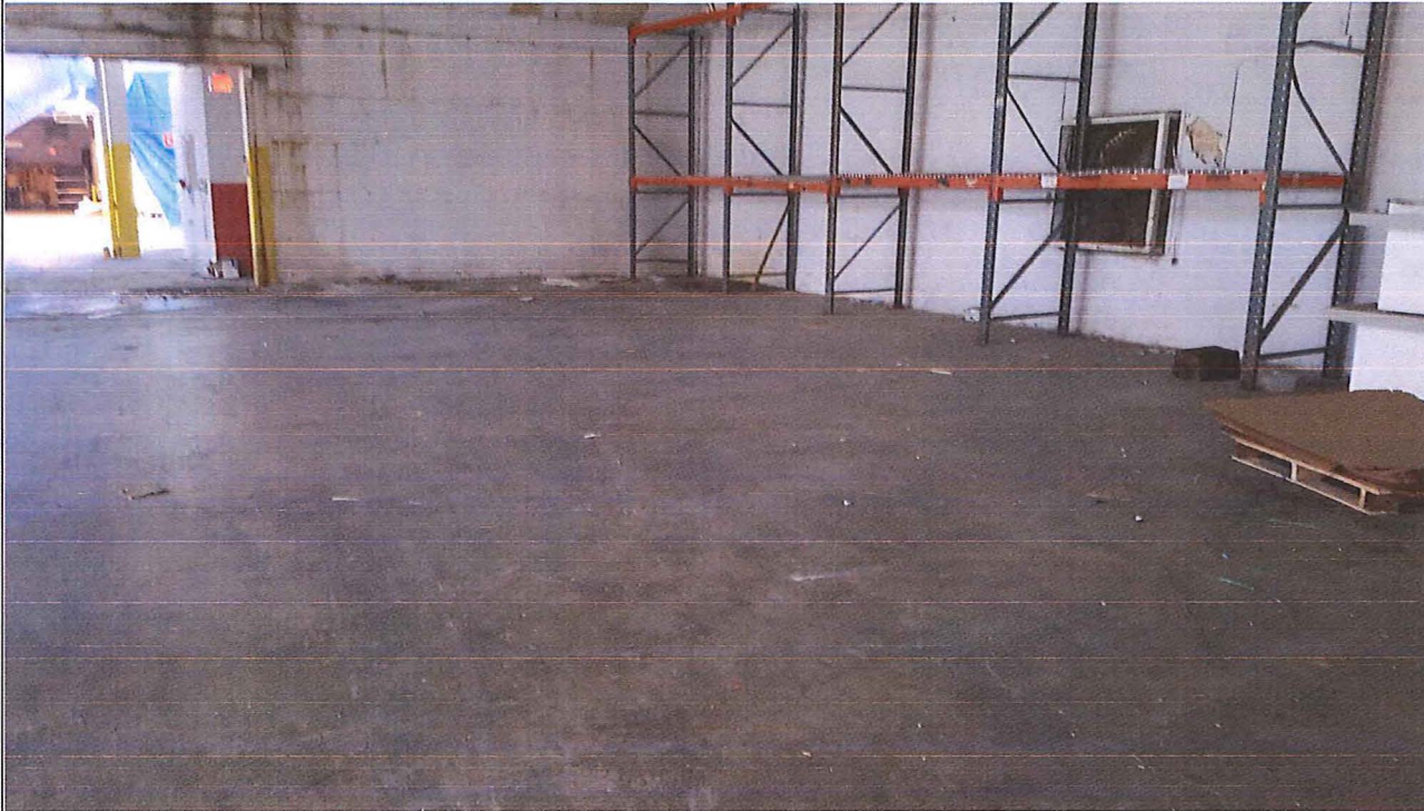
Title: Main Parcel (North Half, Center), Facing S (7/10/2017) - Findley Adhesives Property, BRRTS #: 03-41-005301
