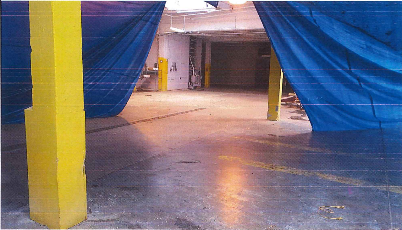
Title: Main Parcel (South Half, Center), Facing S (7/10/2017) - Findley Adhesives Property, BRRTS #: 03-41-005301
