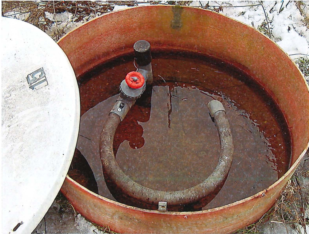
Interior of Fiberglass Cover Assembly 11/29/10
