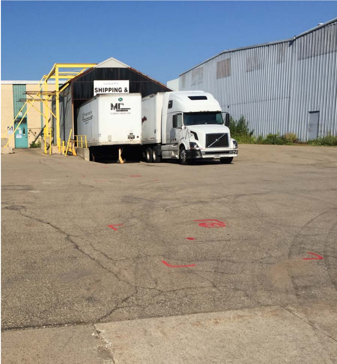
View of the asphalt driveway area north of the warehouse, facing northwest.
