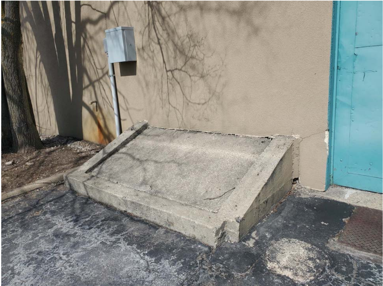
View of a concrete surface feature near the southeast corner of the warehouse, facing northwest.
