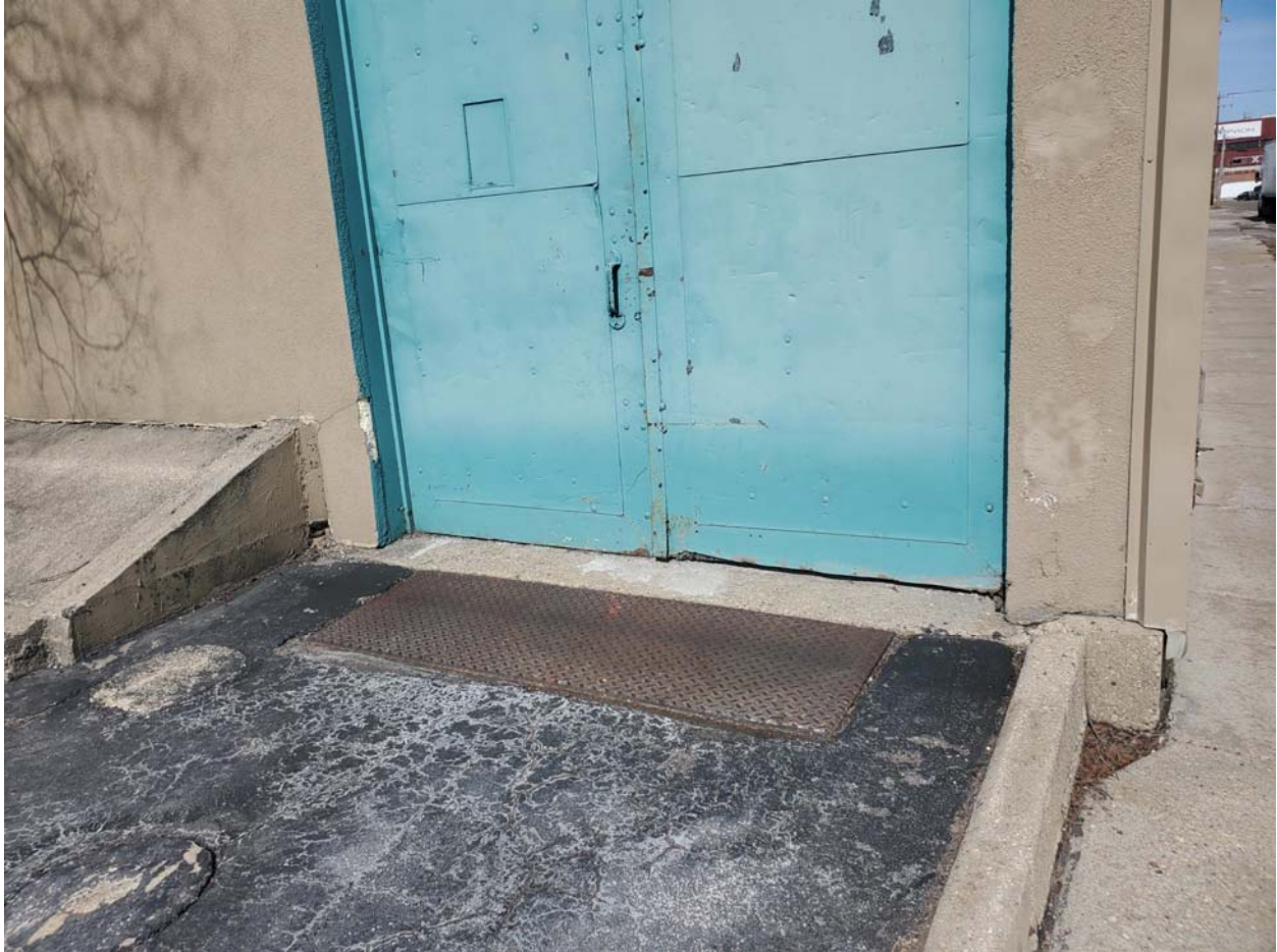
View of the asphalt driveway area outside the southeast corner of the warehouse, facing north.
