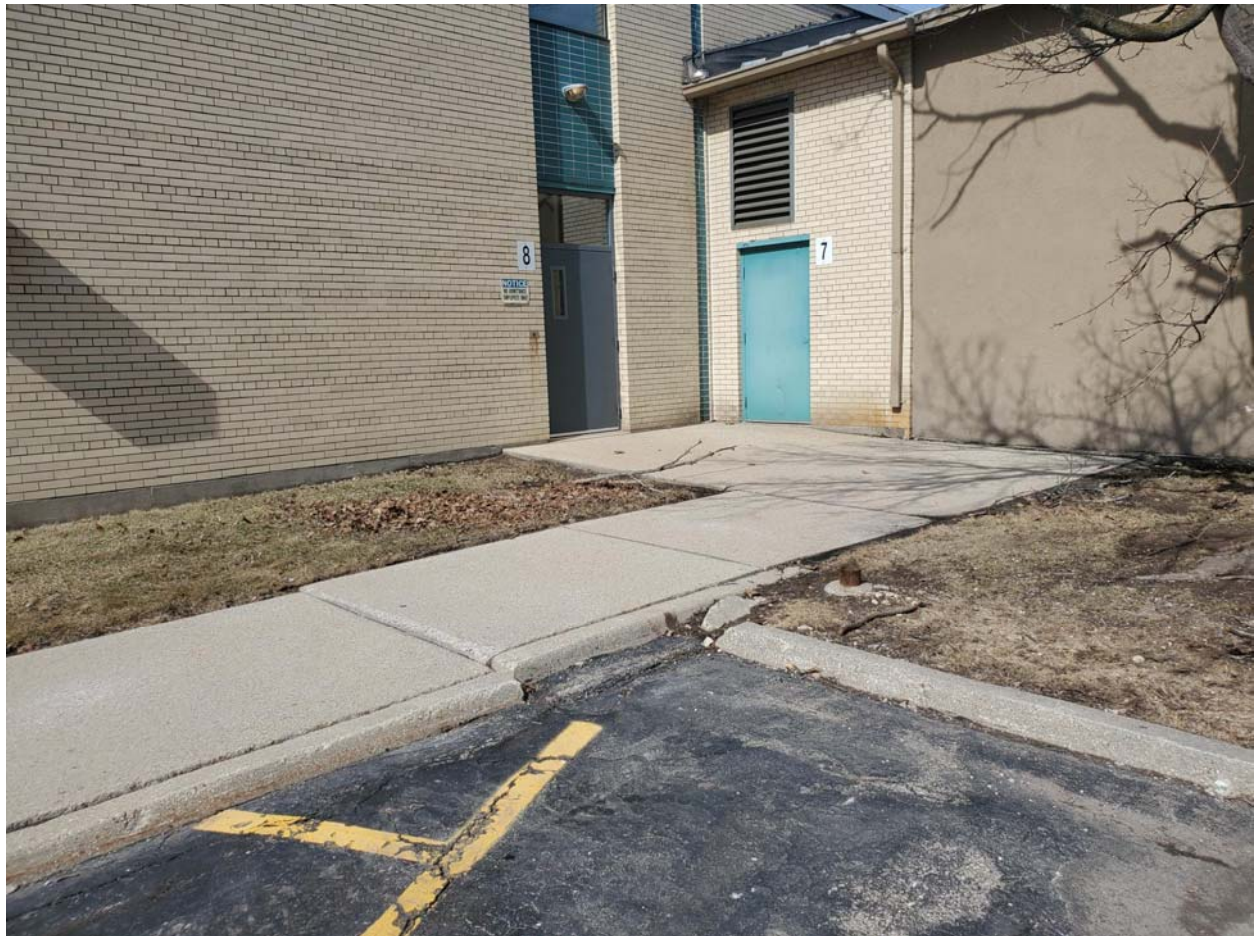
View of grass and concrete portions of the cap outside the southwest corner of the warehouse, facing northwest. The asphalt in the photo is on the 714 Hancock Street parcel.
