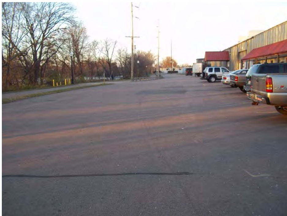
Photo 3 – Parking and access area west of Wausau Chemical. Looking north. Crack repair in foreground.
