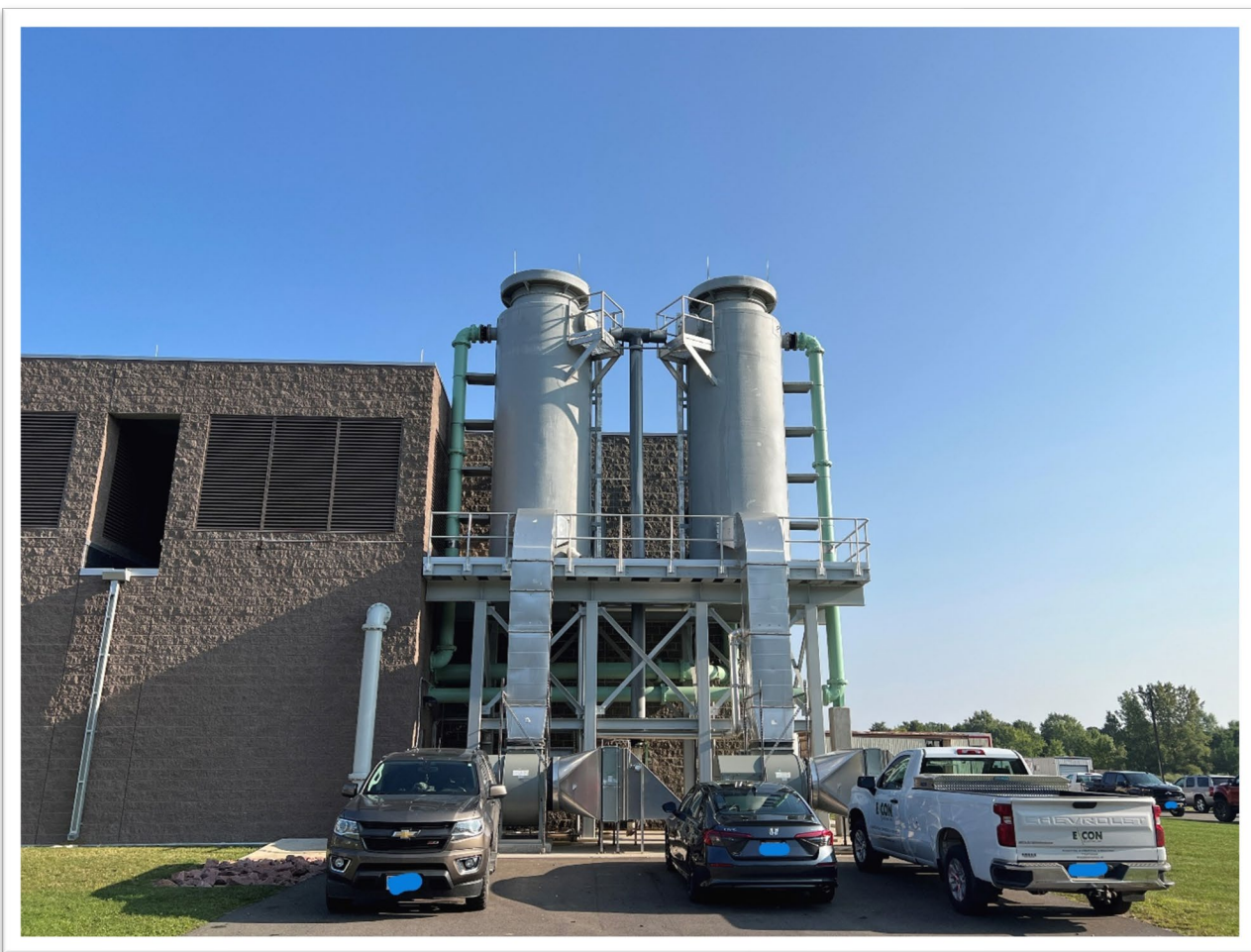
Image 7: Air strippers used at Wausau Water Works to remove VOCs from water
