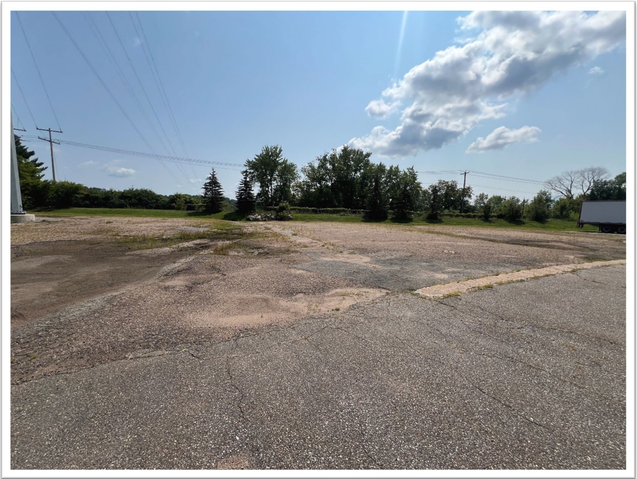
Image 2: Area on West Bank with improperly maintained cap/asphalt barrier
