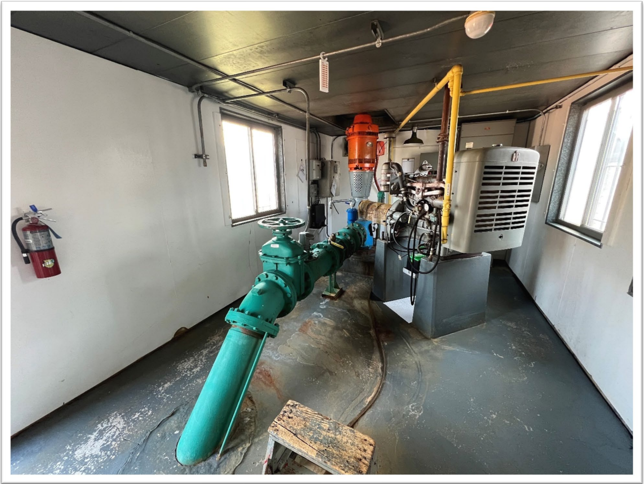
Image 9: View inside of pump house for City Well 3 (CW3)
