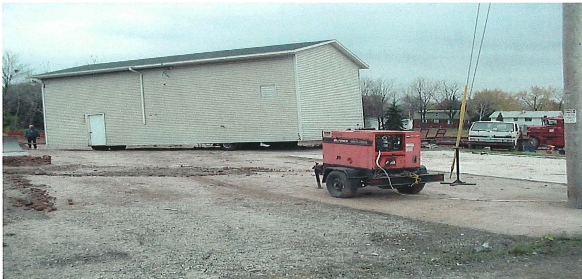
Treatment building moved off foundation at Chrome Shop
