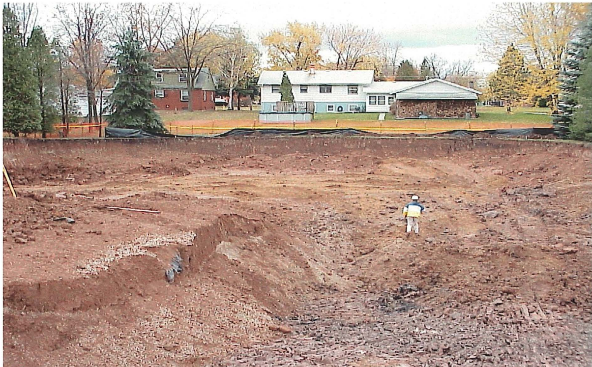
Chrome Shop excavation nearing completion. Quadrants 1, 2, and 3 partially backfilled. Quadrant 4 excavated to depth. Gravel sump area installed by the EPA in the early 1990s visible on left.
