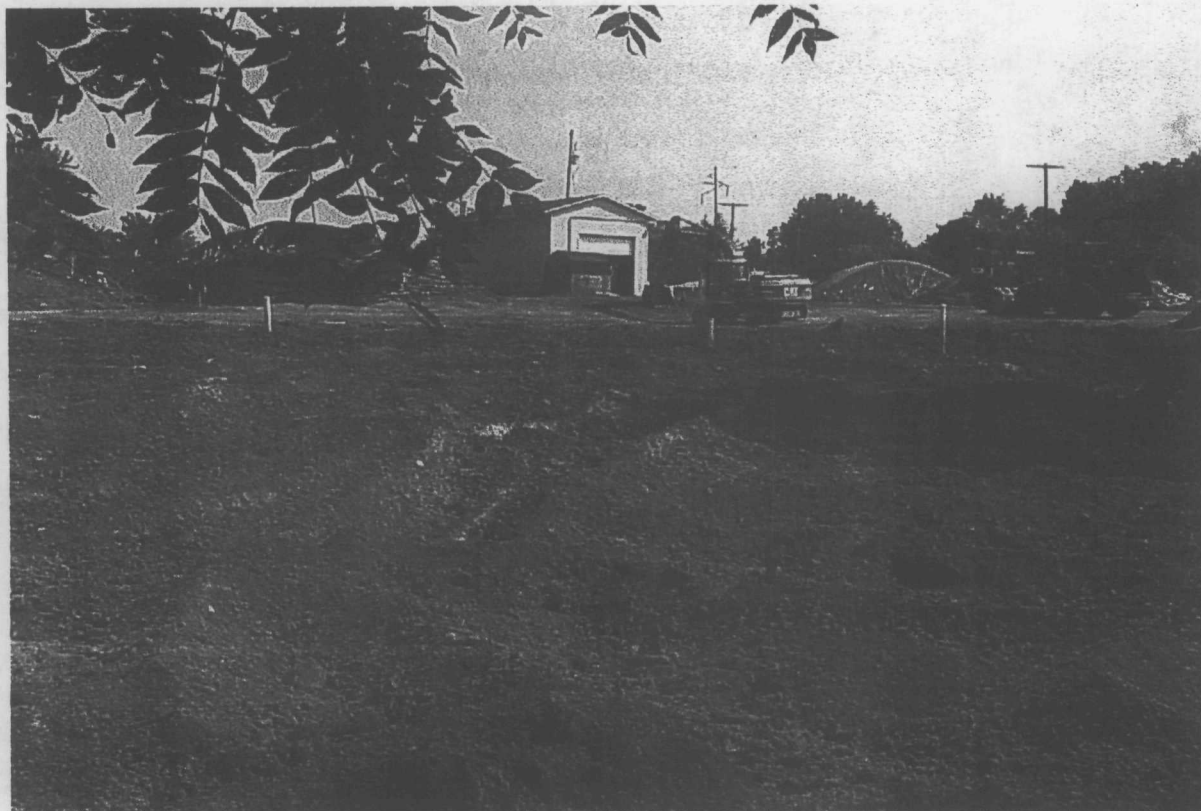
Excavated area at Chrome Shop looking northeast from southwest property corner. Treated soil in foreground (Quad. 2) prior to stockpiling.
