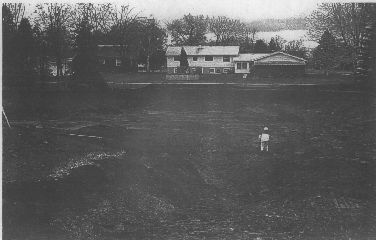
Chrome Shop excavation nearing completion. Quadrants 1, 2, and 3 partially backfilled. Quadrant 4 excavated to depth. Gravel sump area installed by the EPA in the early 1990s visible on left.
