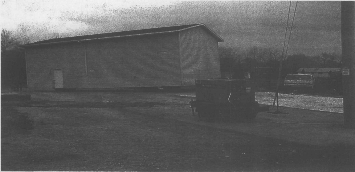
Treatment building moved off foundation at Chrome Shop
