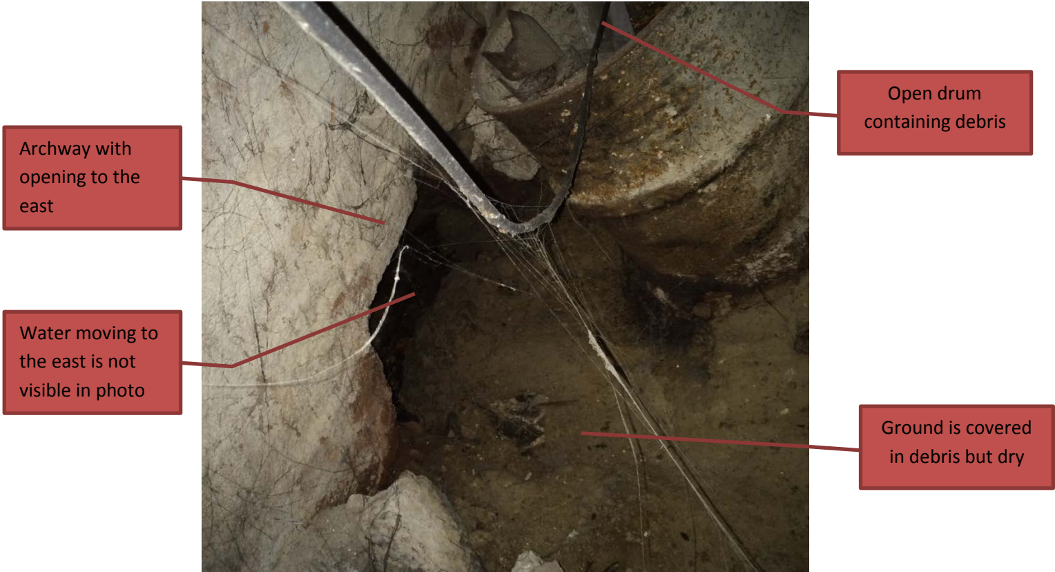
Photo 7. Looking southeast through the dry wall of the boiler room at the archway through the east wall of the boiler room.
