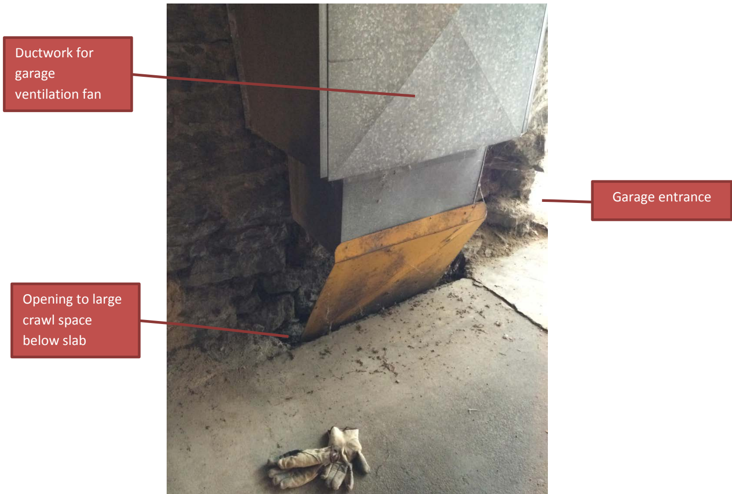
Photo 5. Access to large crawl space through garage floor just south of garage entrance.
