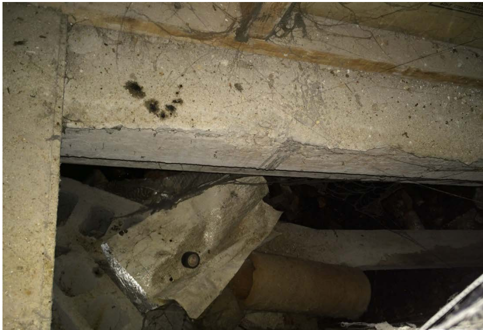
Photo 4. Looking down into large crawlspace, standing water is present below the debris.
