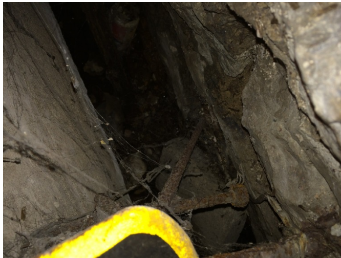
Photo 6. Looking into the opening between the slab and the building wall south of the garage entrance.
