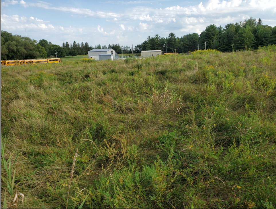
Title: Neillsville Foundry, 02-10-000048, 08/21/2020. Photo taken from northwest edge of cap. Facing northeast. Cap in good condition.
