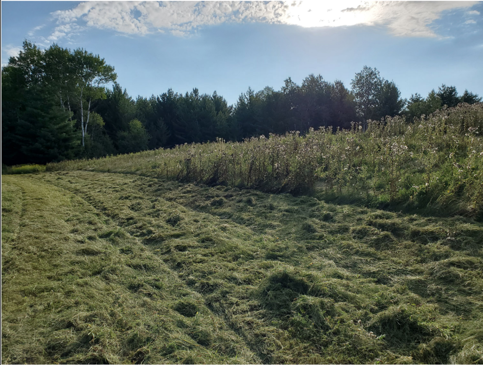
Title: Neillsville Foundry, 02-10-000048, 08/21/2020. Photo taken at the northern edge of cap. Facing directly west-southwest. Cap in good condition.
