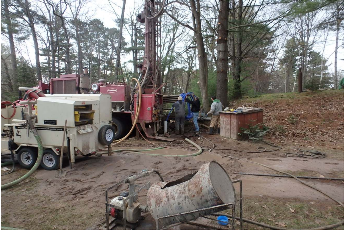
Photo 5 – Installing development pump after installation of filter pack using tremie pipe and mixing barrel.
