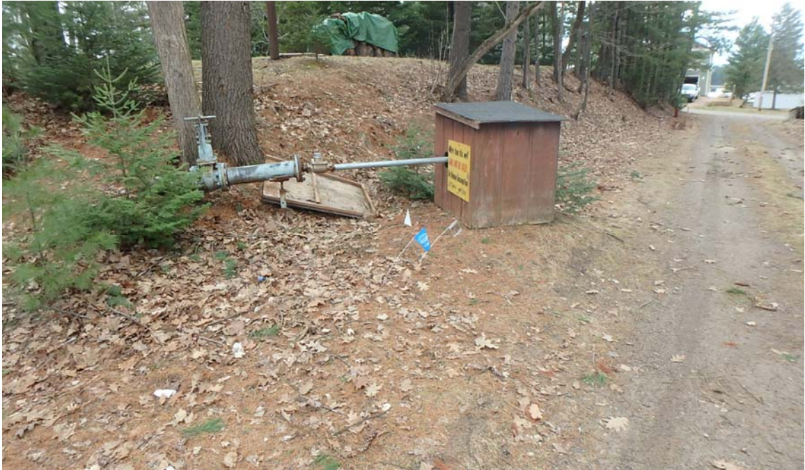
Photo 1 – Failed well EXW-4 in doghouse on April 14, 2017 prior to replacement. Pine Street in photo right.
