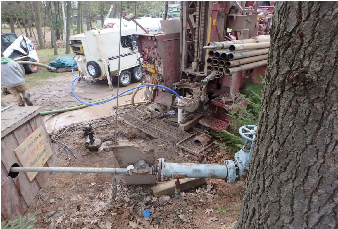
Photo 6 – Developing new well with submersible pumping, old well header pipe and flowmeter in foreground.
