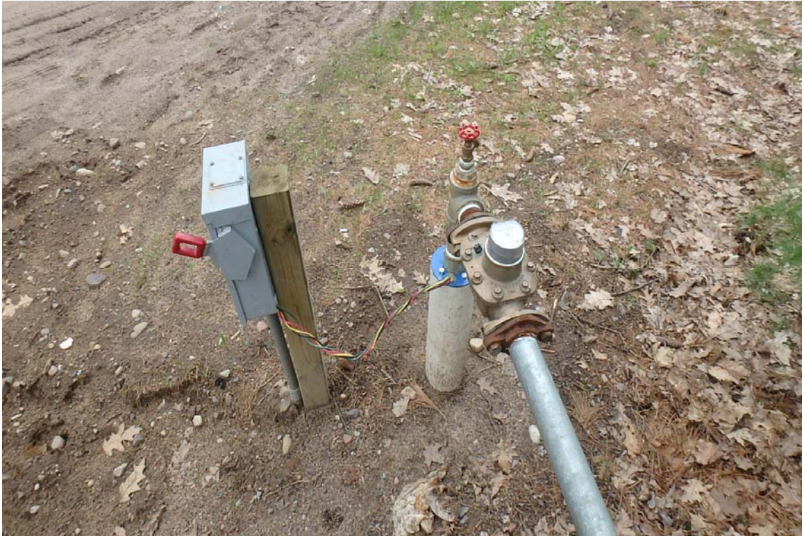
Photo 10 – New well EXW-4 with flowmeter and electrical service prior to placing doghouse over well.
