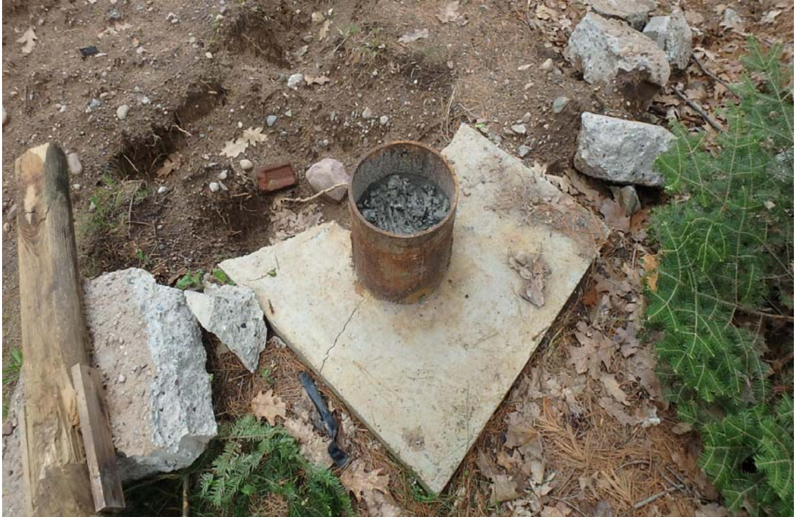
Photo 9 – Abandoned failed well EXW-4 with bentonite chips prior to well stickup being cutoff.
