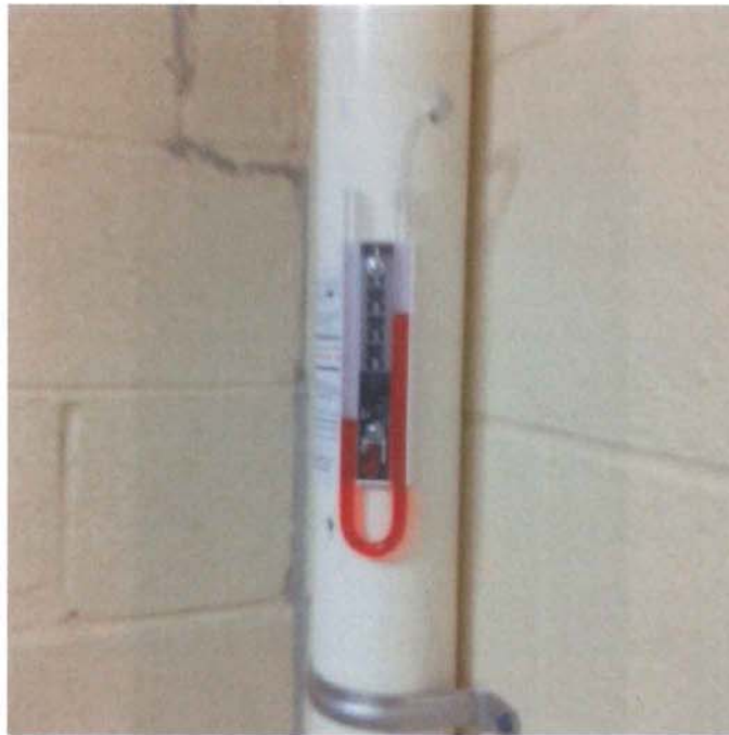
Photo 9: Manometer installed on pickup point #3 in main building. Note caulking on crack to the left of the pipe. Smoke detected leaks in the crack.
