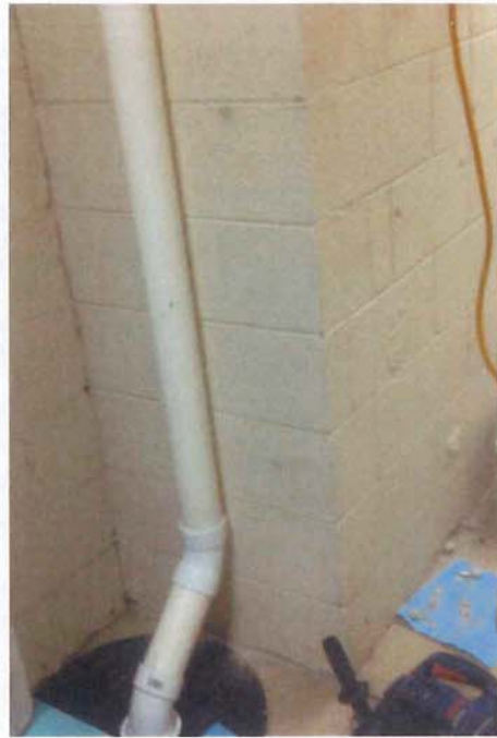
Photo 11: Hole/pickup point #3 in hall of storage area of main building (beside crack/joint).
