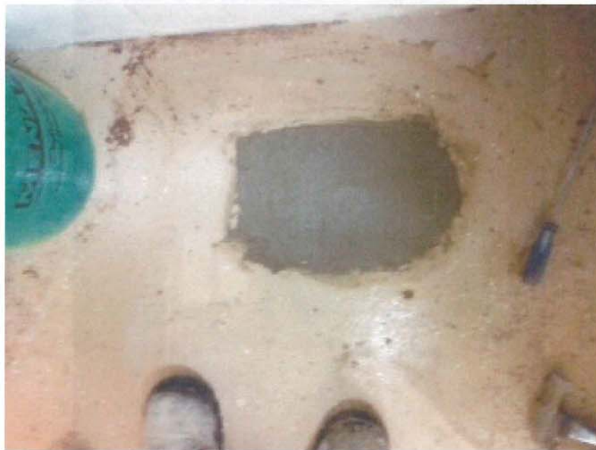
Photo 10: Failed pickup point #3; concrete tank underneath. Resealed with concrete (hole #3 moved).
