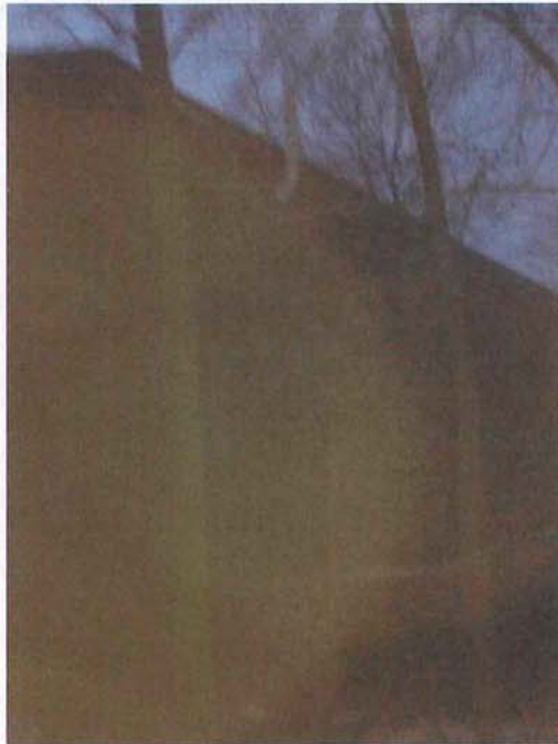
Photo 7: Discharge piping – system #2.
