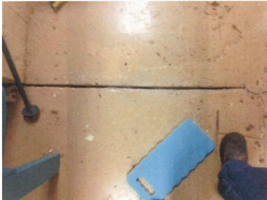
Photo 16: One-half-inch crack/joint in locker/storage area of main building. Crack later sealed where exposed.
