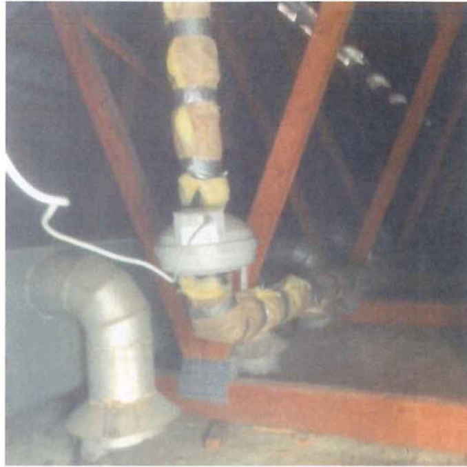
Photo 1: Prowler fan and connecting piping in attic space. System #1, main building.
