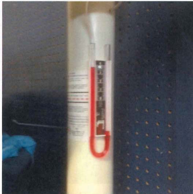
Photo 4: Manometer on system #2, garage.
