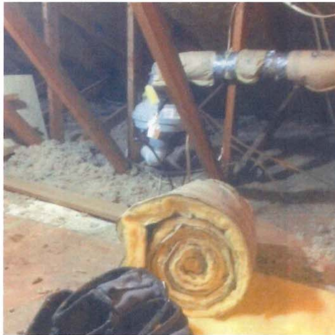
Photo 6: Eagle fan in attic above garage – system #2.
