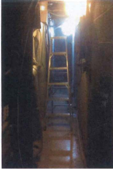
Photo 13: Maintenance access behind dryers in main building.
