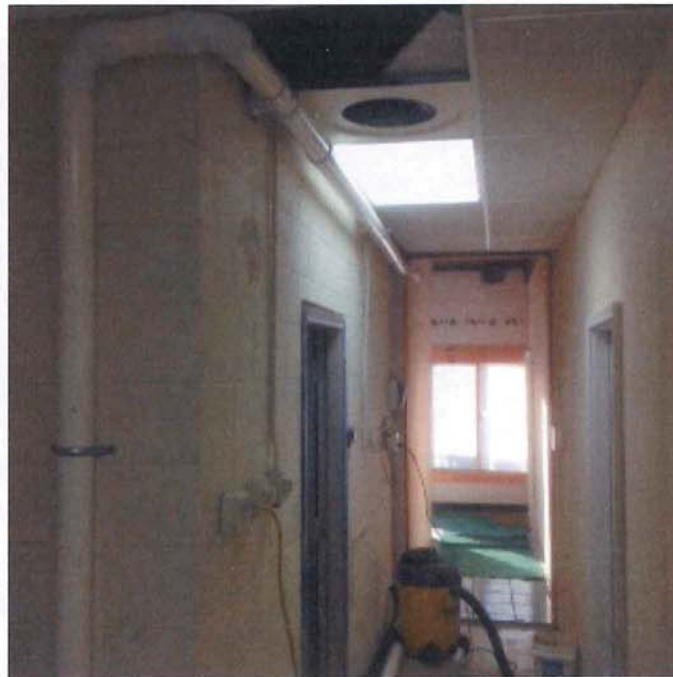
Photo 12: Piping connecting pickup points #2 and #3 in main building.
