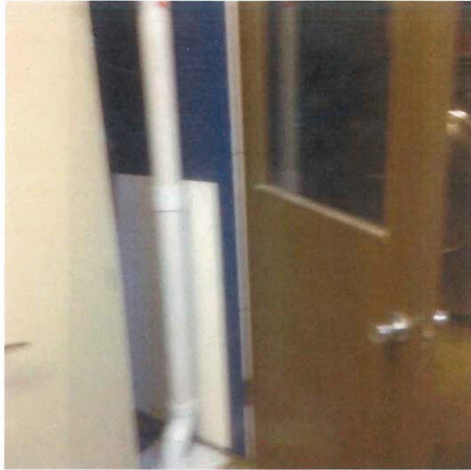
Photo 5: Pickup location in garage – system #2. CT 11/21/14
