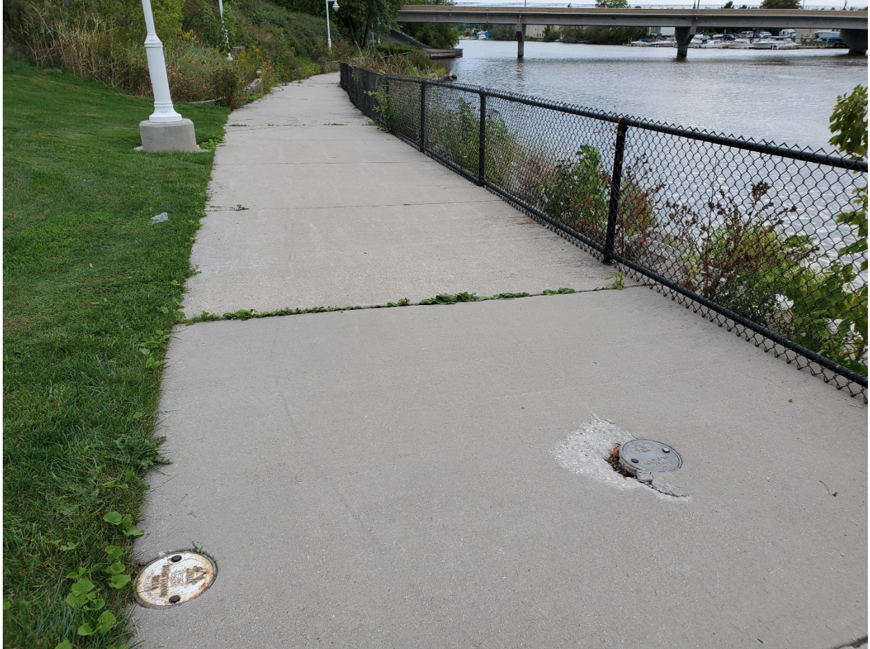
Photo 8: Likely MW-707R (left) and PZ-703 (right) showing damage to surface pavement. Photo looking southeast from near the southeast end of the site taken September 21, 2022.
