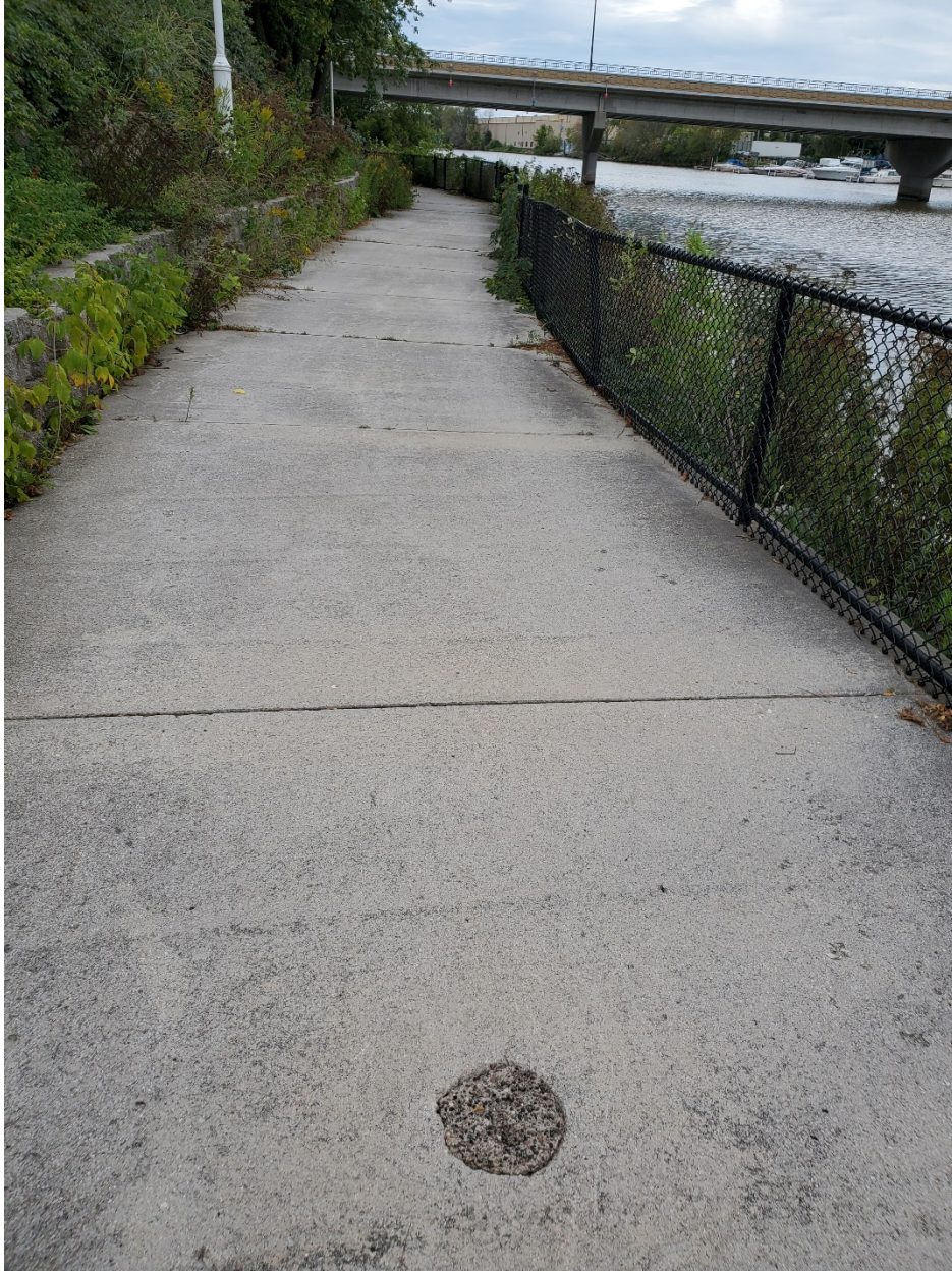
Photo 10: Possible abandoned boring/geotechnical boring at the extreme southeast end of the site near retaining wall (left side of photo). Looking Southeast, taken September 21, 2022.
