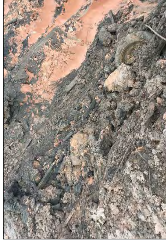
Buried debris and organics in new UST basin
