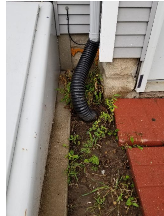
Photo #2 West roof drain. The corrugated connecting tubing was observed to be leaking at the bend.
