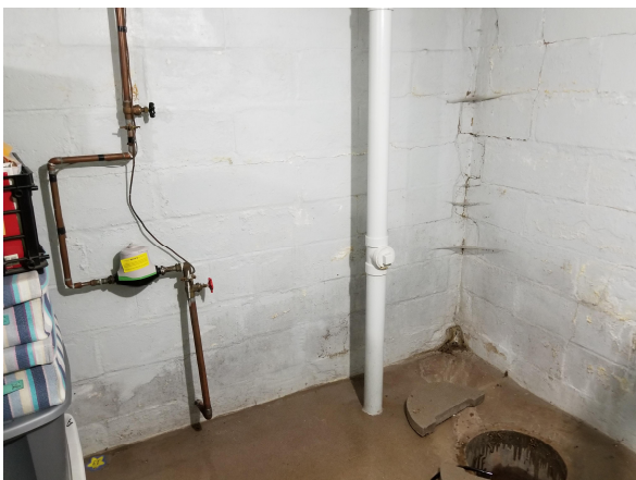
Photo #5 Sump pit, water line, and sanitary sewer line in the southeast corner of the basement.
