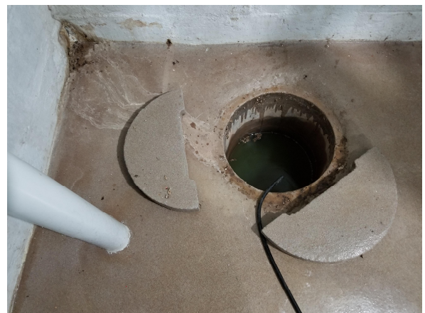
Photo #6 Sump pit with standing water above the discharge pipe.
