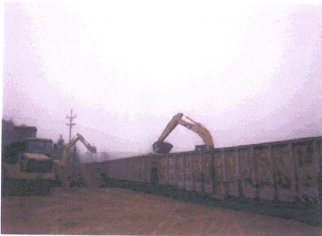
Photo 5: Excavated soil was transported off-site via the railroad to a solid waste landfill.
