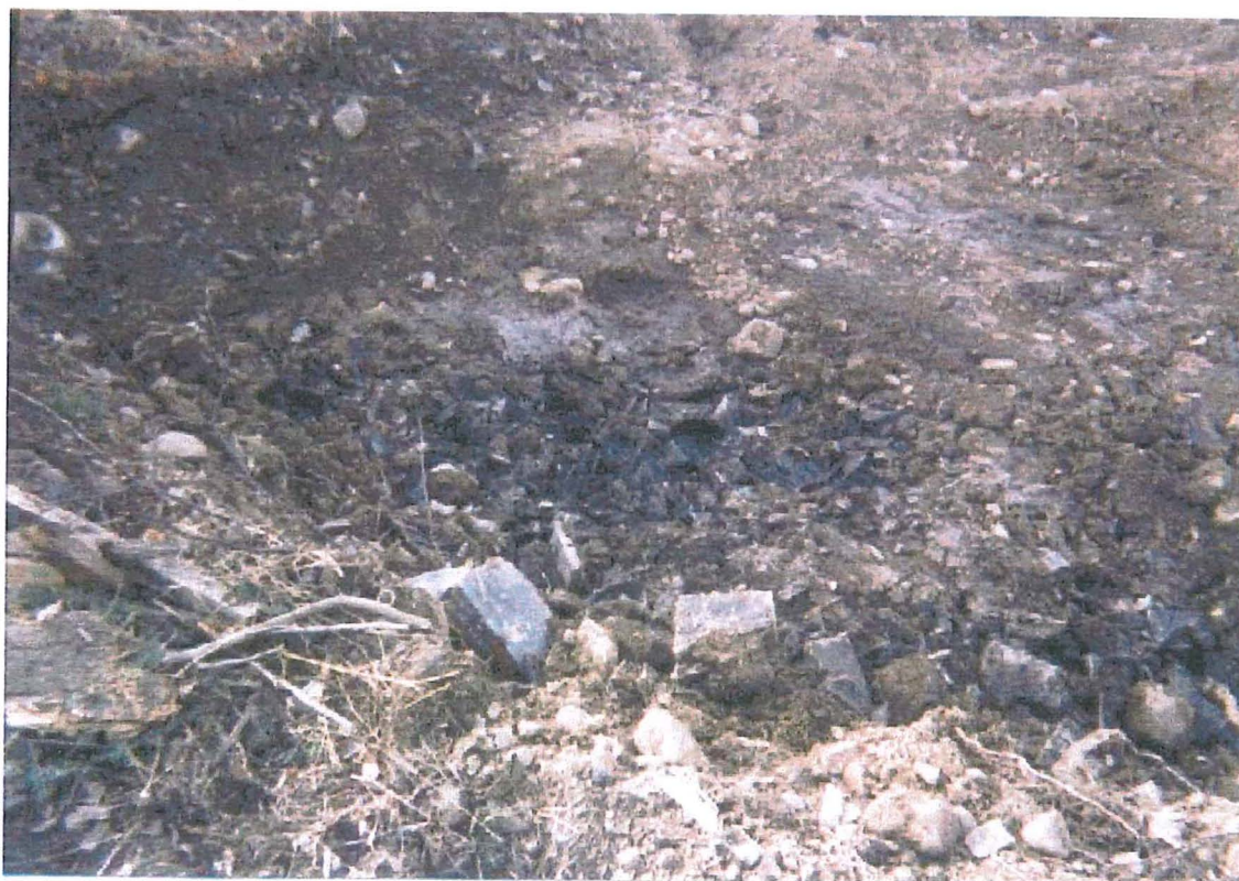
Photo 6: Buried battery casings were discovered on-site during excavation activities. Battery casings were stabilized and disposed of with excavated soil.
