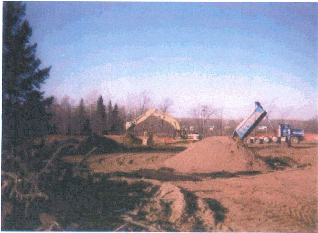
Photo 7: Excavated areas were backfilled with clean general fill from an off-site borrow source.
