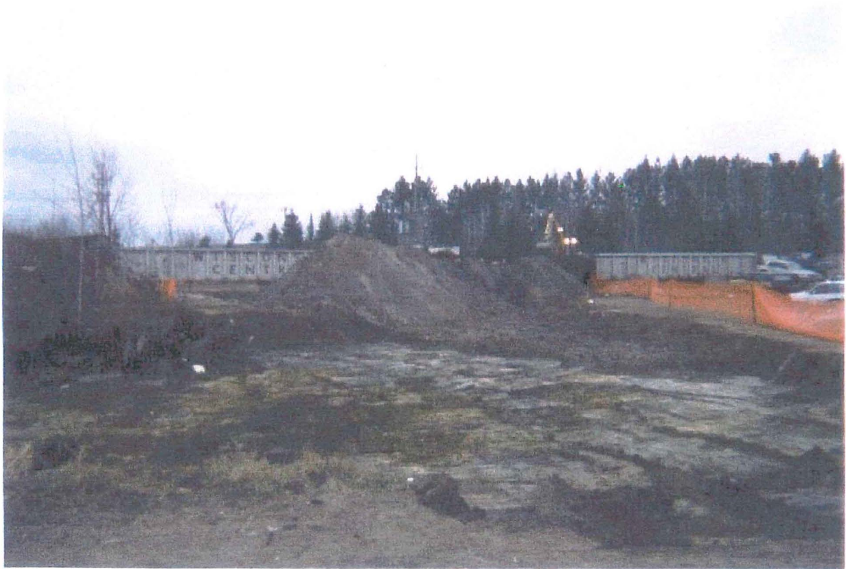
Photo 4: Soil above the TCLP lead limit of 5 mg/L was stabilized in-situ, stockpiled, and sampled prior to being disposed of off-site.
