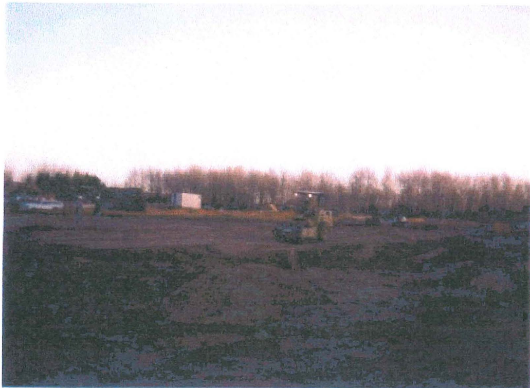
Photo 8: All backfilled areas were compacted and tested to meet the site compaction criteria.
