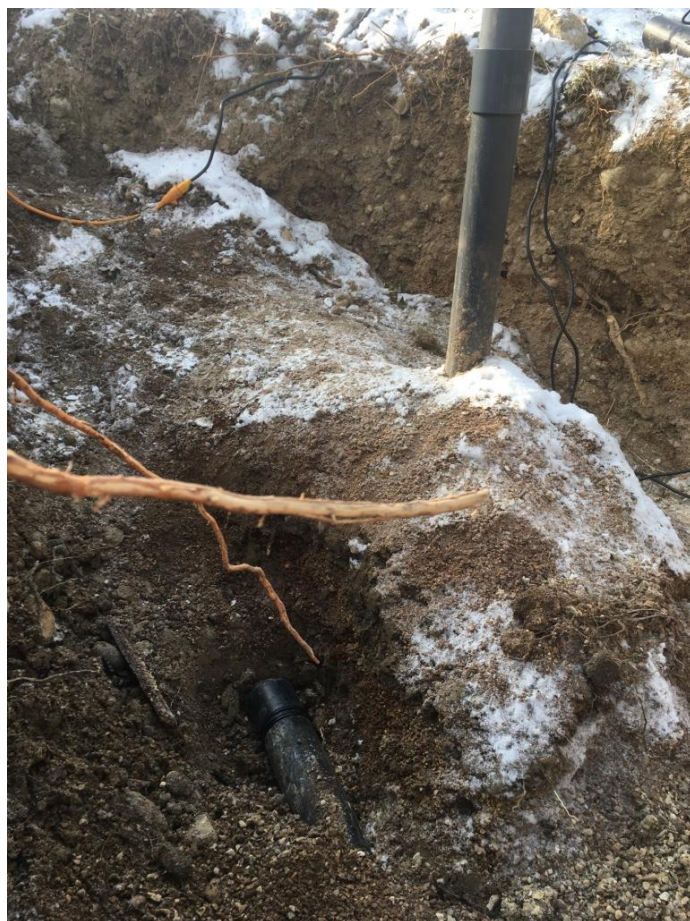
12/11/17 Stationing 5+38 at gas well EW-20. Existing 3 inch diameter lateral terminated and capped with HDPE butt fusion weld, looking southwest.
