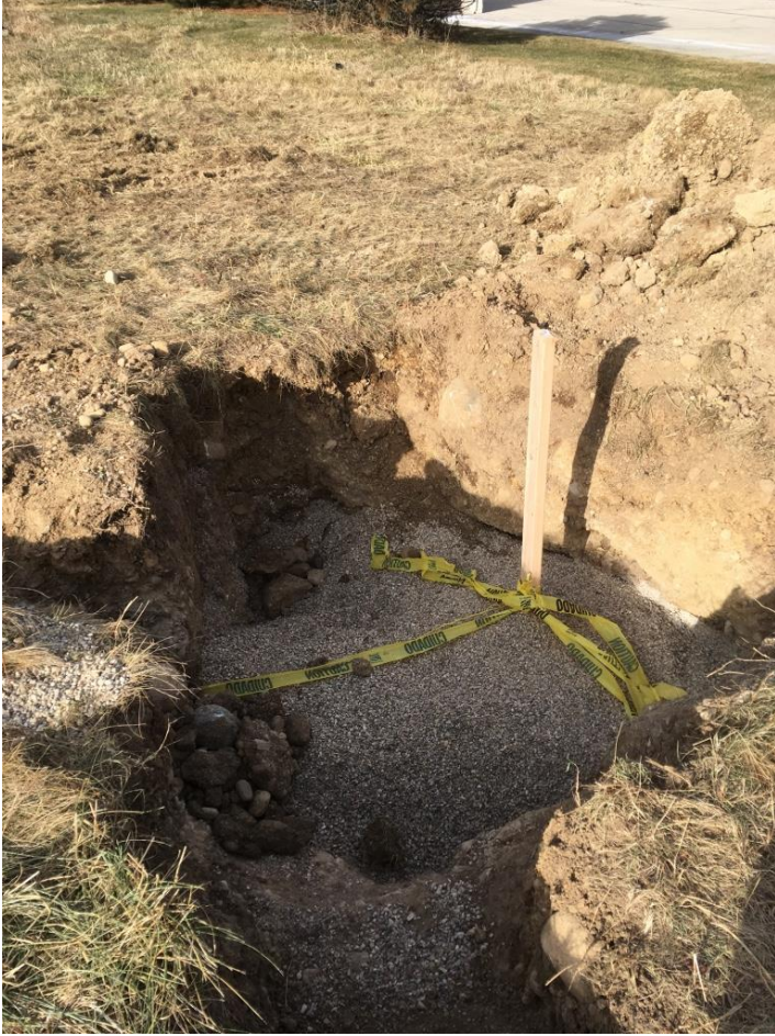
12/7/17 Stationing 0+00, Wood 2x4 marking location, pea gravel back fill, warning ribbon and electrical tracer wire in place, just prior to soil backfilling.
