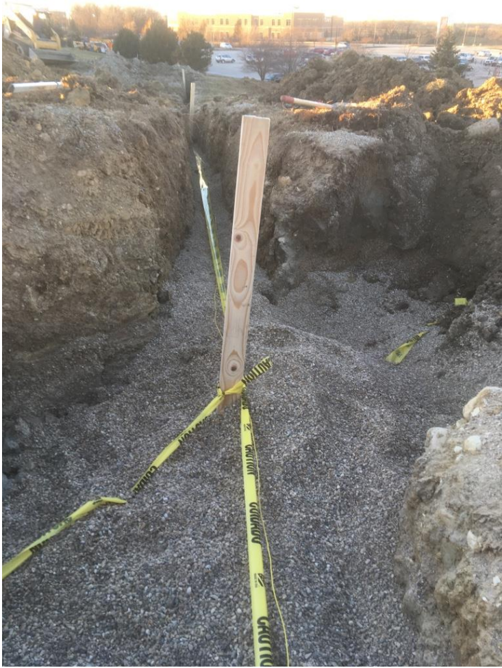
12/7/17 Stationing 2+56, pea gravel backfill, caution tape and electrical tracing wire in place just prior to soil backfill.
