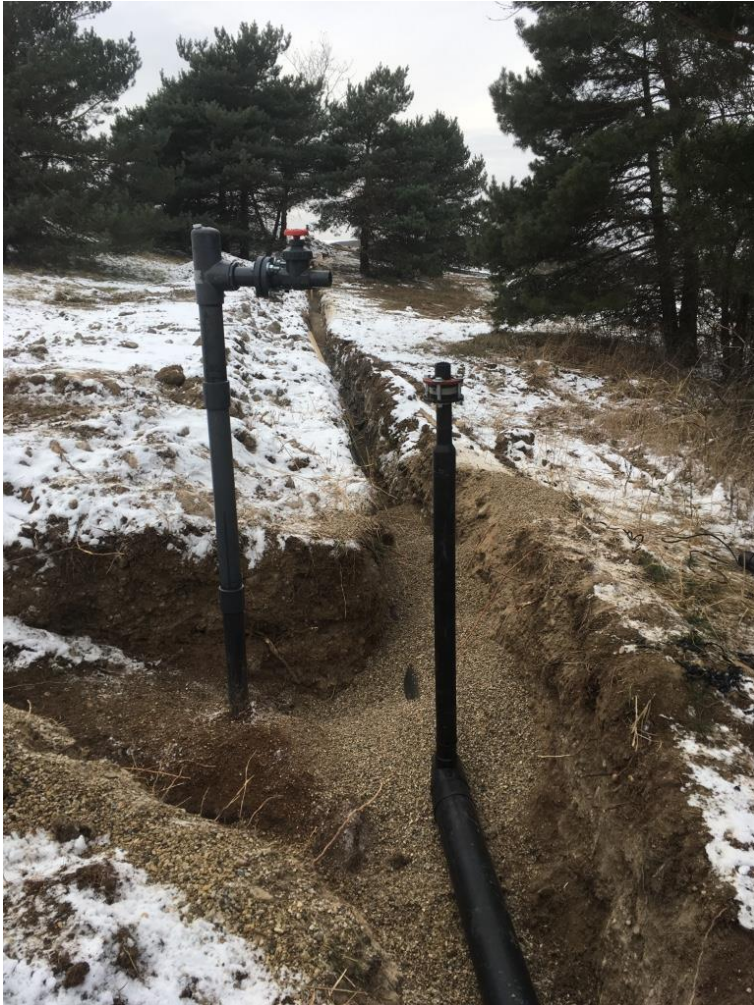
12/11/17 stationing 5+38, 2x6 tee, with 2 inch diameter vertical riser at EW-20, looking west.
