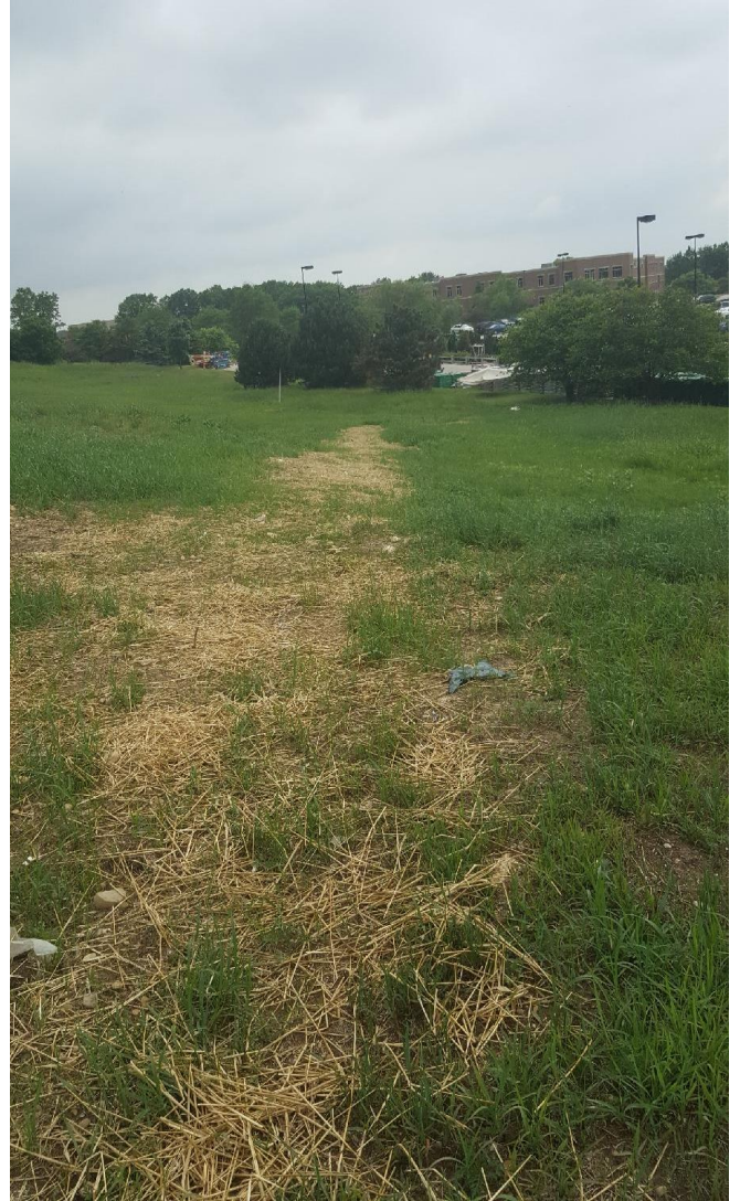
June 7, 2018 re-seeded, fertilized and straw mulch by- pass trench, near station 3+00, looking northwest
