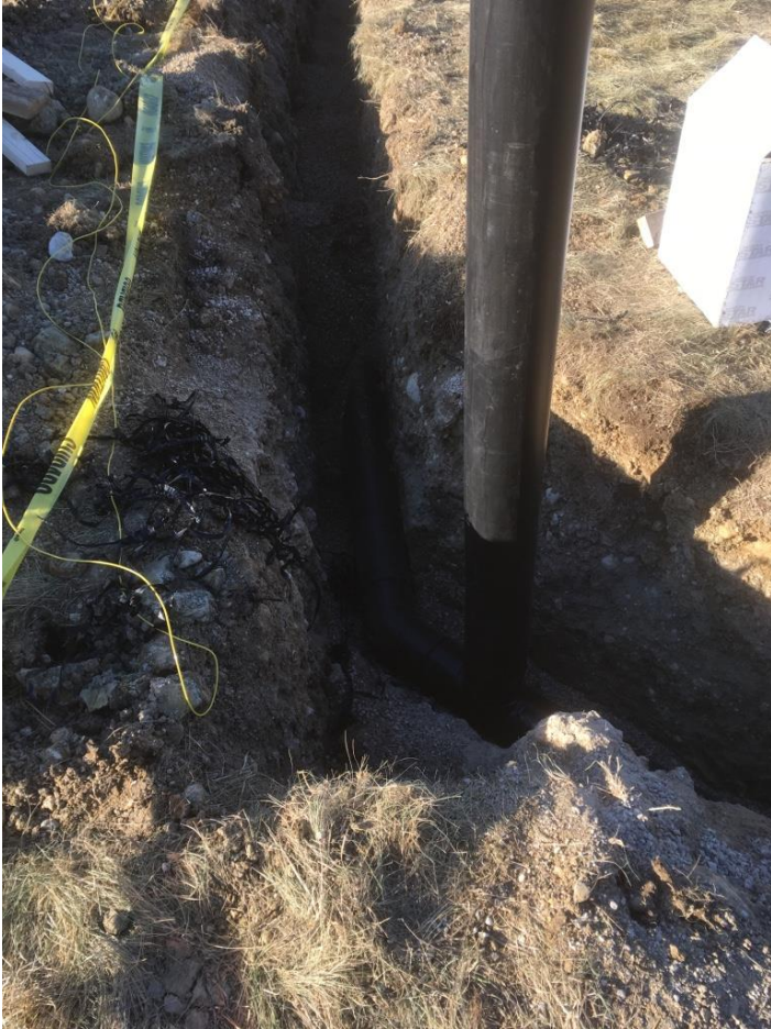
12/8/17 Stationing 2+98, 33 degree bend and vertical standpipe at high point.
