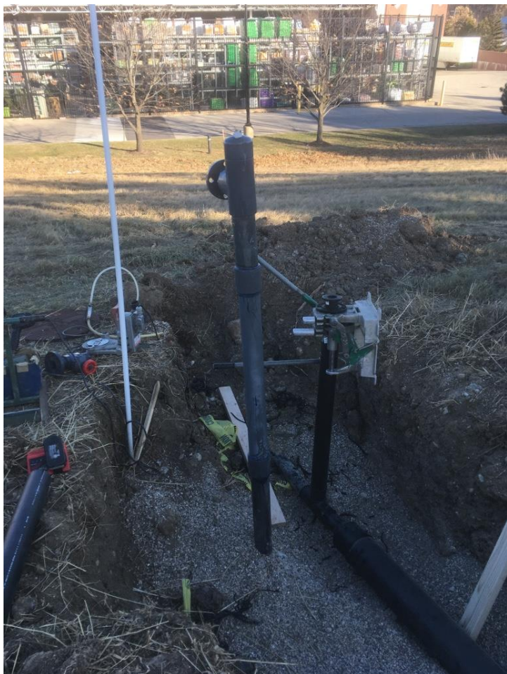
12/11/17 Gas well EW-19, 6 inch lateral connected to existing 3 inch lateral and vertical 3 inch riser, looking north.
