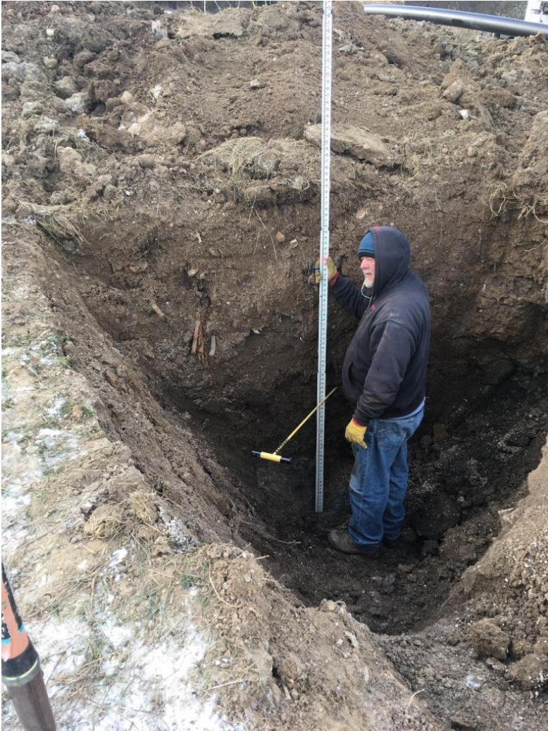
12/12/17 Stationing 7+58, Proposed by-pass header pipe connection to existing 6 inch diameter header pipe, trench excavation approximately 8 feet below grade, looking southwest.
