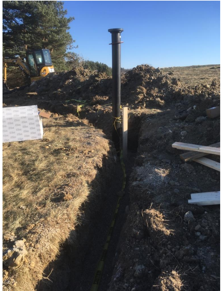
12/8/17 Stationing 2+98, 33 degree bend and standpipe. Pea gravel backfill, wood 2x4, warning ribbon and electrical tracer wire.
