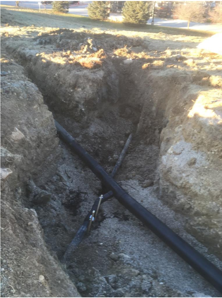
12/7/17 Stationing 2+56, Existing 3 inch diameter lateral to gas well G-2, connected to 6 inch by-pass header. Two 3x6 tees with electro-fusion couplers utilized to make the connection.
