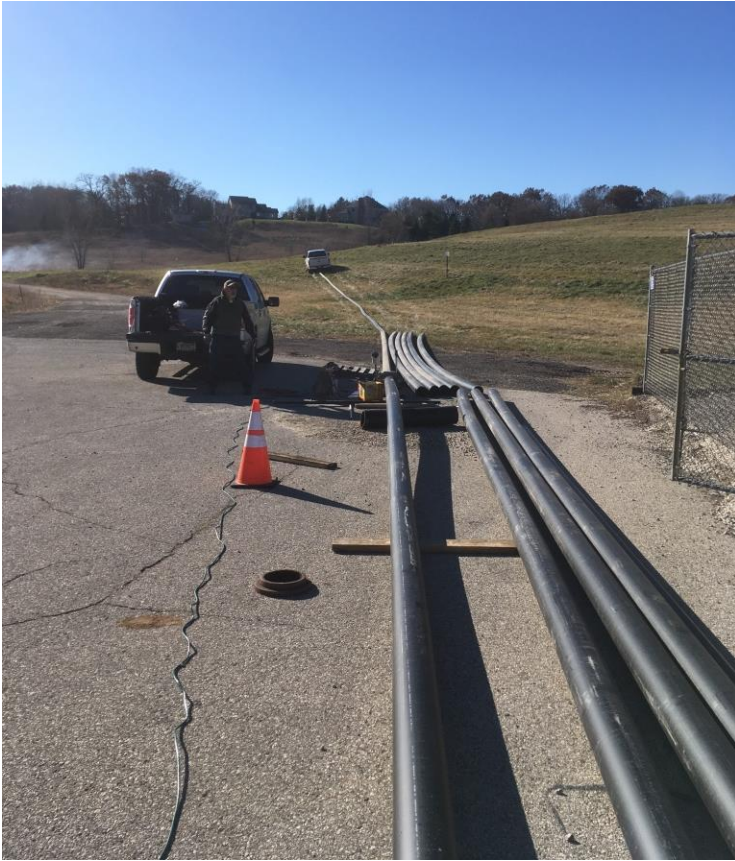
11/29/17 new 6 inch diameter by-pass header pipe, butt fusion welded. 200 to 250 foot lengths pulled into position.
