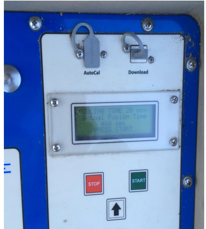
12/6/17 electro-fusion controller used with electro-fusion couplers. Screen indicates timing and successful weld.
