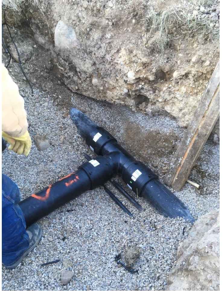
12/6/17 Project Stationing 0+00, exposed existing 6 inch diameter header. 6X6 Tee and new by-pass header installed with three electro-fusion couplers.
