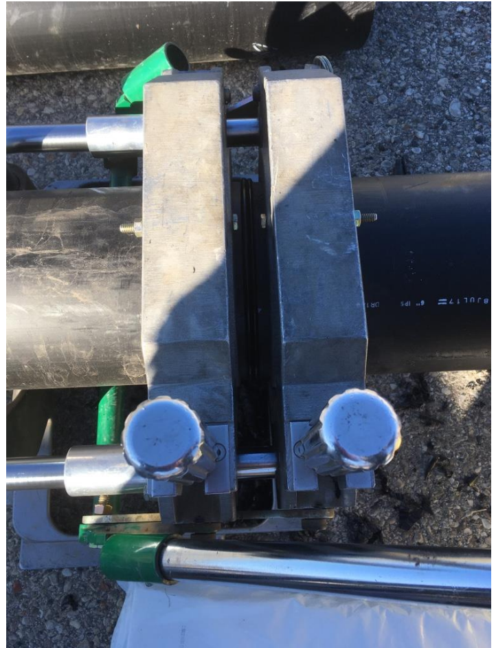
11/29/17 new 6 inch diameter by-pass header pipe, butt fusion welded. Final compression process.
