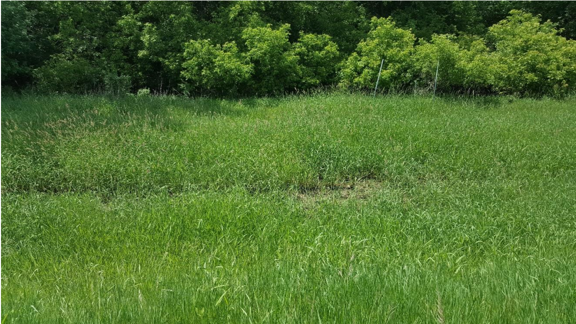
Settlement Area 2 – Located on West Side of Landfill near CS-2 and MP-9. Looking West. Area needs to be surveyed so that drainage can occur.
