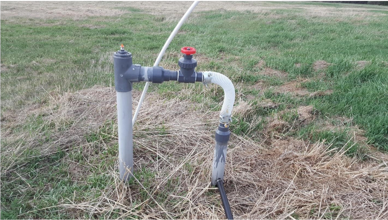
EW-2 Looking West with a temporary 1 ¼" diameter HDPE temporary Jumper Line connected to EW-6.
