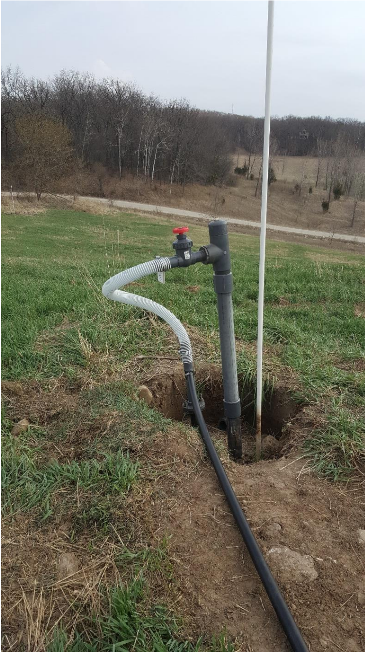
EW-6 Looking North with a temporary 1 1/4" diameter HDPE temporary Jumper Line connected to EW-2.
