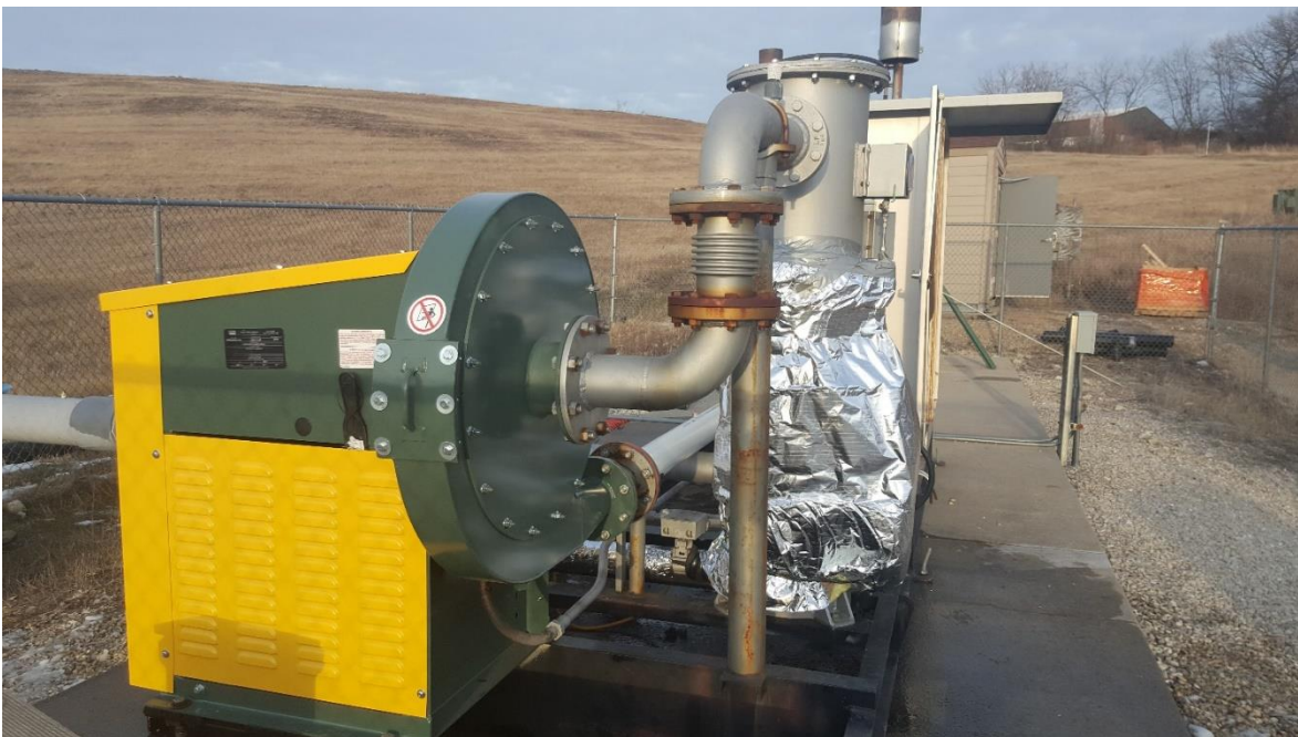
Blower Flare Station – Looking Northeast. The new blower, motor and insulation on the demister tank
