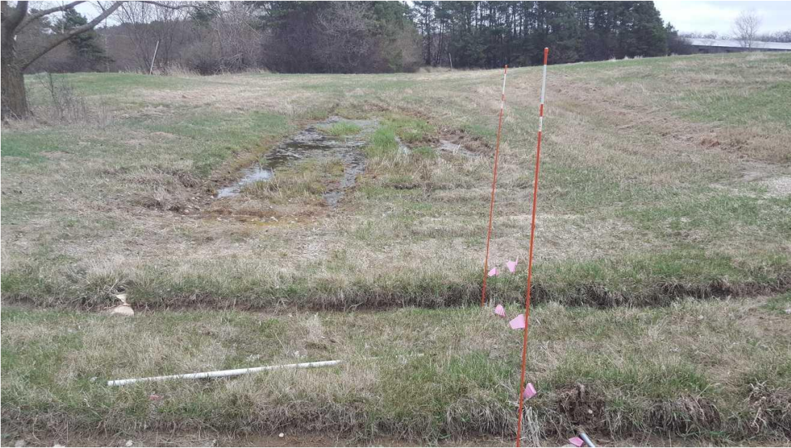
Settlement Area 1 – Located on the North Side near the pine trees looking East. Before filling in and regrading.
