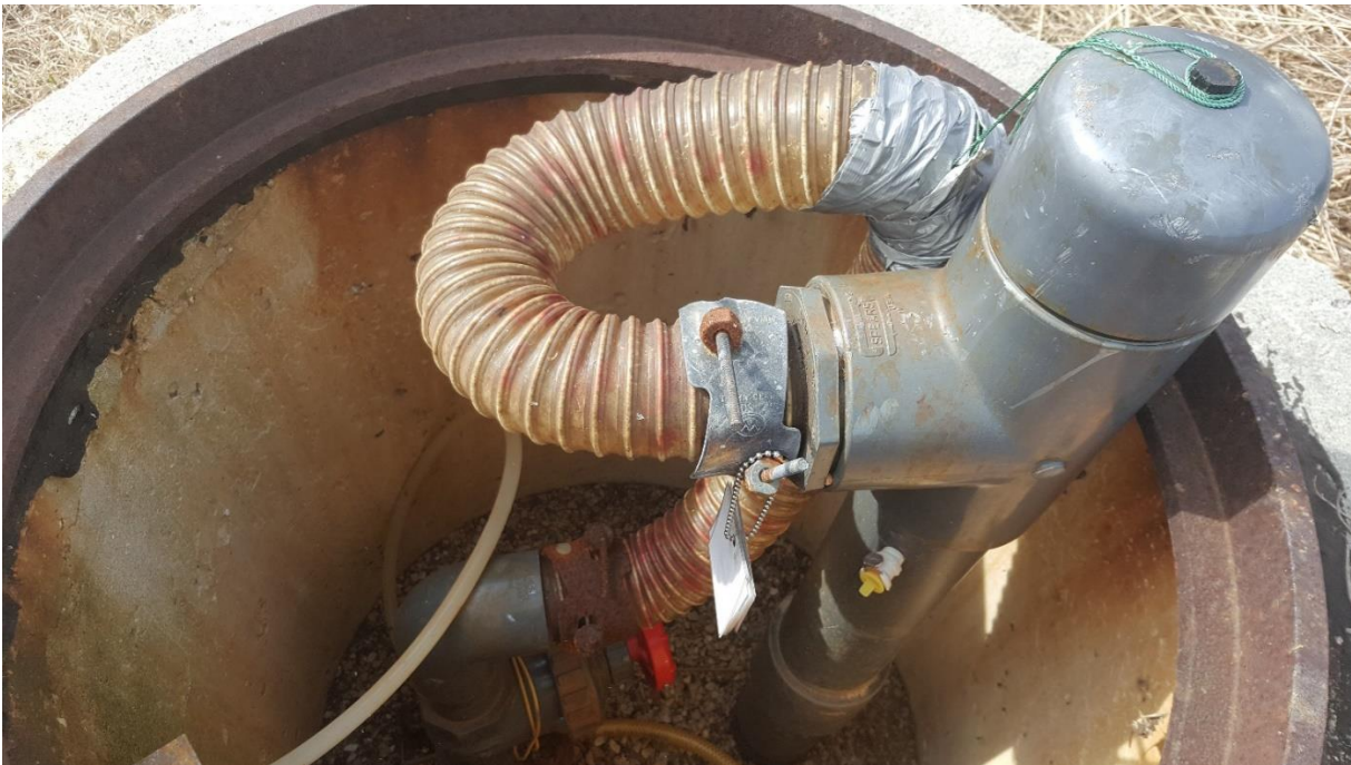
Broken Kanaflex hose. Repaired April 2018.
