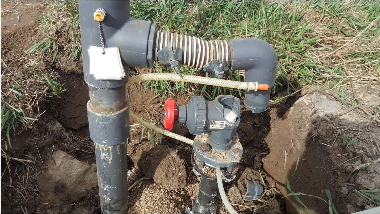
Broken valve at EW-6. Repaired May 2018.
