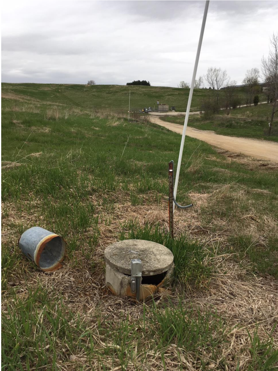
2,000 gallon UST near leachate load out area (May 2019)
