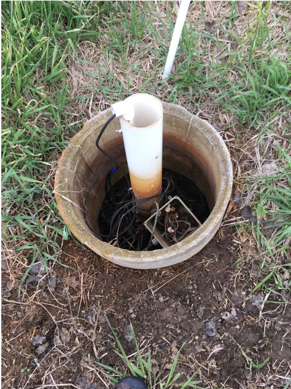
10,000 gallon UST leachate tank flat manhole
