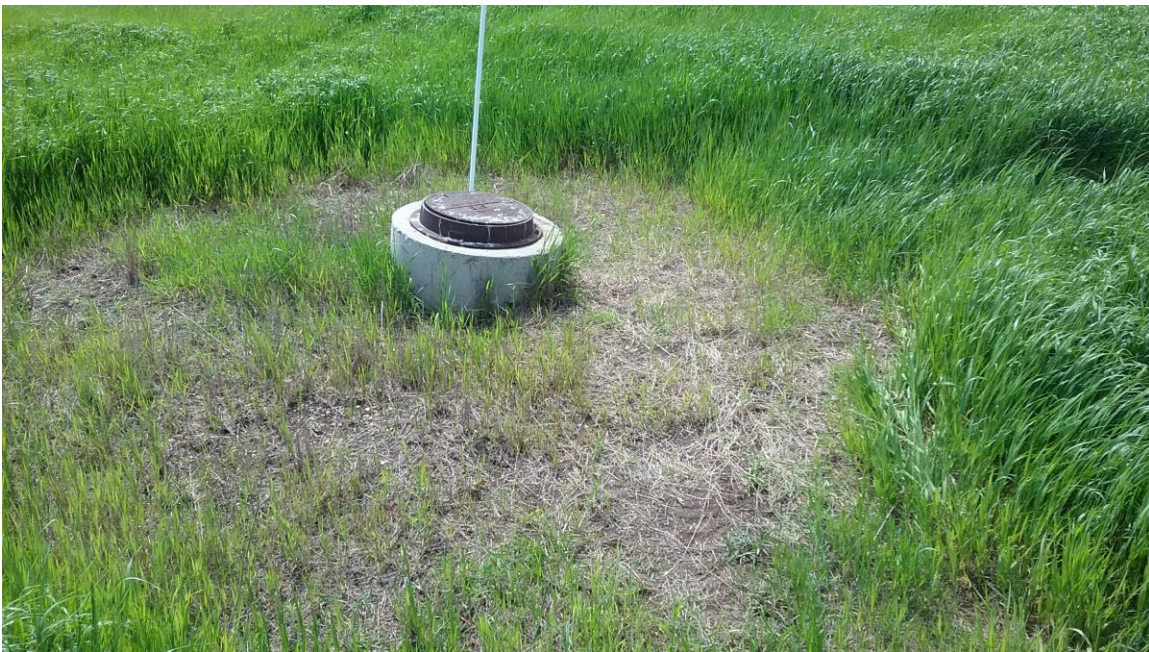
Photo #2: Gas Well G-1 – Stressed Vegetation Surrounding Gas Well
