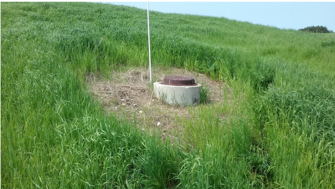
Photo #11: Gas Well G-8 - Stressed Vegetation Surrounding Gas Well.
