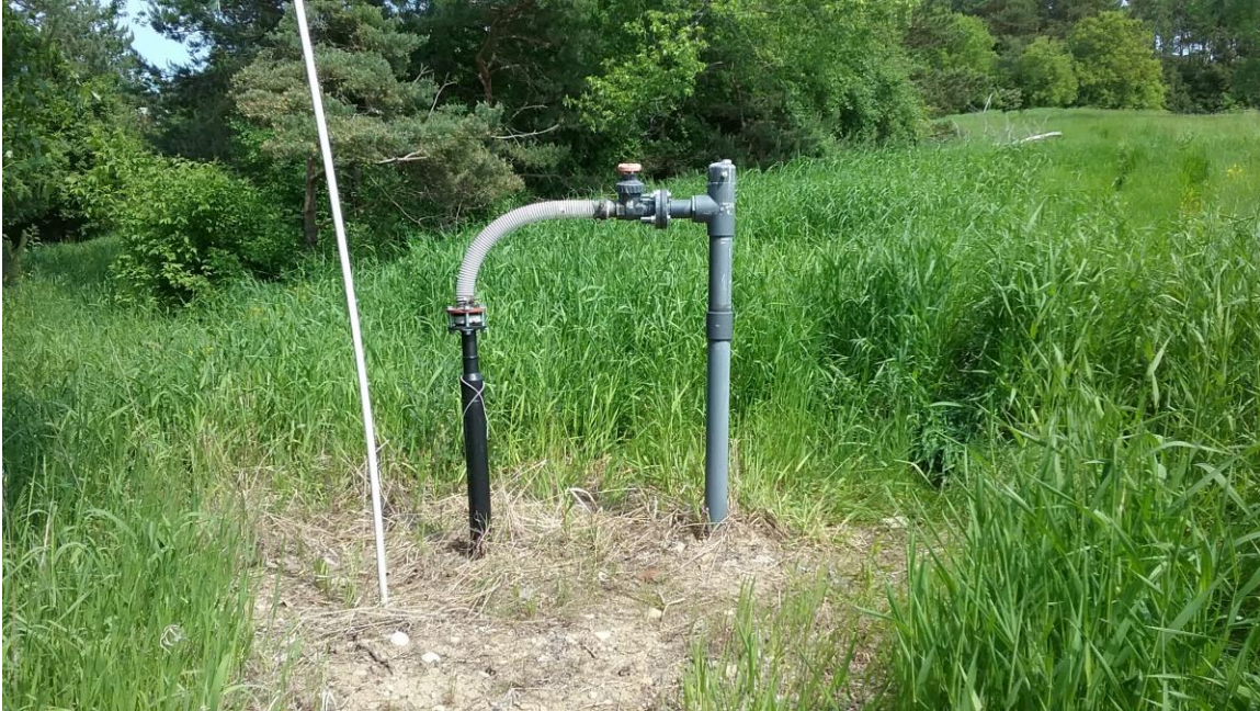
Photo #3: Gas Well EW-20 - Stressed Vegetation Surrounding Gas Well
