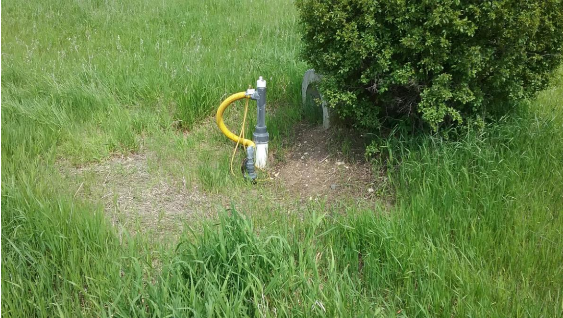
Photo #8: Gas Well G-4 - Stressed Vegetation Surrounding Gas Well.
