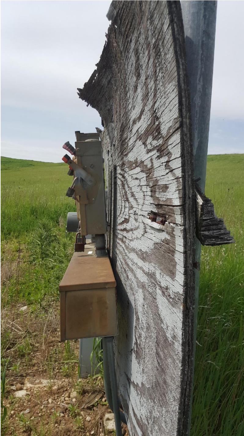
Photo #19: Main Electrical Panel Needs To Be Replaced
