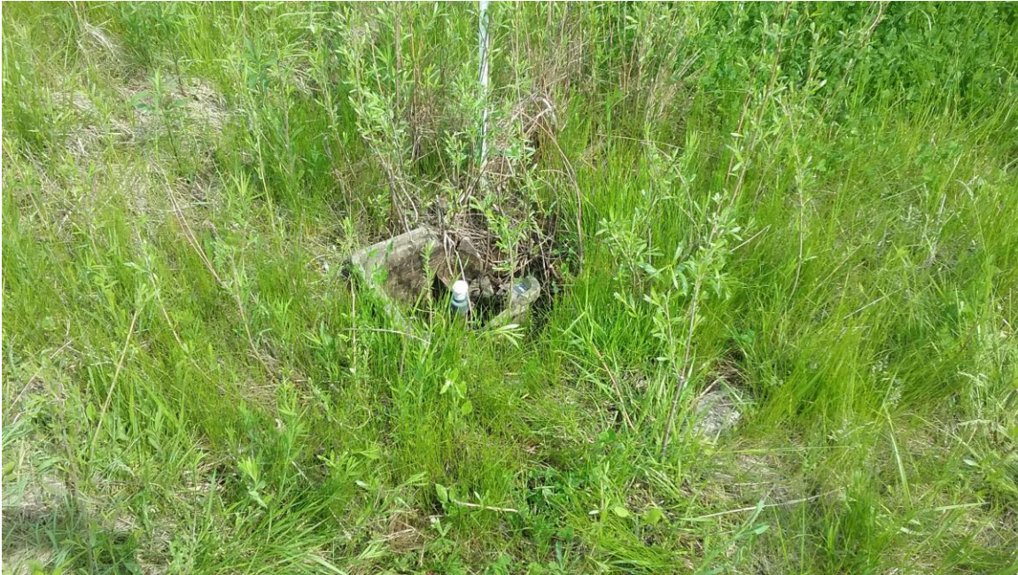
Photo #9: HMP-2 – Protective Casing Has Settled. HMP-2 Is Located In A Low Area.
