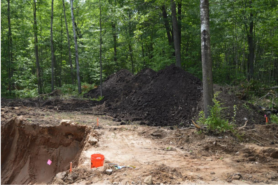
6/10/15: Temporary stockpiling of clean backfill over soil scrape areas on the northwest end of the site, looking west
