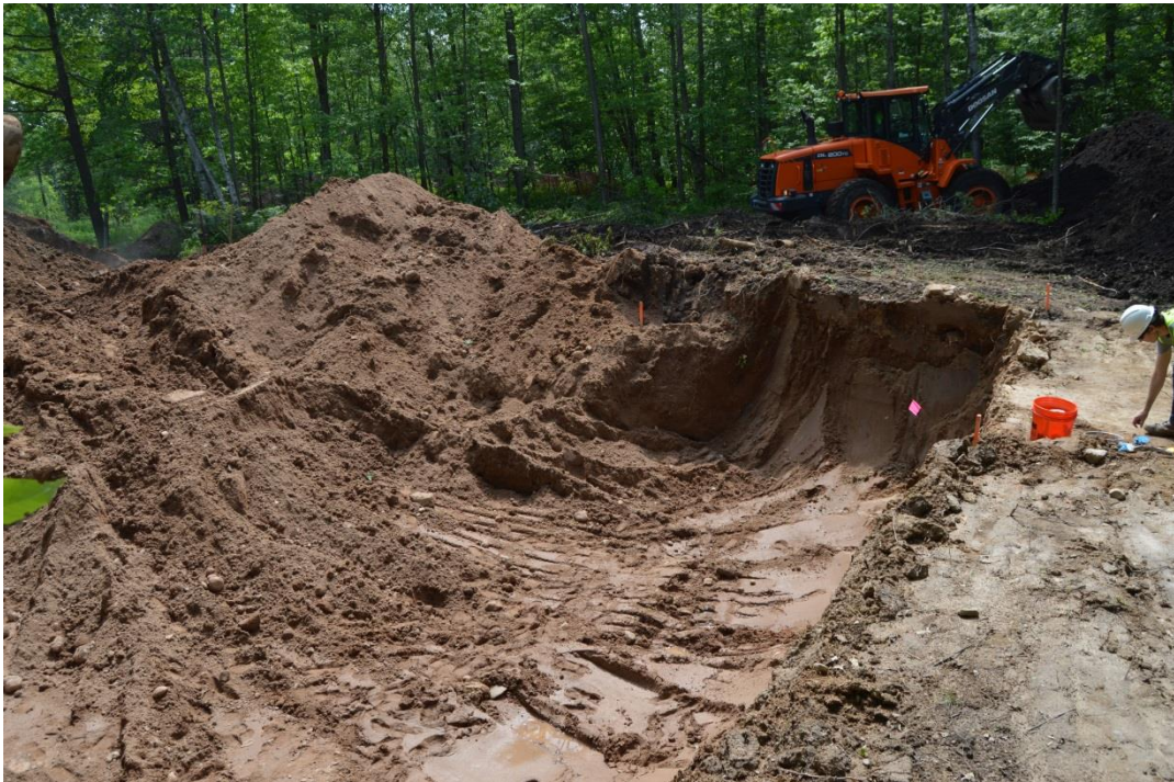
6/10/15: Beginning removal of former burial pit area on southwest corner of deep excavation
