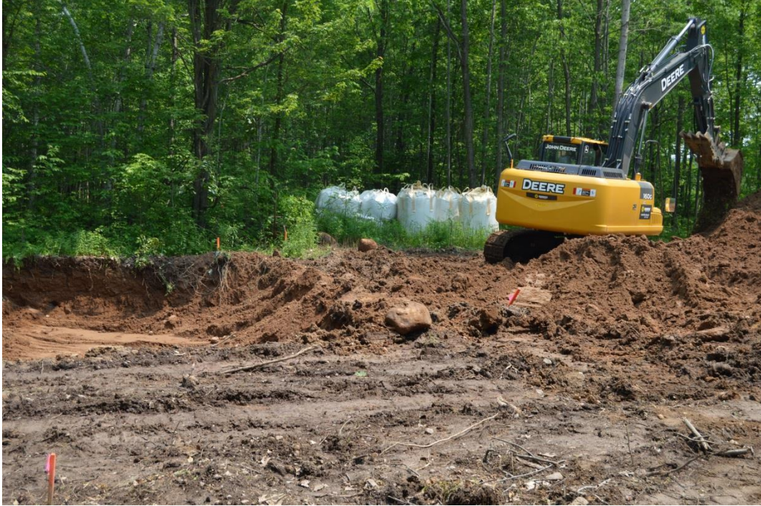
6/9/15: Temporary stockpiling of contaminated soil that has been mixed with Free Flow, looking east-southeast
