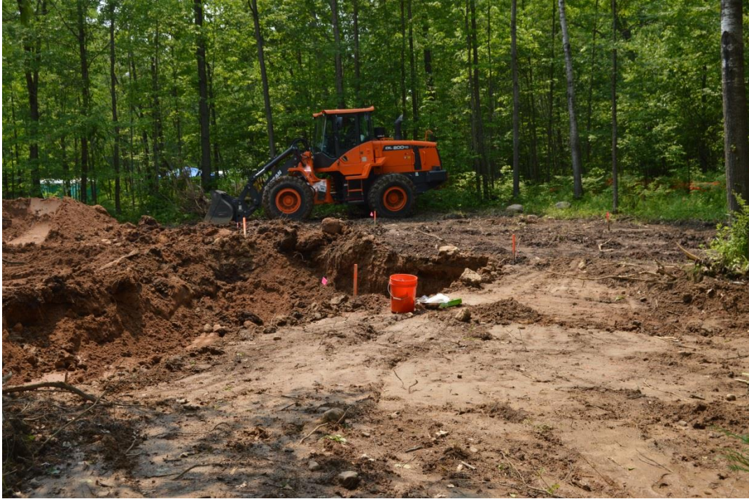
6/9/15: Shallow soil scrape areas north and west of deep excavation, looking west-southwest
