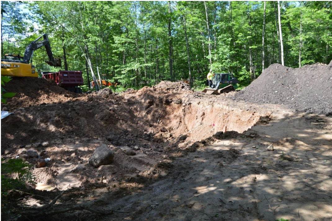
6/16/15: Deep excavation to approximately nine feet below ground surface, former burial pit area excavated to approximately ten feet below ground surface, looking southwest
