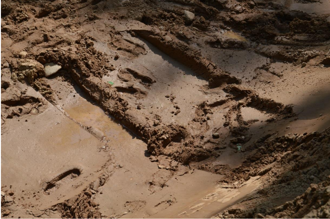
6/10/15: Bottom of deep excavation dug down to saturated zone at approximately nine feet below ground surface
