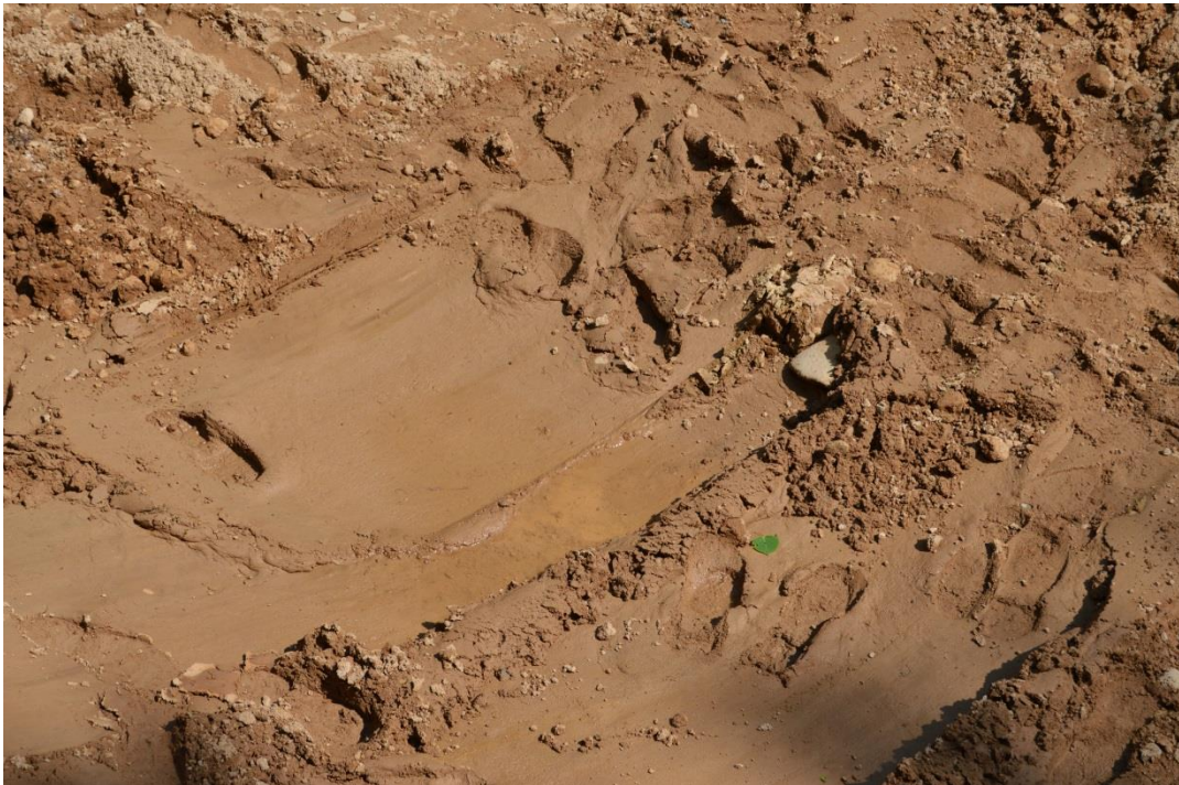
6/10/15: Bottom of deep excavation dug down to saturated zone at approximately nine feet below ground surface
