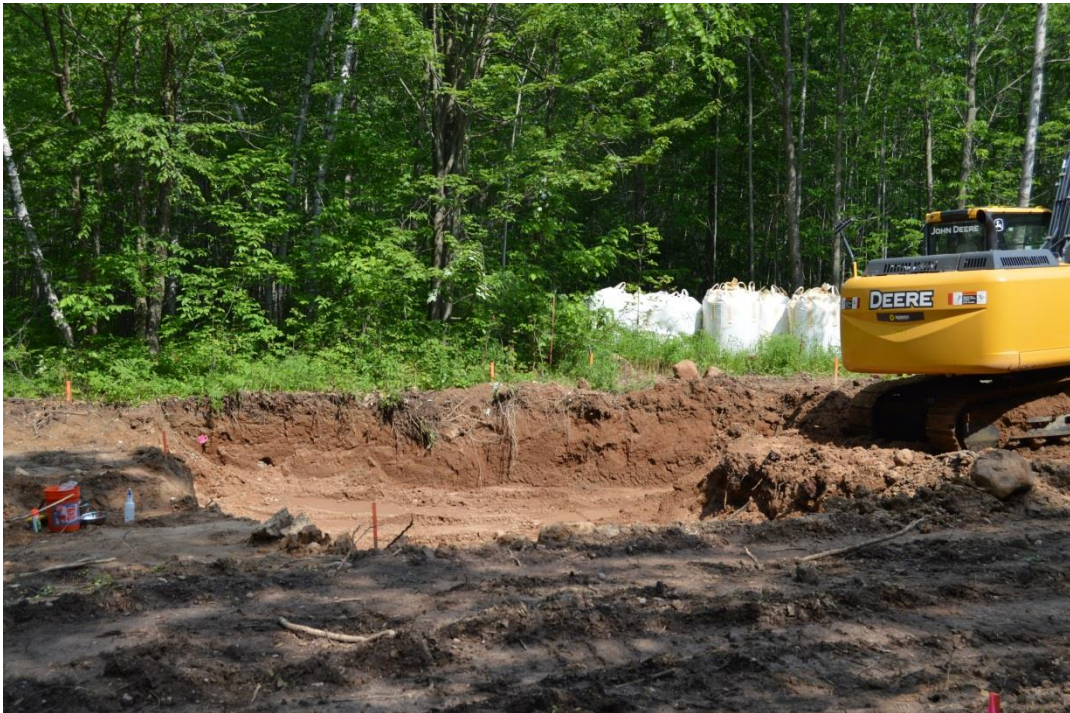
6/9/15: Former storage shed area continues to be excavated deeper due to high arsenic concentrations field screened in soil with an XRF, looking east-southeast
