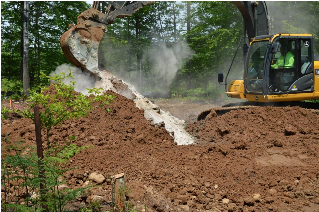
6/9/15: Contaminated soil being mixed with Free Flow prior to temporary stockpiling, looking north-northeast
