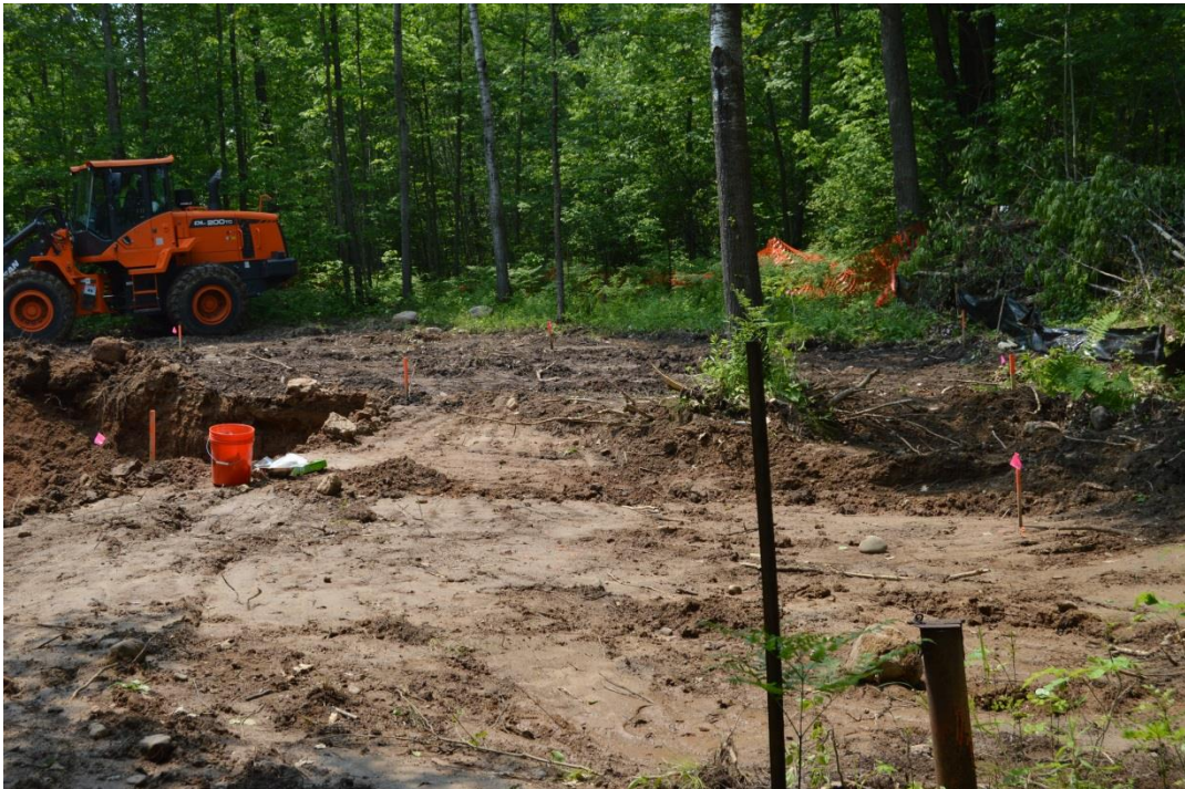
6/9/15: Silt fence between removal area and marsh and orange security fence bordering excavation area, monitoring well B-10 in foreground, looking west-southwest
