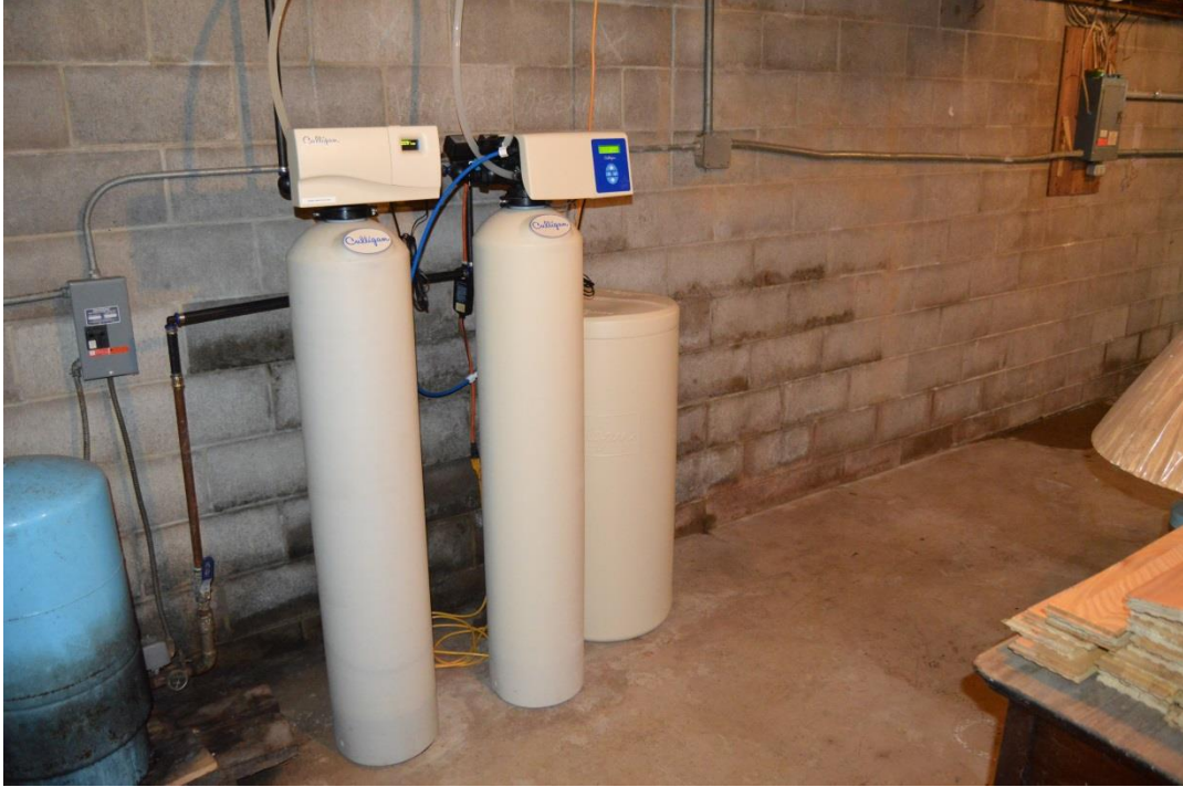
6/17/15: Water treatment system installed in adjacent Timm residence
